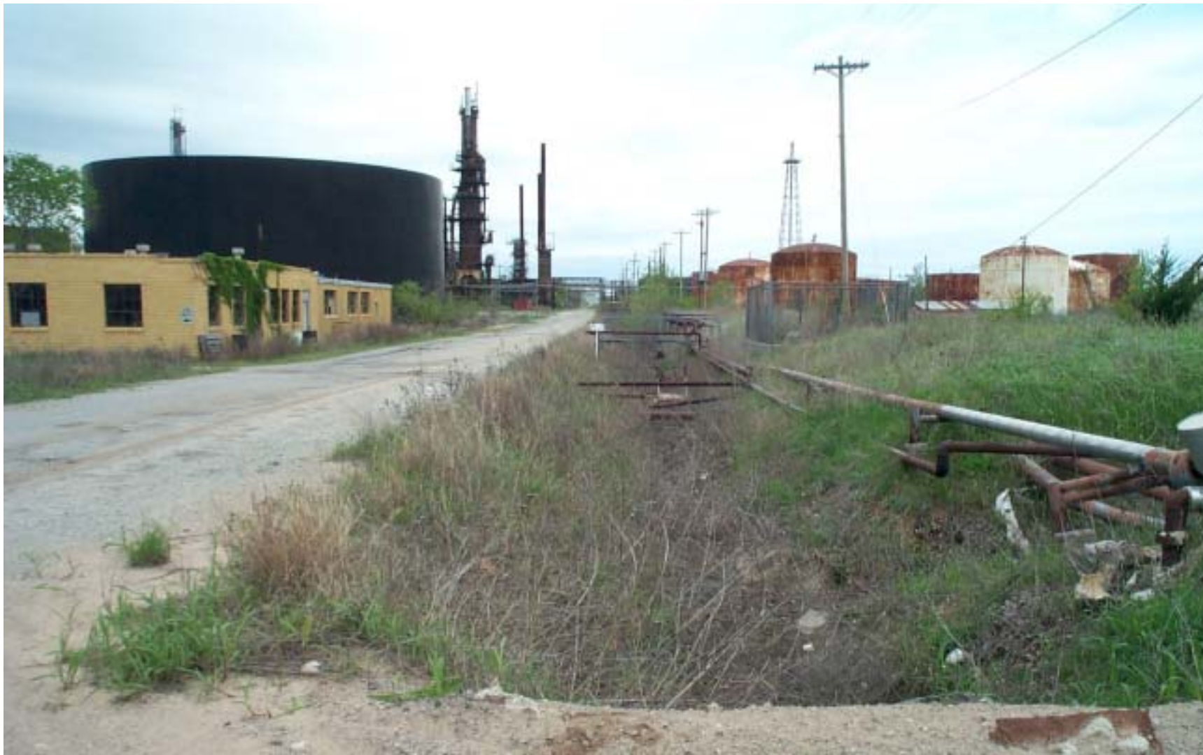
Photograph 40: Looking west along surface water runoff ditch on CPC property, clogged by vegetation and debris.
