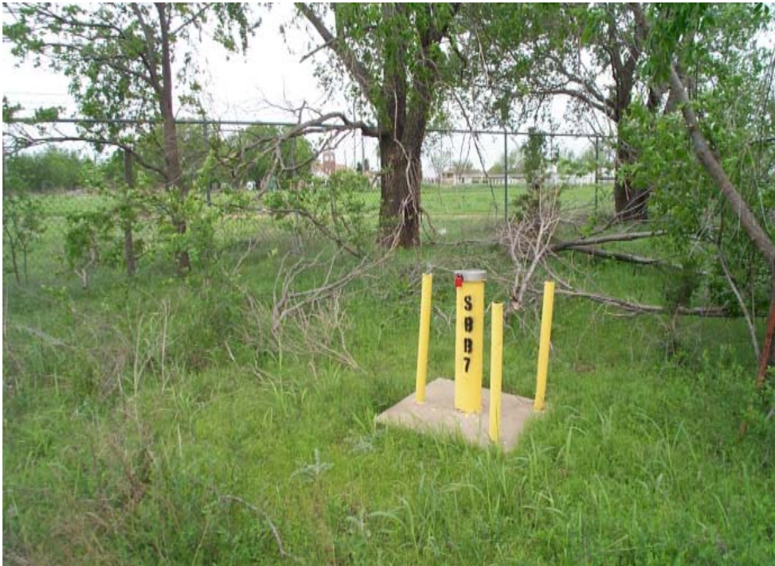
Photograph 6: Typical ground water monitoring well.
