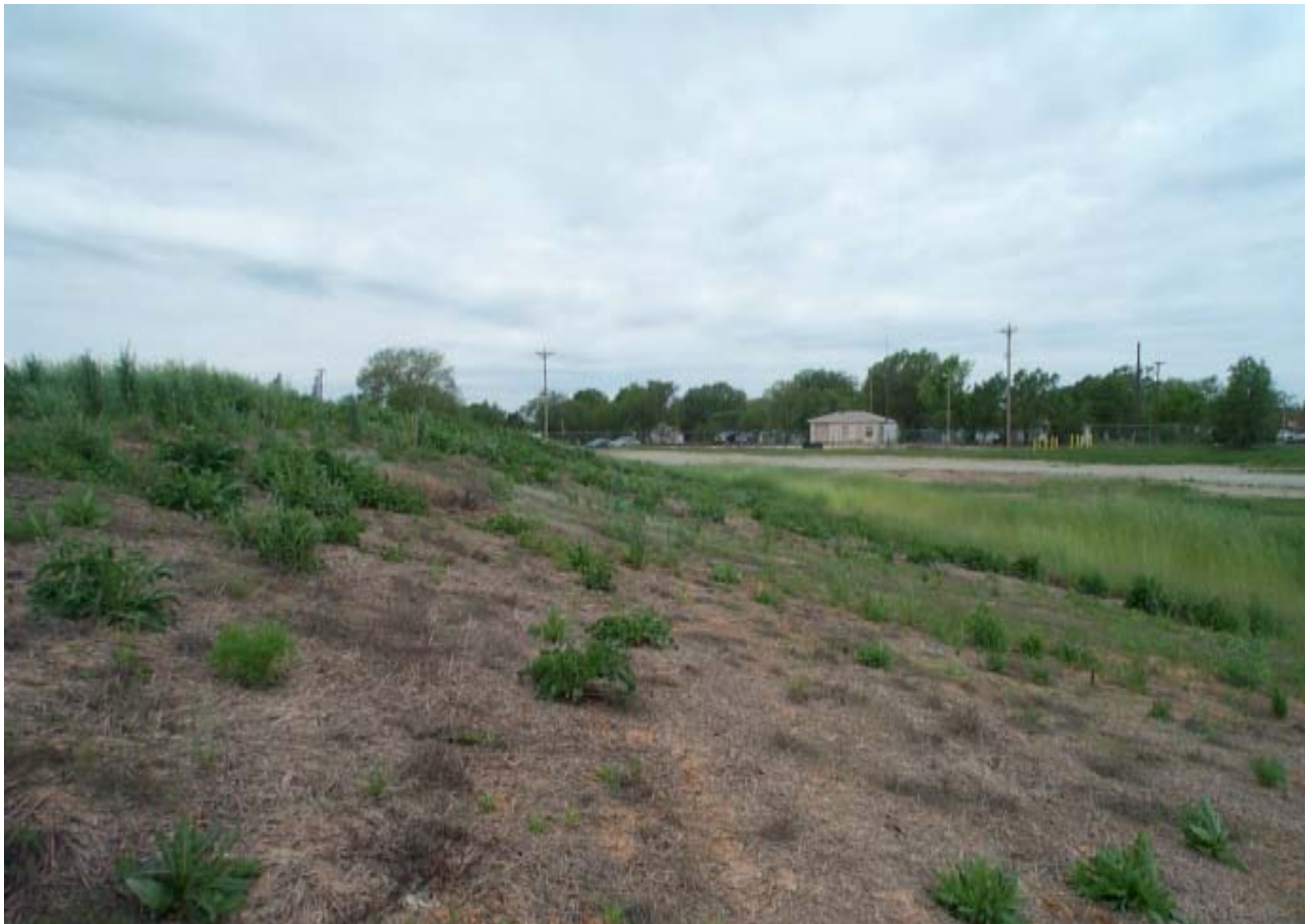
Photograph 1: Sparse vegetative cover visible on embankment of non-hazardous waste landfill.
