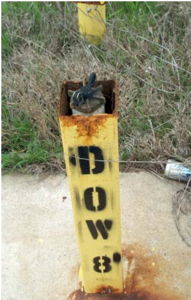
Photograph 42: Ground water monitoring well located north of Highway 277. Protective casing damaged by corrosion (possibly hydrogen sulfide).
