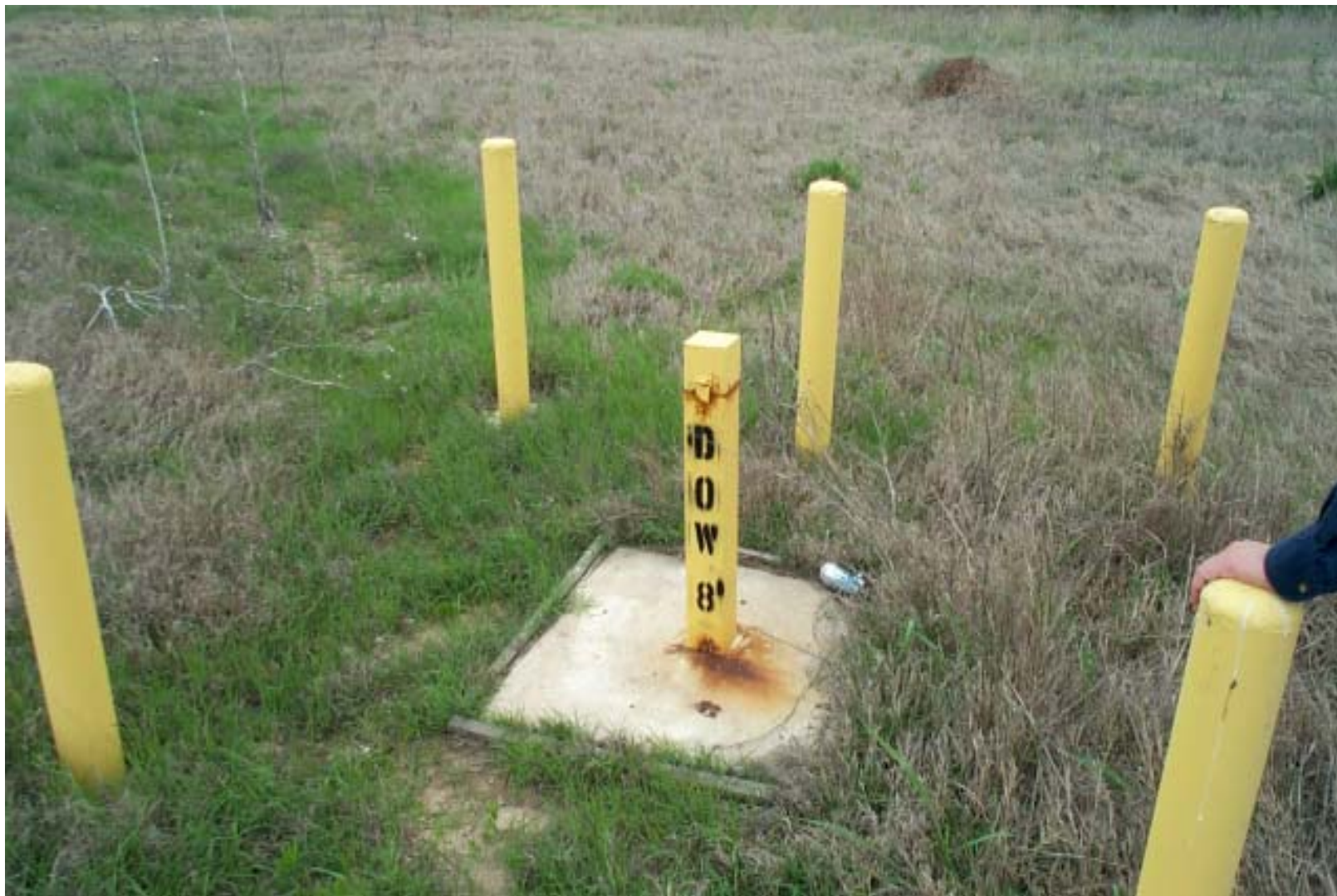
Photograph 43: Ground water monitoring well located north of Highway 277. Protective casing damaged by corrosion (possibly hydrogen sulfide).
