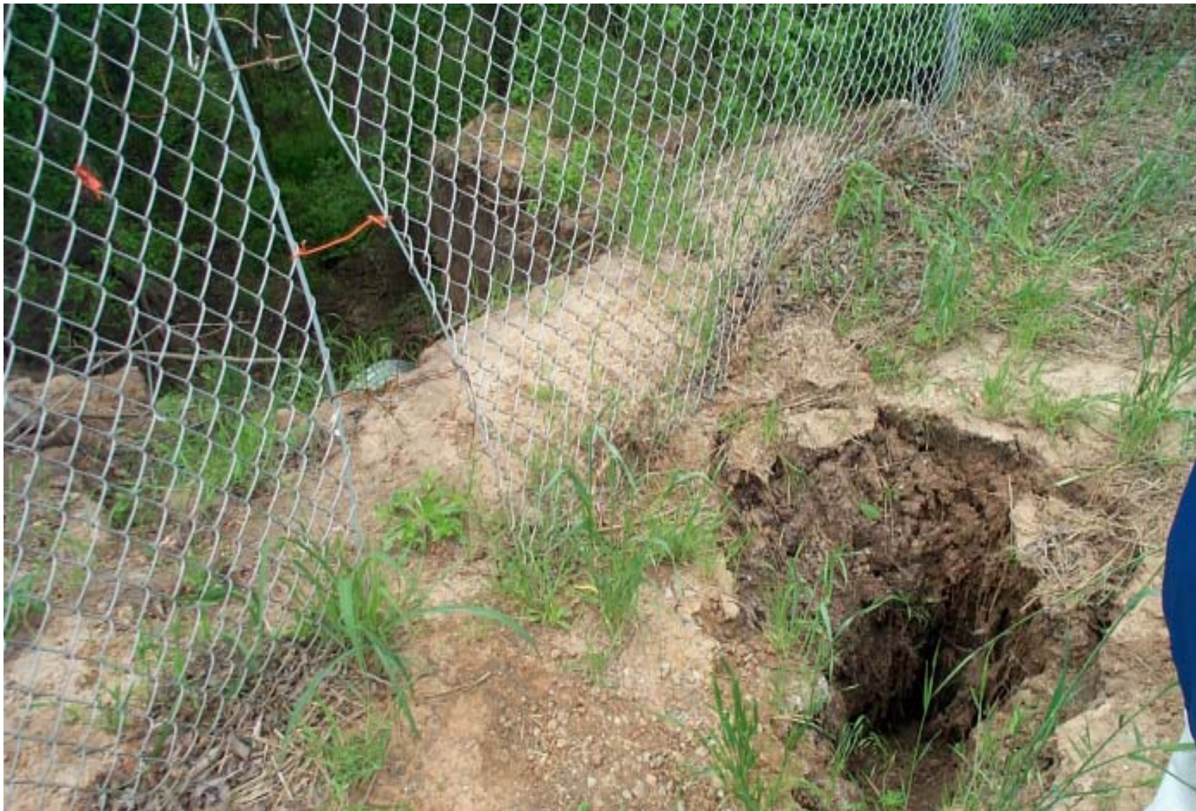
Photograph 15: Damaged fence along east perimeter and hole caused by erosion, approximately 250' south of monitoring well SBB-11.
