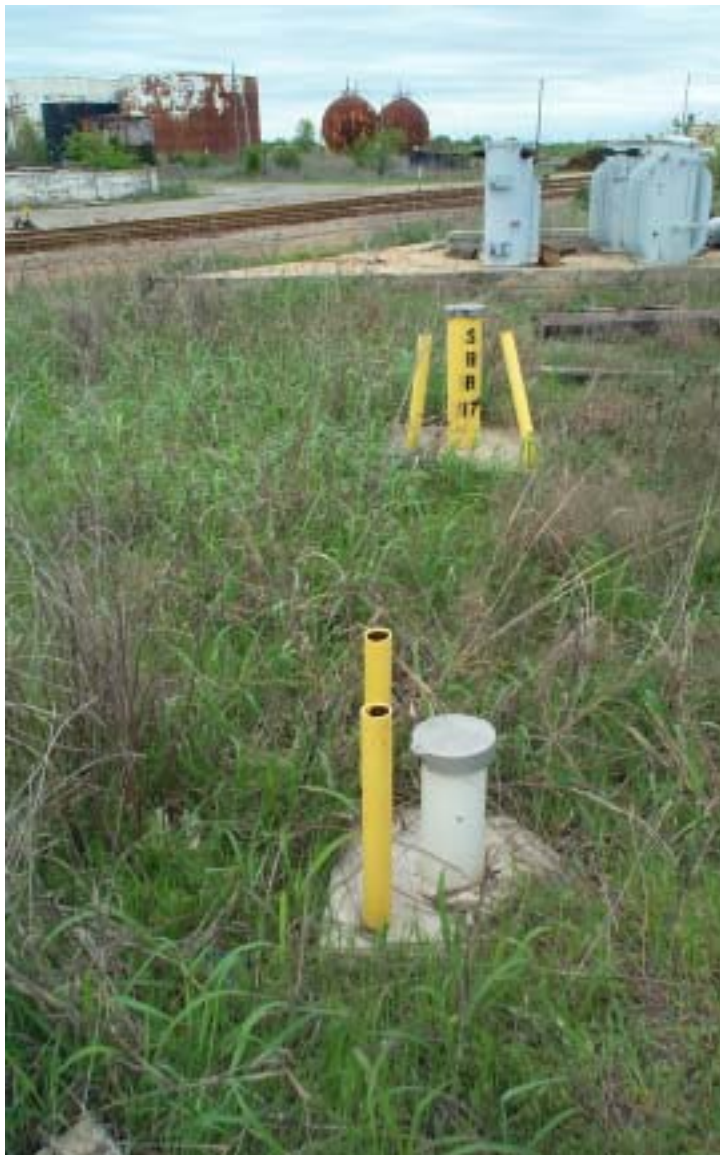
Photograph 39: Monitoring wells on CPC property. Damaged RCRA well in foreground.
