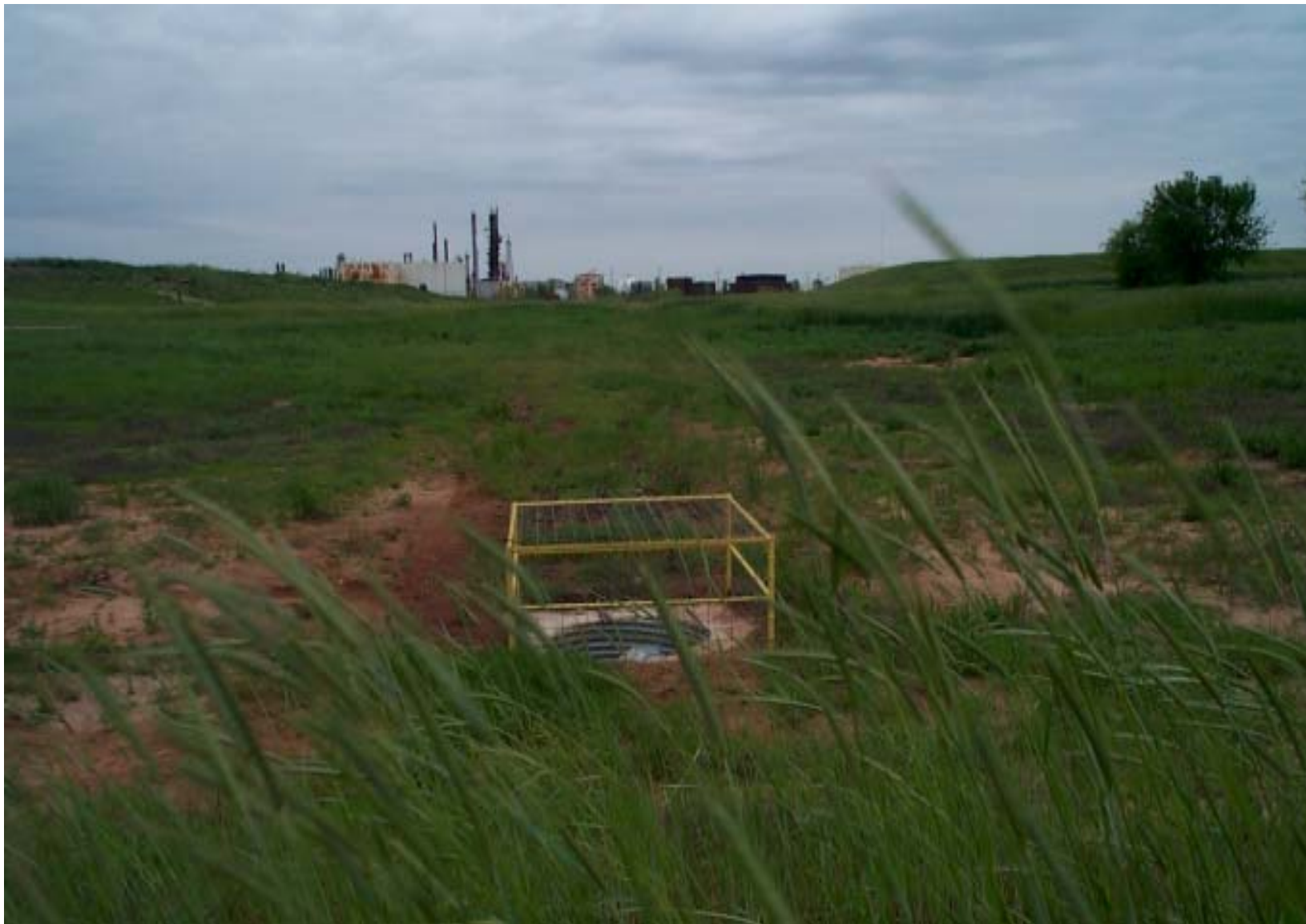
Photograph 7: Storm water outfall No. 003 for off-site discharge.
