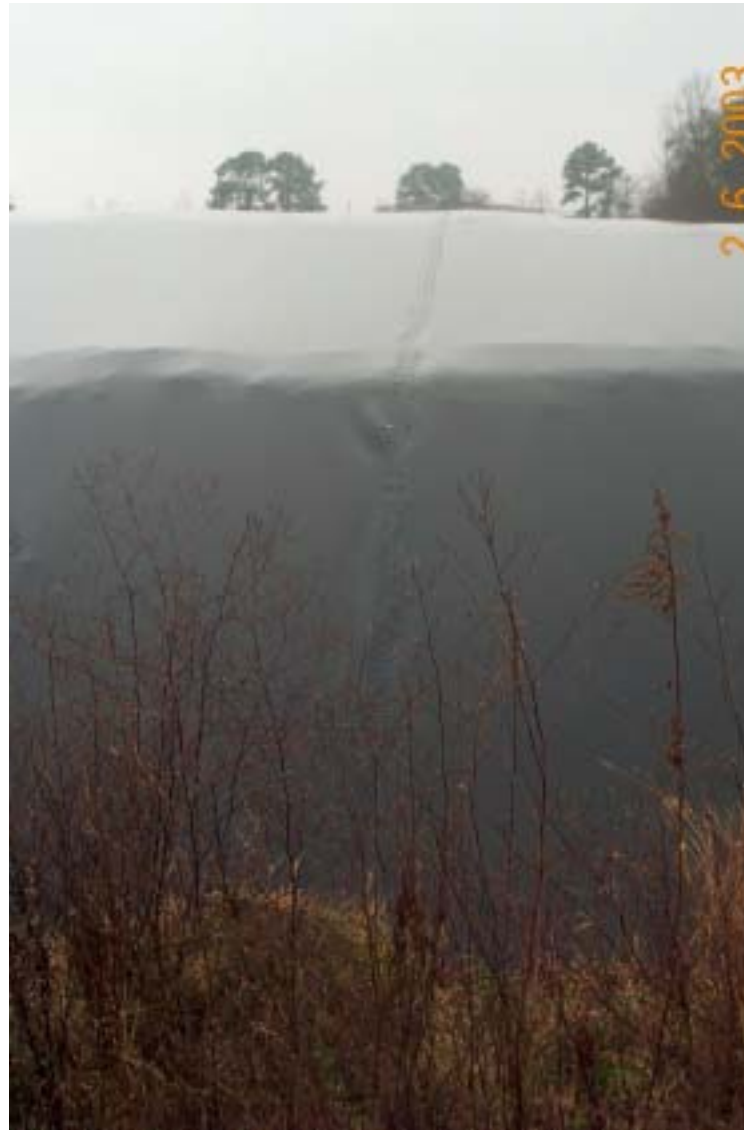
Looking west, across the biopile cover, at a seam in the cover.
