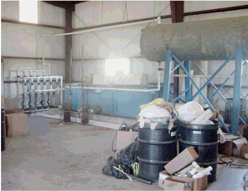
Photo 1: Oil-Water separator within wastewater treatment plant (WWTP)
