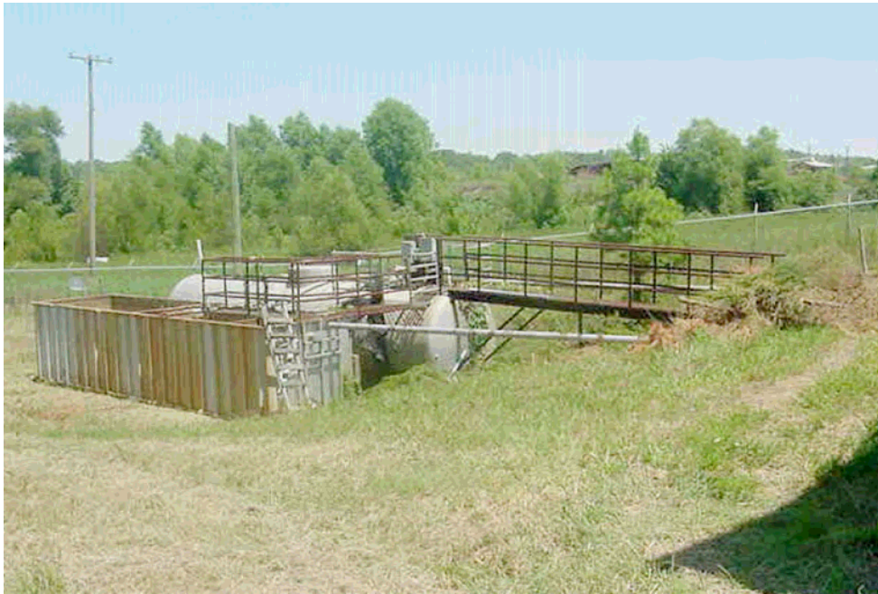
Photo 2: Storage and Overflow tanks north of (WWTP)
