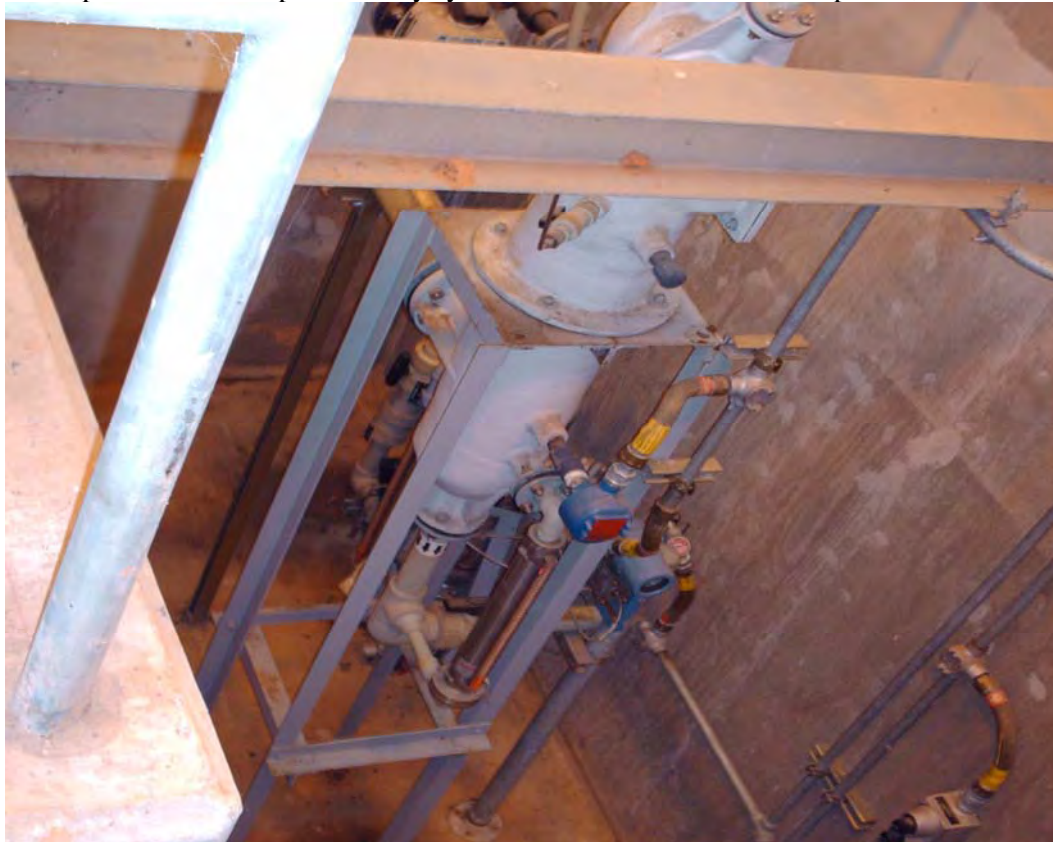
Photograph No. 8 Description: PMRS vapor recovery system
