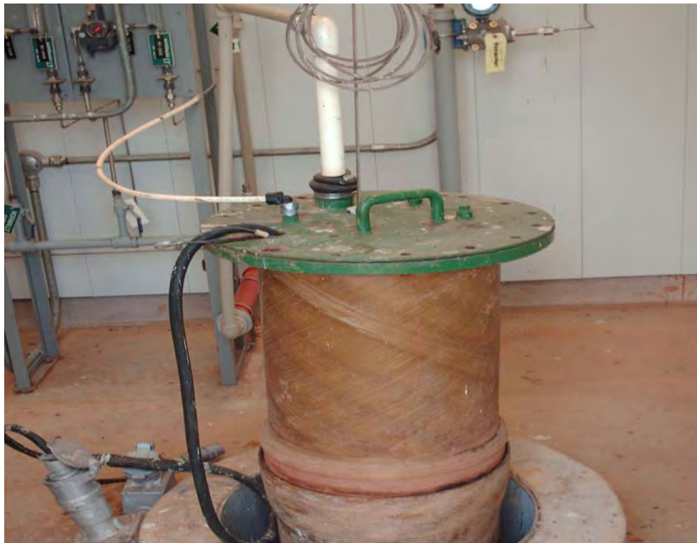
Photograph No. 3 Description: V-Trench recovery well (TRS-10)
