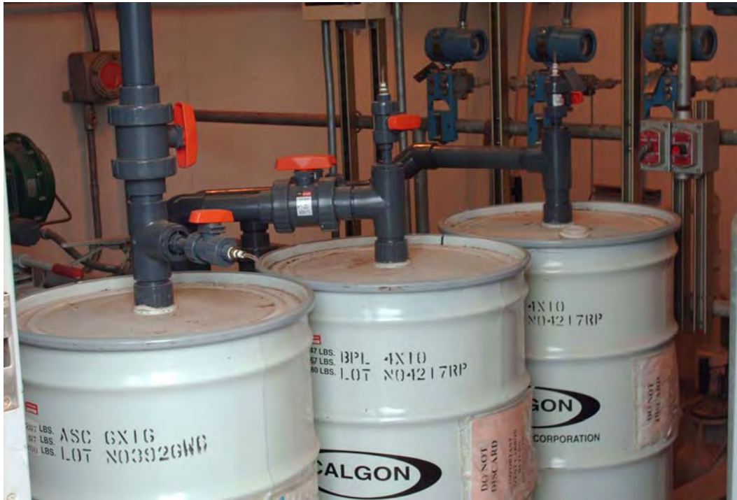
Photograph No. 7 Description: PMRS vapor recovery system
