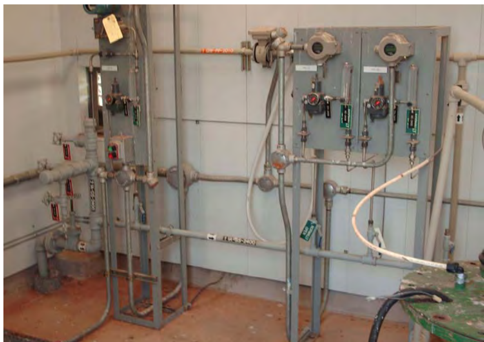
Photograph No. 4 Description: Control instruments within TRS-10 housing unit
