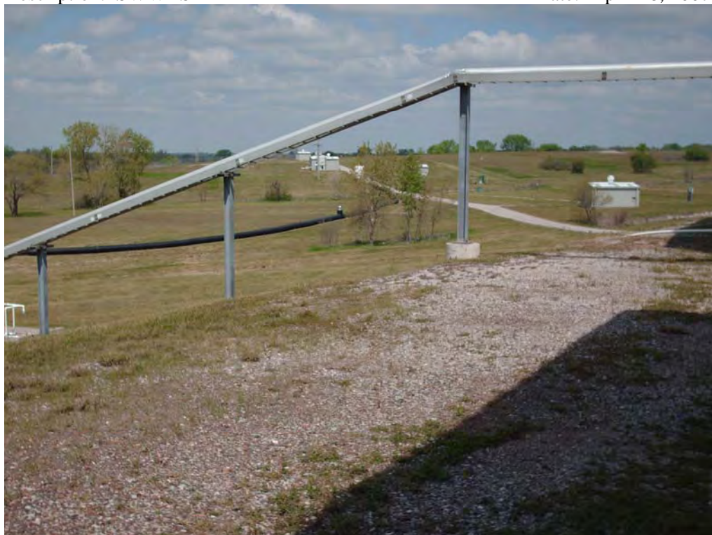
Photograph No. 20 Description: V-Trench Passive Aeration Pilot System
