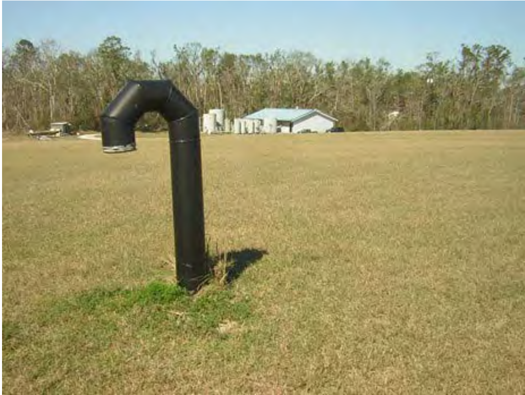
Photo 43: Landfill vent pipe on top of landfill cover. Ground water treatment plant visible in background. Taken 2/16/2006
