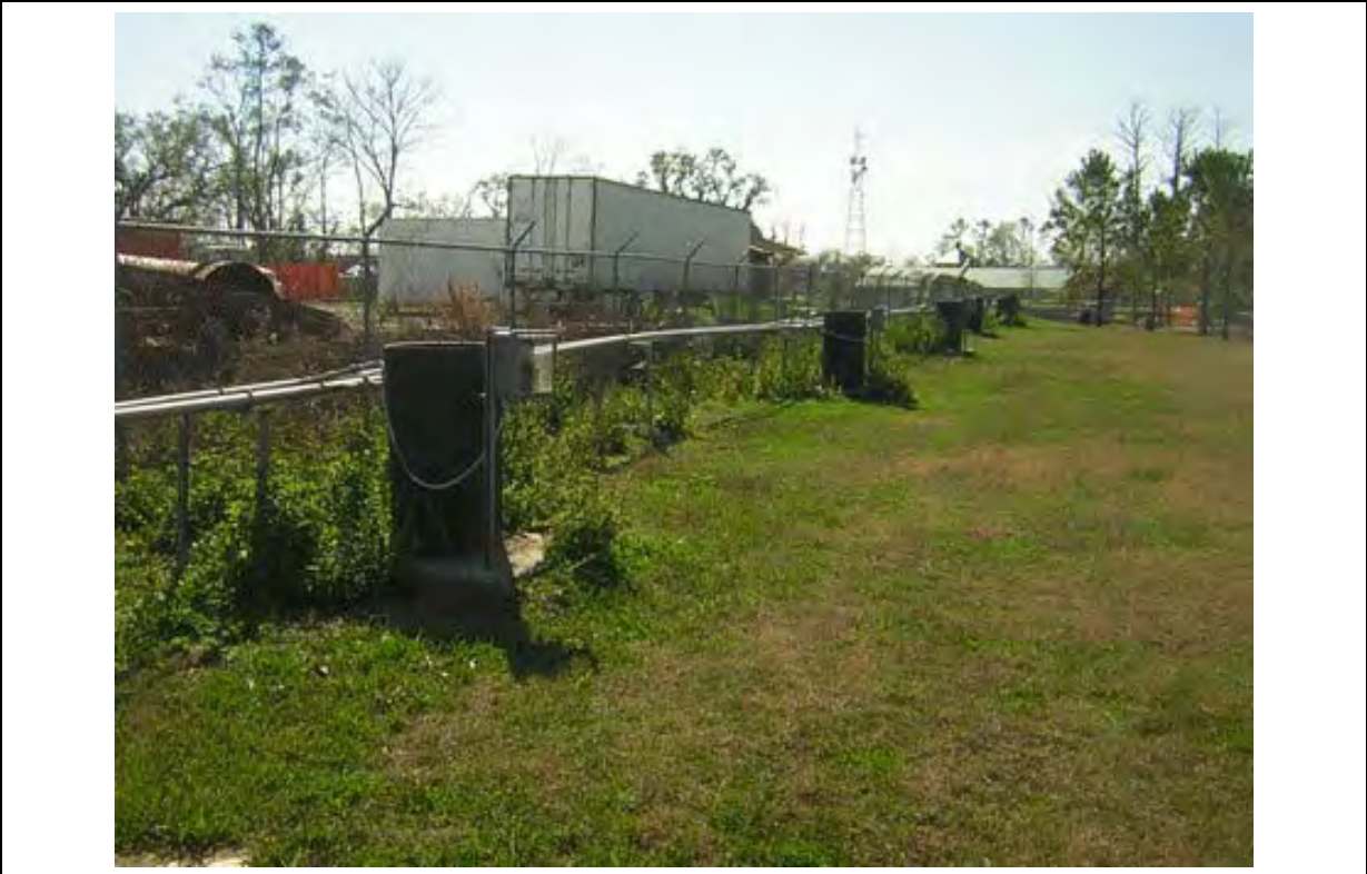
Photo 41: Looking south along piping and well vaults for northeast side of recovery array 2. Taken 2/16/2006
