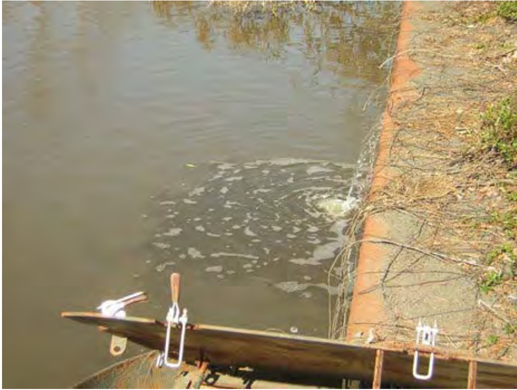
Photo 23: Treated discharge into bayou from ground water treatment plant. Taken 2/16/2006
