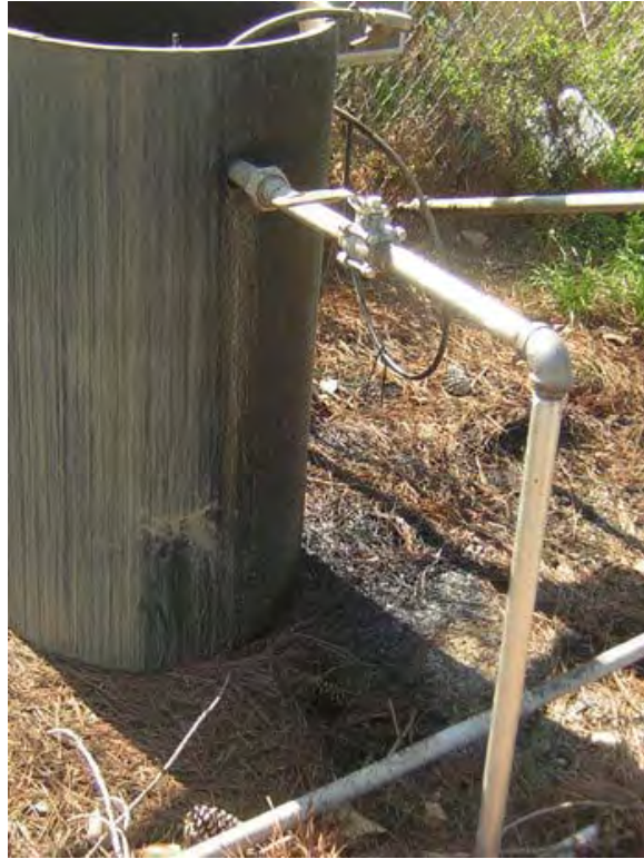
Photo 35: Close up of piping and well vault for recovery array 2. Taken 2/16/2006
