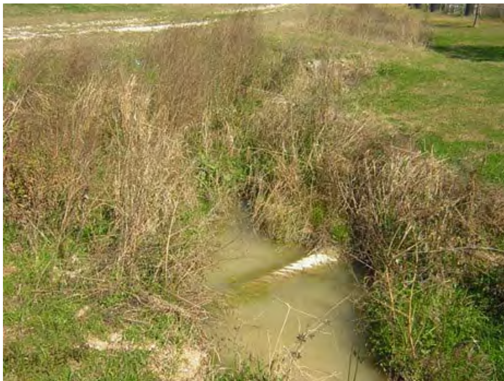
Photo 40: Looking north along surface drainage ditch on southeast side of landfill. Taken 2/16/2006
