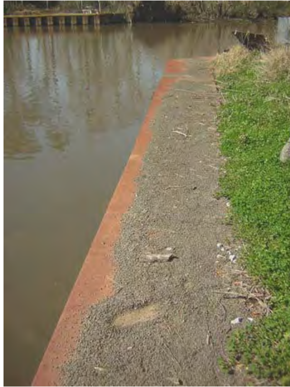
Photo 29: Dried sediment on top of sheet pile wall along bayou left behind by floodwaters associated with Hurricanes Katrina/Rita. Taken 2/16/2006
