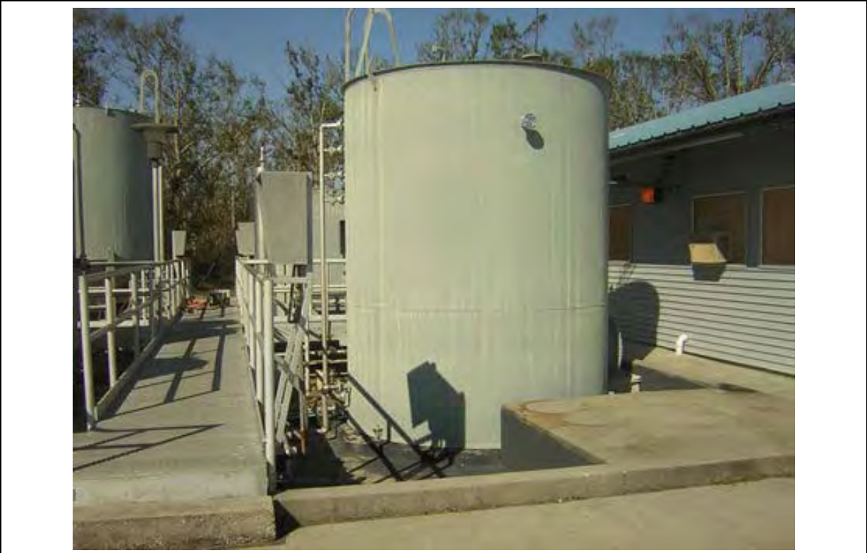
Photo 3: Bayou Bonfouca ground water treatment plant. Taken 2/16/2006.
