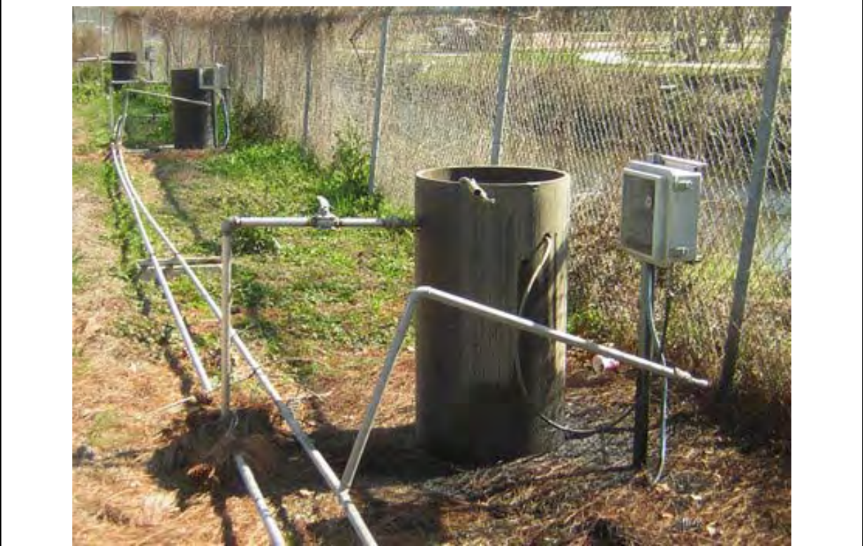
Photo 34: Close up of piping and well vault for recovery array 2. Taken 2/16/2006
