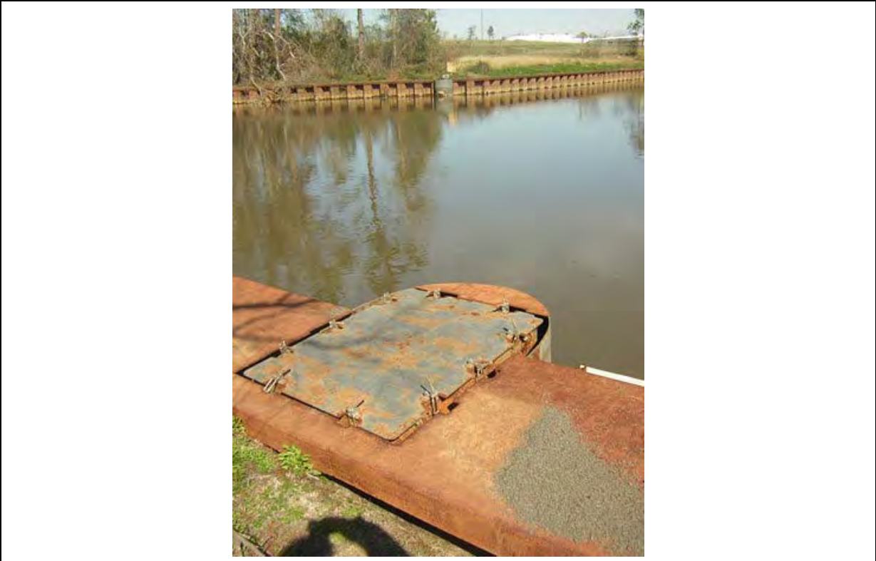
Photo 52: Vault for pipeline at bayou crossing from recovery array 3 to main part of site. Taken 2/16/2006
