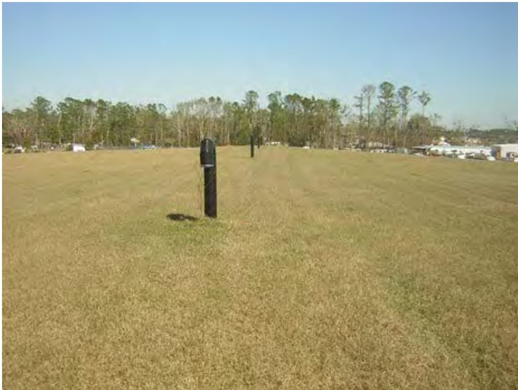
Photo 44: Looking north along line of vent pipes on top of landfill cover. Note small tree growing adjacent to vent pipe in foreground. Taken 2/16/2006
