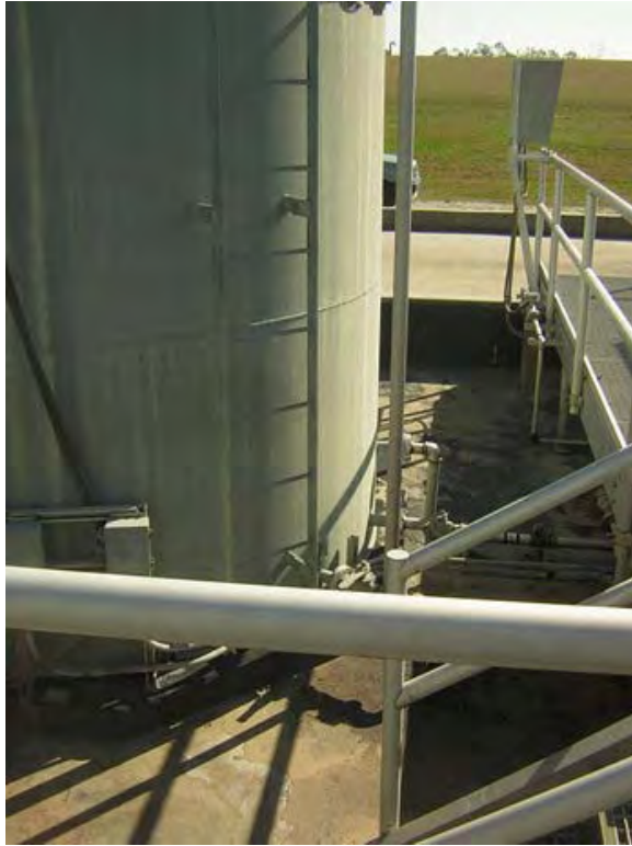
Photo 5: Bayou Bonfouca ground water treatment plant. Taken 2/16/2006.
