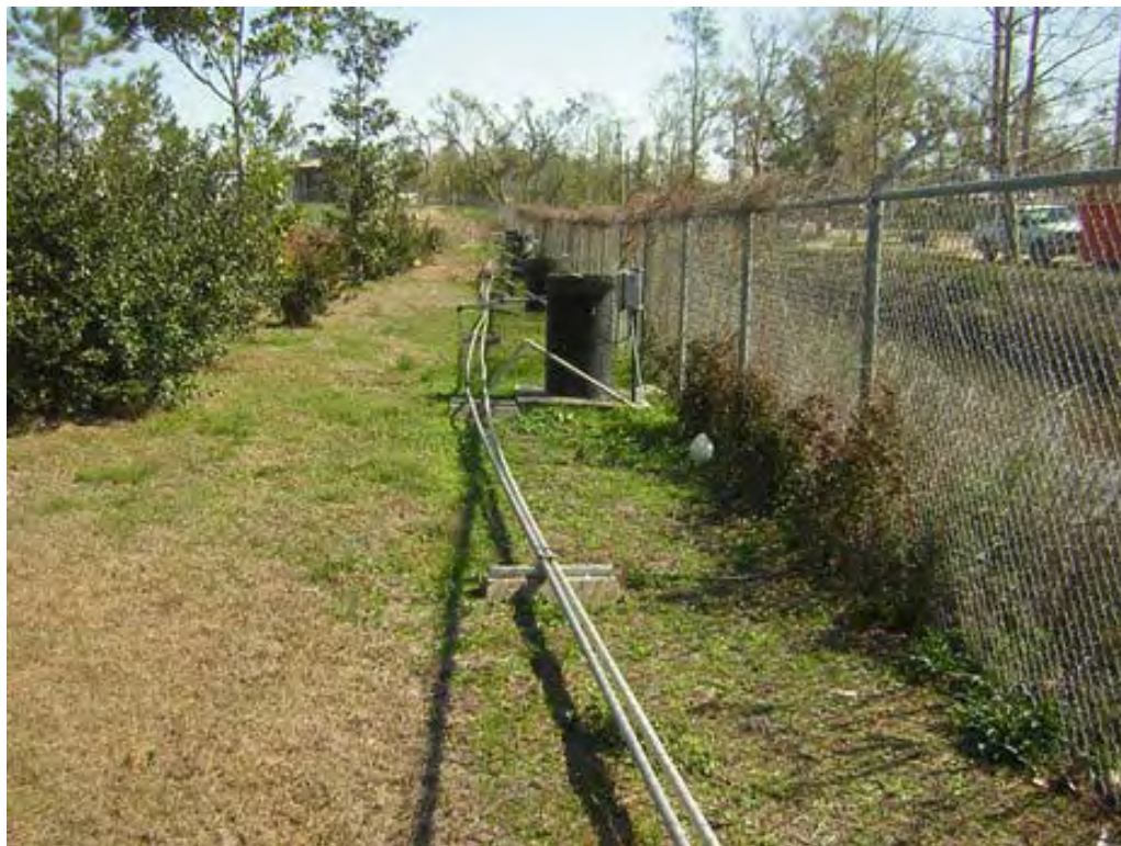
Photo 32: Looking east along piping and well vaults for recovery array 2. Taken 2/16/2006
