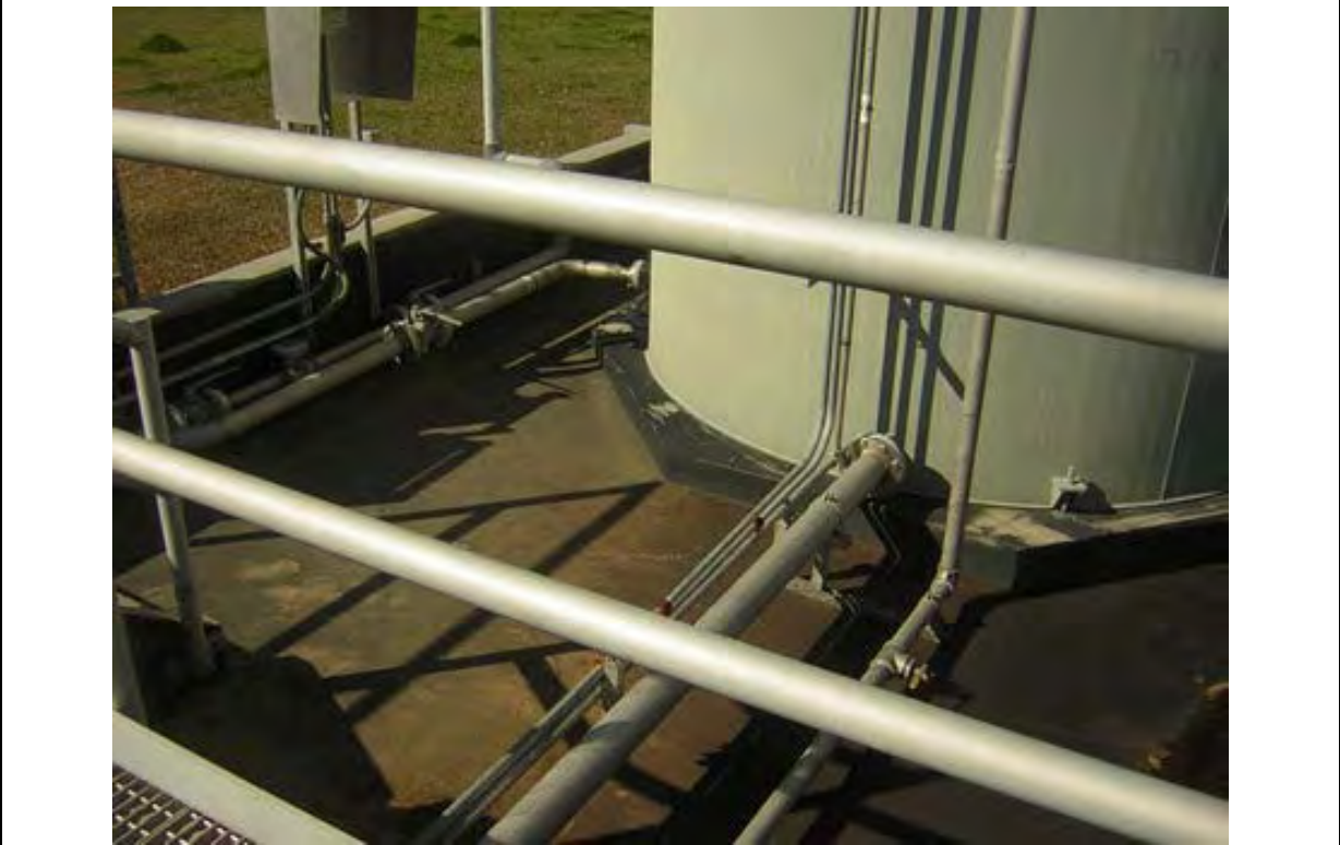
Photo 8: Ground water treatment system piping. Taken 2/16/2006
