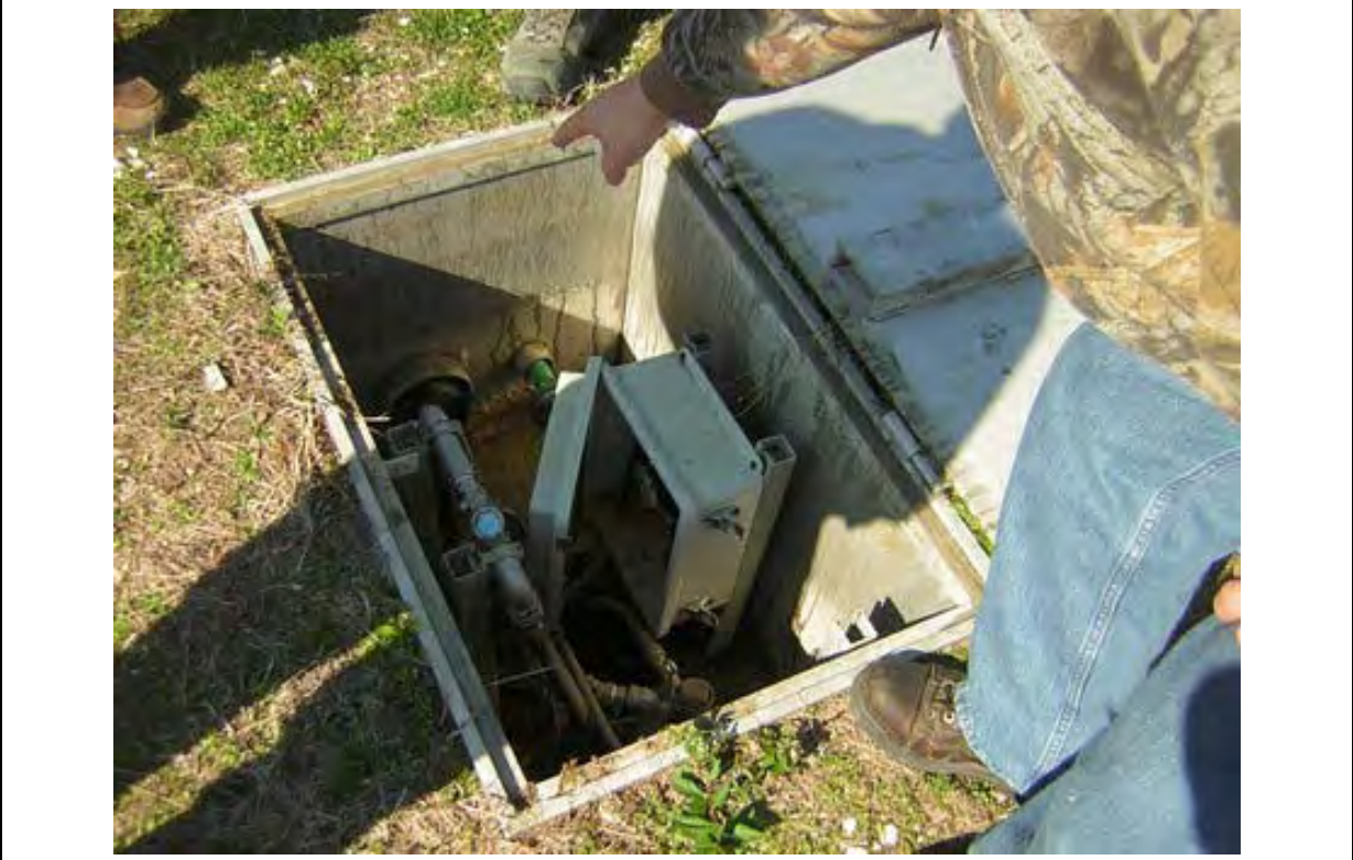
Photo 16: . Inside recovery array 1A well vault. Taken 2/16/2006
