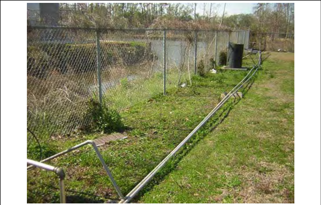
Photo 33: Looking west along piping and well vaults for recovery array 2. Taken 2/16/2006
