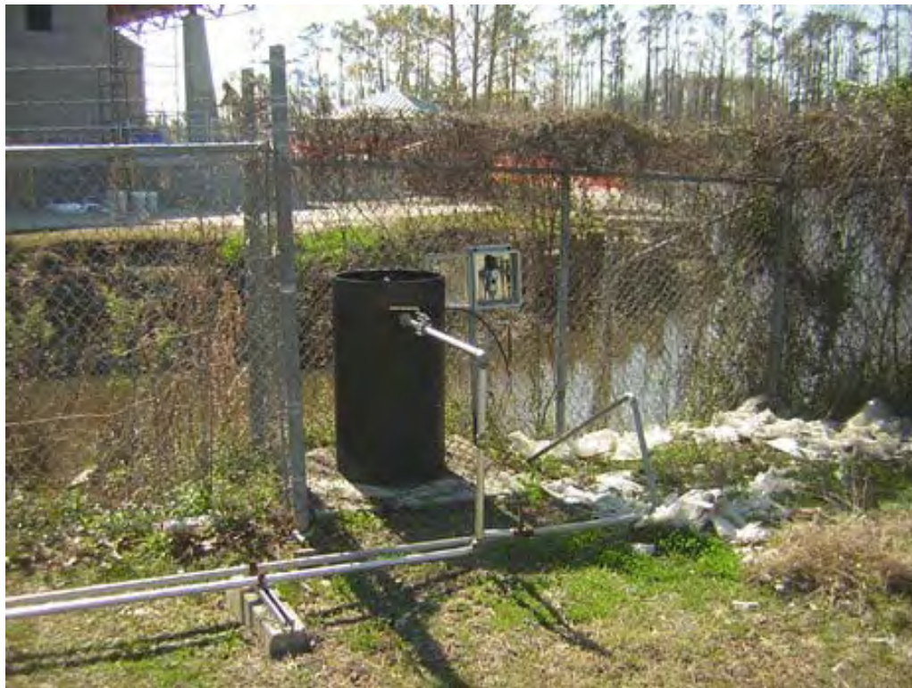
Photo 31: Well at west end of recovery array 2. City park in background. Taken 2/16/2006
