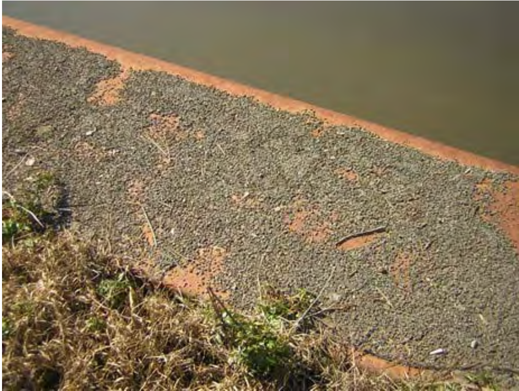
Photo 21: Dried sediment on top of sheet pile wall along bayou left behind by floodwaters associated with Hurricanes Katrina/Rita. Taken 2/16/2006
