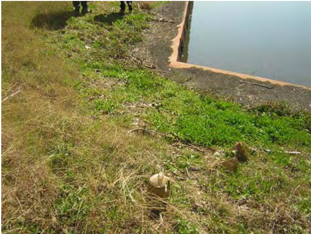
Photo 30: Dried sediment on top of sheet pile wall along bayou and debris left behind by floodwaters associated with Hurricanes Katrina/Rita. Taken 2/16/2006
