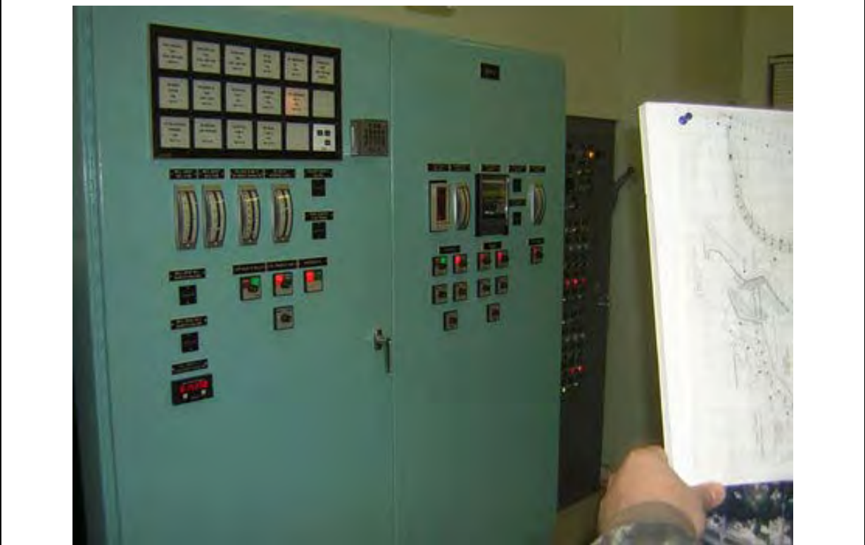
Photo 4: Control panel -- Inside ground water treatment plant control building. Taken 2/16/2006.
