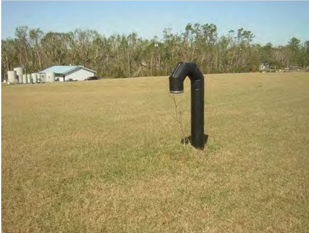
Photo 45: Vent pipe on top of landfill cover. Note small tree growing adjacent to vent pipe. Taken 2/16/2006
