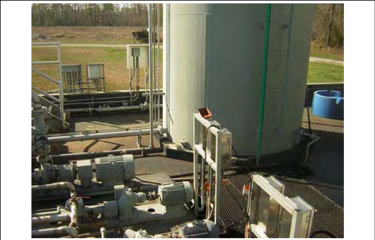
Photo 7: Bottom left, pumps within ground water treatment system, submerged and damaged during Hurricane Katrina. Taken 2/16/2006.
