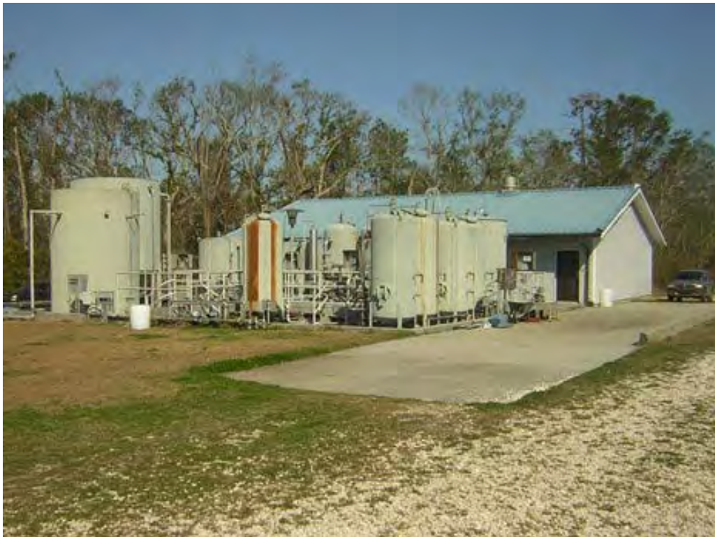
Photo 10: Overview of ground water treatment plant. Taken 2/16/2006
