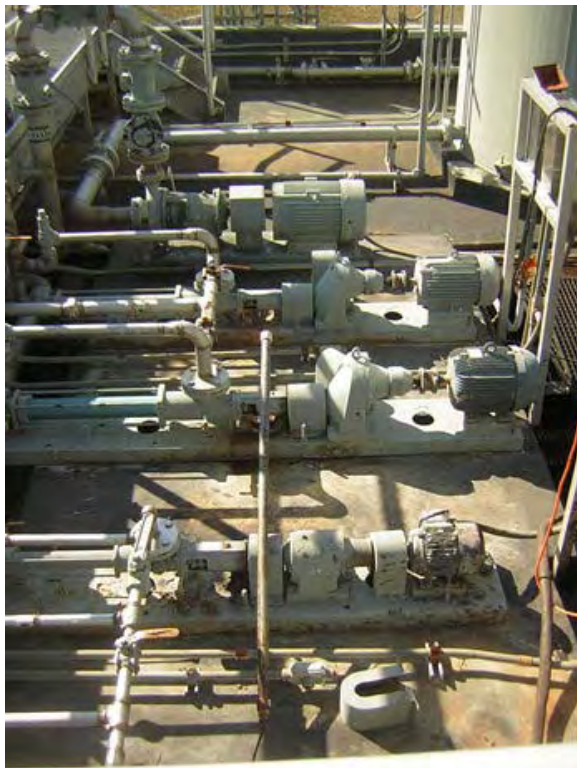
Photo 6: Pumps within ground water treatment system, submerged and damaged during Hurricane Katrina. Taken 2/16/2006.
