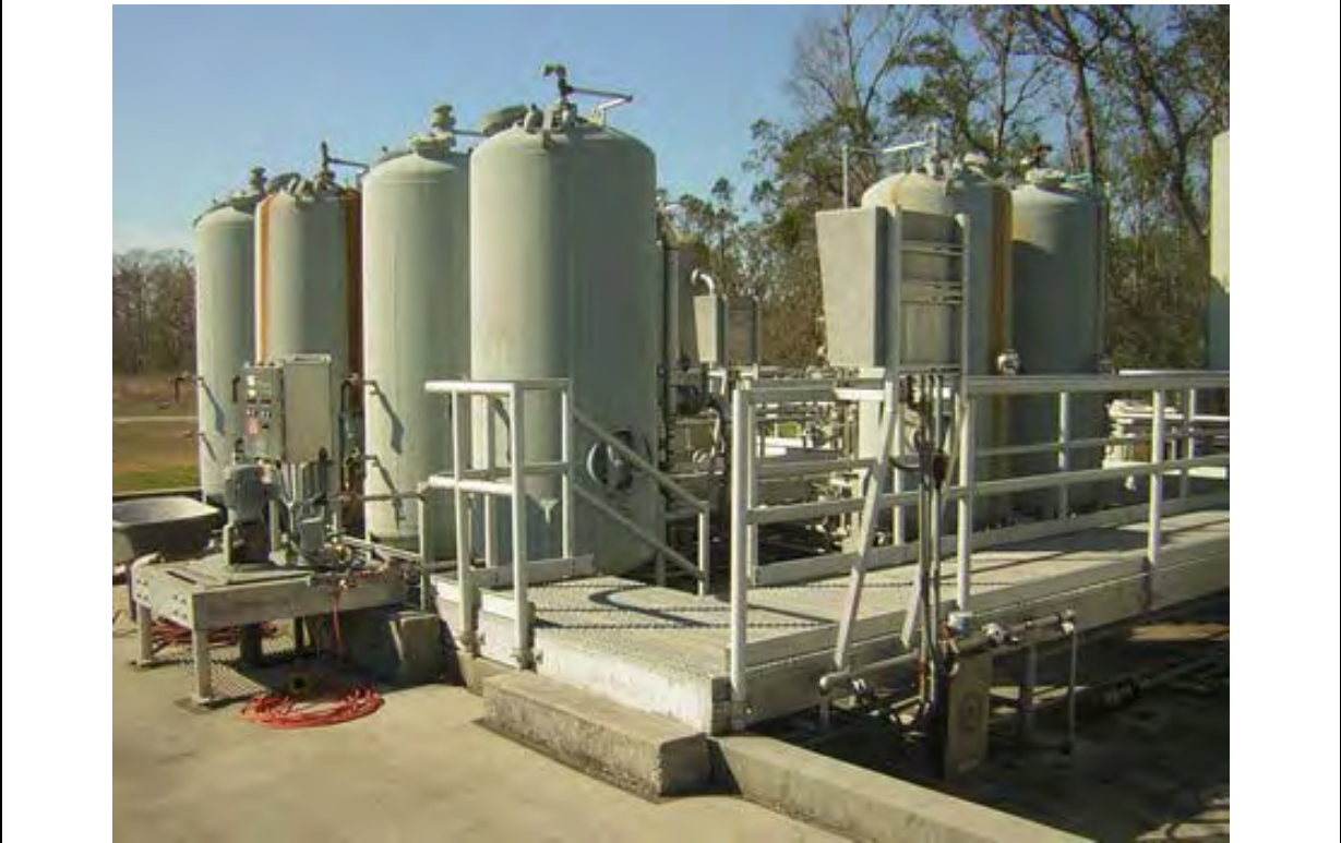
Photo 2: Bayou Bonfouca ground water treatment plant. Taken 2/16/2006
