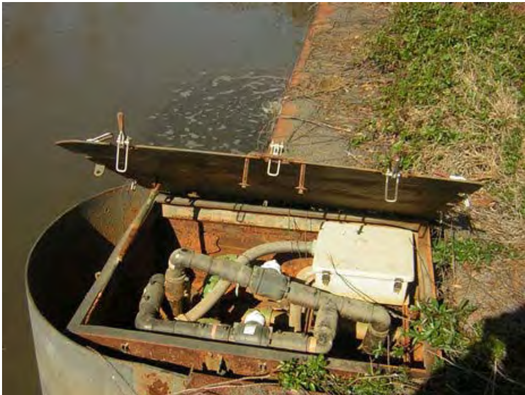
Photo 22: Vault for piping connection across bayou to recovery array 3, on east side of bayou. Taken 2/16/2006
