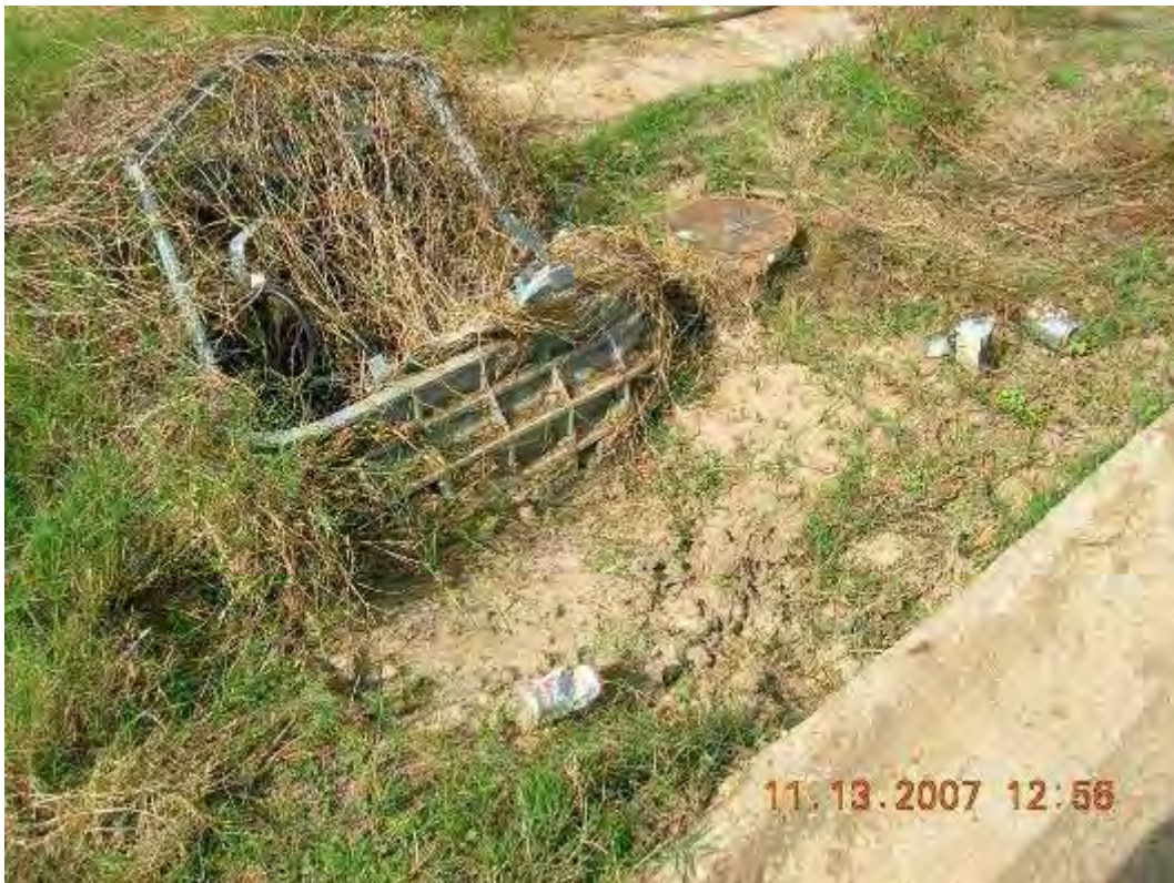
Photo 38: View of an excavated area near a water main line at Press Street. The geotextile liner was not exposed.
