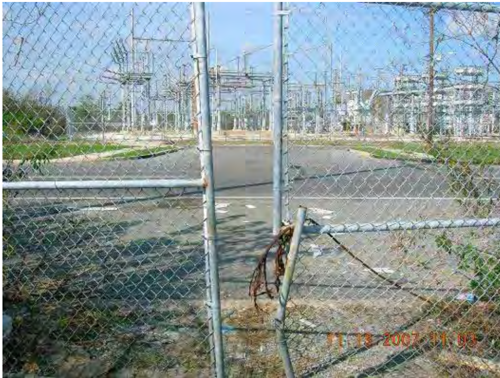
Photo 4: Inside OU 1, looking west through the security fence. Almonaster Blvd is in background. Chains and locks were removed at this gate. LDEQ personnel came back and placed new chains and lock on the gate.
