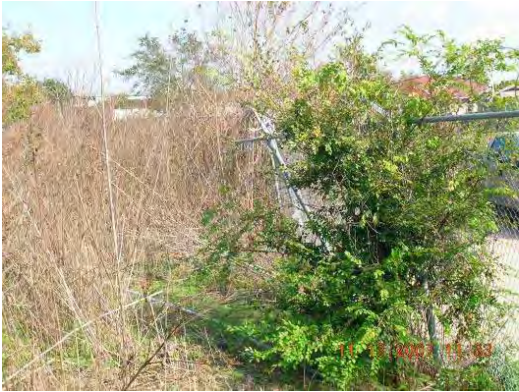
Photo 15: View of damaged fence near one of the gates at the corner of St. Ferdinand St. and Abundance St.
