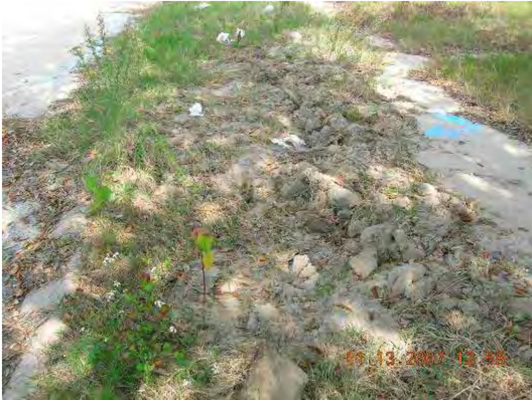
Photo 39: Evidence of digging along the sidewalk at Press Street near the corner of Benefit Street. The geotextile liner was not exposed.
