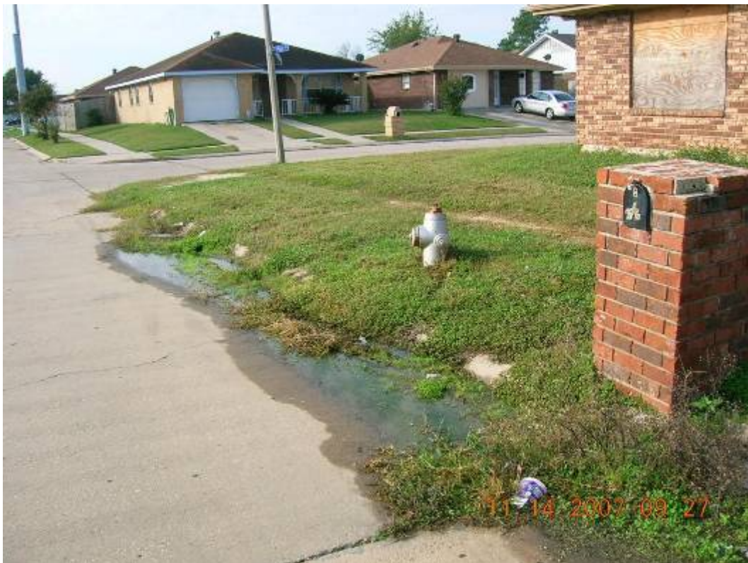
Photo 48: A water leak apparently from a fire hydrant. View is to the south at the corner of Press Street and Benefit Street.
