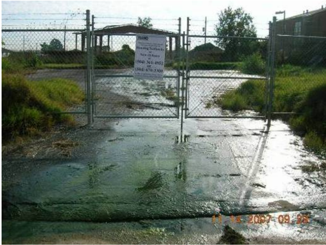
Photo 49: A water leak was spotted at this location apparently coming from one of HANO's apartments.
