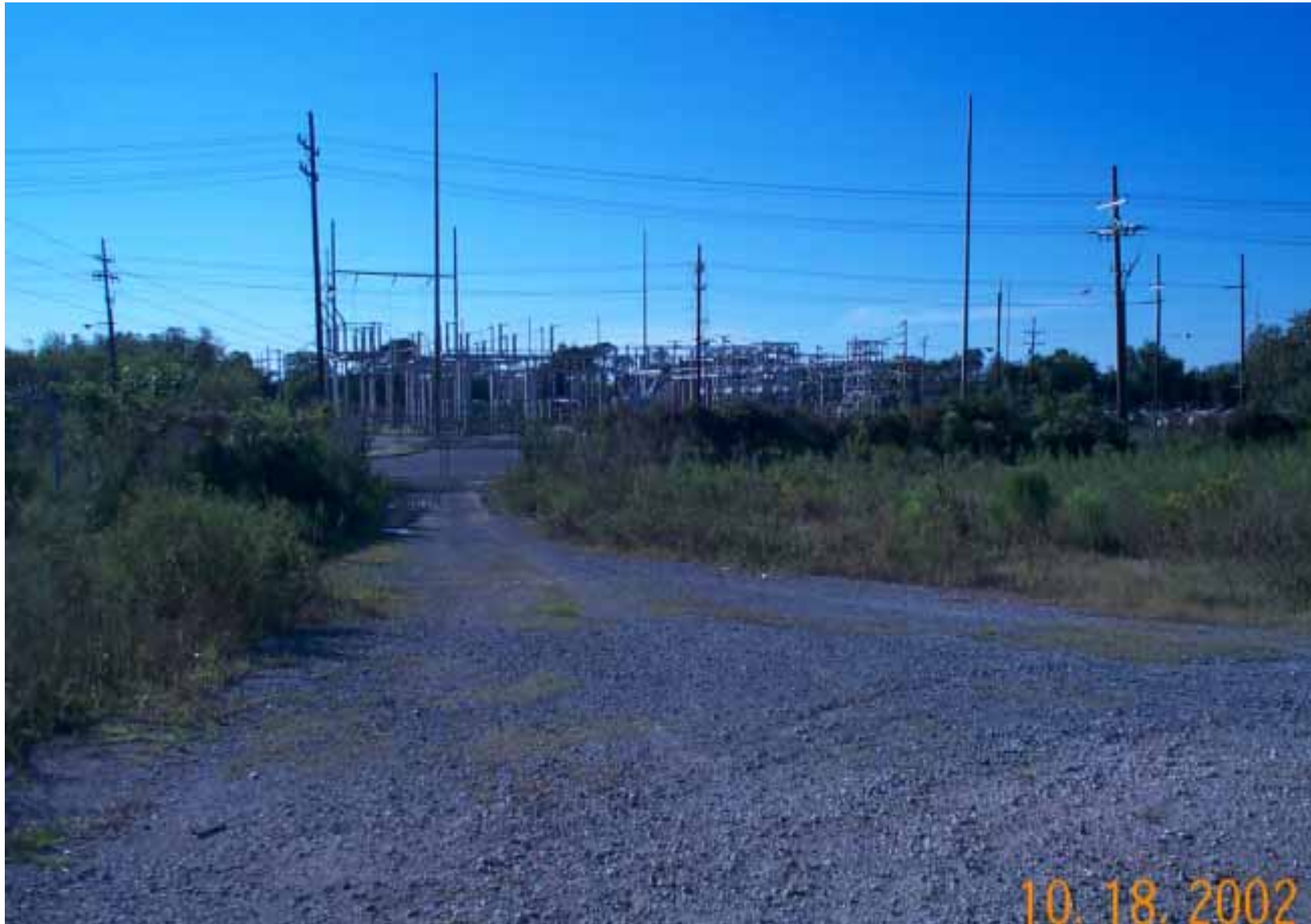
Photo 40: Looking west at gate and fence on OU1, and substation across Almonaster Boulevard. Graveled drive was used for entry to the command center area for response activities.
