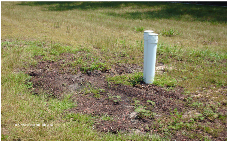
Photograph 15 Date: July 15, 2008 Site: Cleve Reber Superfund Site Description: Repair of surface water erosion (facing south).
