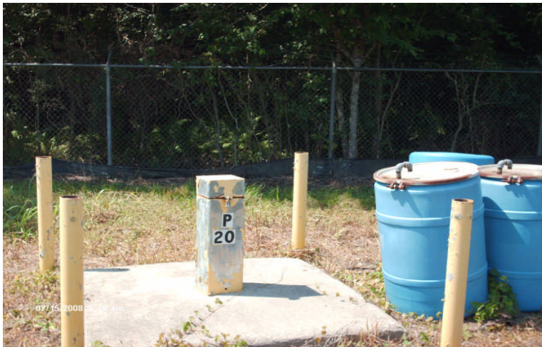
Photograph 3 Site: Cleve Reber Superfund Site Description: Monitoring well P-20 (facing south). Date: July 15, 2008
