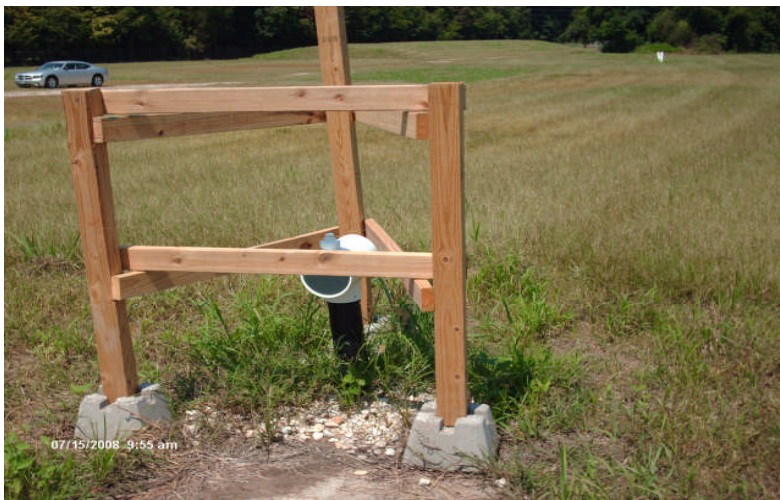
Photograph 7 Site: Cleve Reber Superfund Site Description: Gas venting system point V-3 (facing west). Date: July 15, 2008
