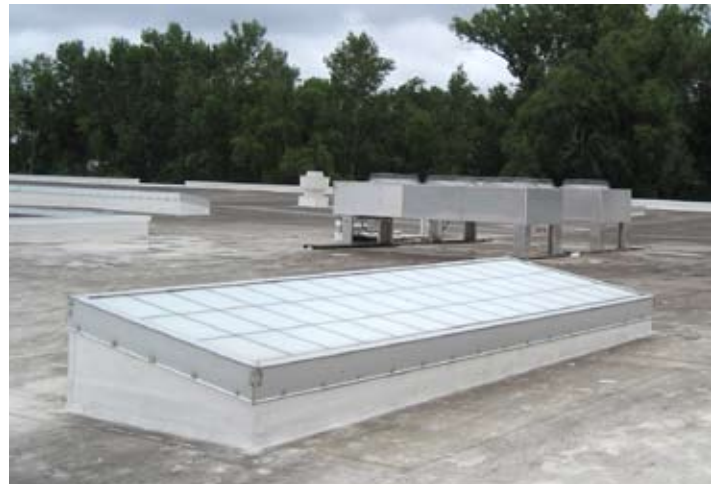
Skylights provide daylight where needed
