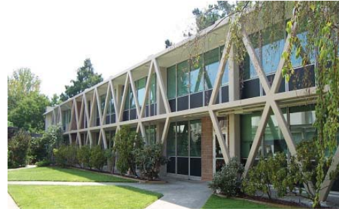
Example of exterior structural bracing that is part of the building's original design.
