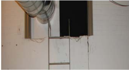
Ladder leading to the opening of a crawl space that is included in Gross.
