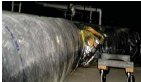
Crawl space inside opening of photograph at left. Note wheeled device used to lie on and roll within crawl space.
