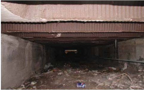
Unfinished crawl space. PBS does not consider an unfinished crawl space with dirt floor part of the total constructed area of a building and therefore is not included in the Gross.
