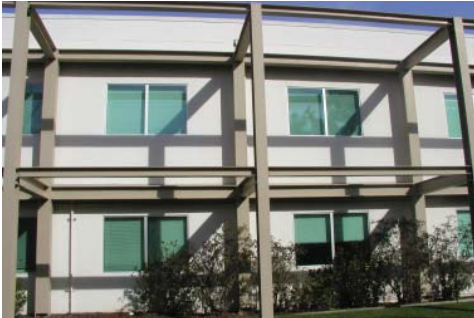
Example of an older building with exterior structural bracing added to improve earthquake resistance.
