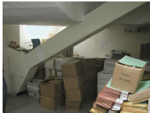
Space with a structural brace. This room is basement storage that is built out and is assigned as GNS.
