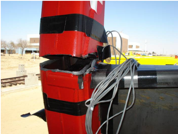
Figure 14. The back of the collision post, at the connection to the shelf, post-test (bottom)
