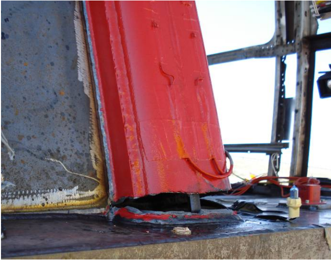
Figure 17. Fracture at the connection between the collision post and the buffer beam
