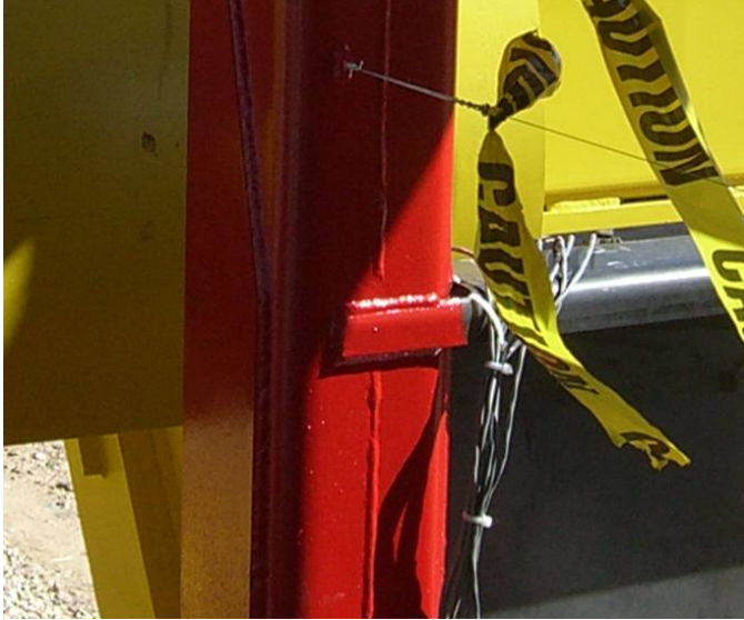
Figure 13. The back of the collision post, at the connection to the shelf, pre-test
