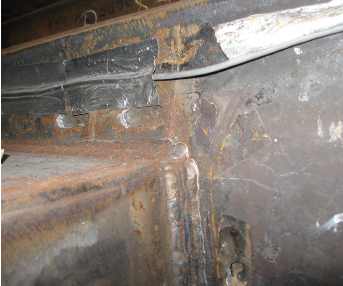
Figure 26. Three Failed Slot Welds
