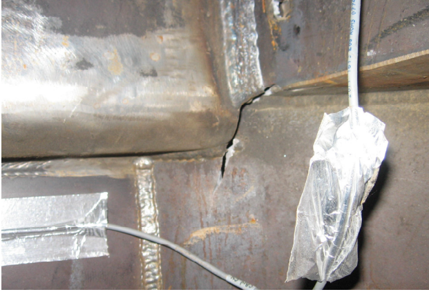
Figure 22. Crack on the Outside of the Bellmouth
