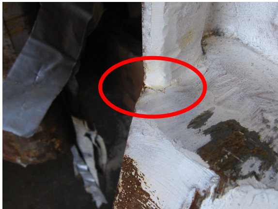
Figure 2. Cracks in the Coupler Head
