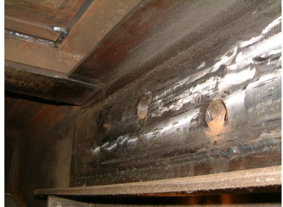
Figure 24. Signs of Scraping on the Fixed Sill Where the Sliding Sill Contacted
