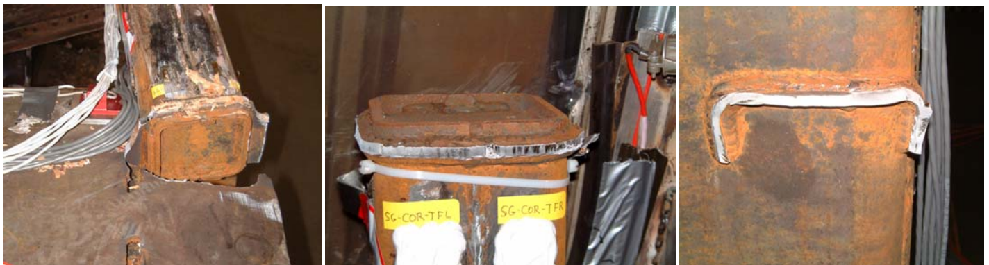
Figure 16. Post-Test Photographs of Material Failure in 1990's Design, Corner Post Connection to End Beam, Failed Connection at Top of Corner Post, and Failed Connection to Shelf on Collision Post
