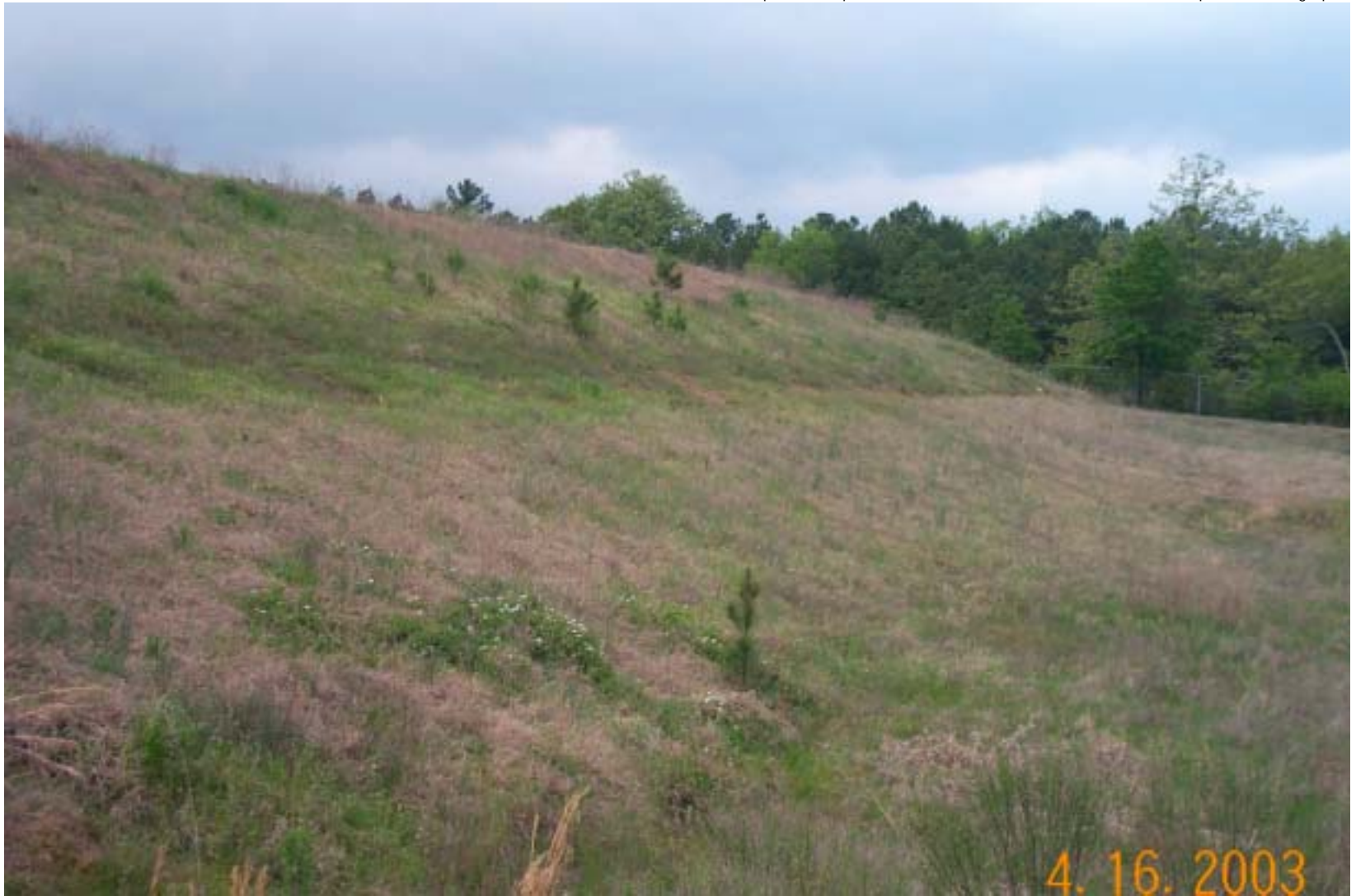
Photo 26: View of the north side of the OU1 landfill. View is facing west. Note small trees growing on the cap.
