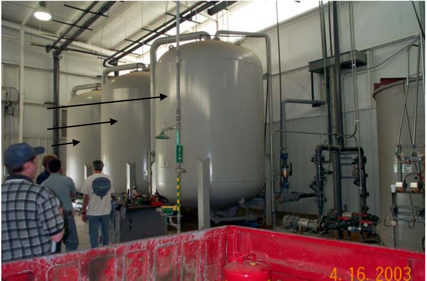
Photo 49: View inside Wastewater Treatment Plant. The three large tanks are the carbon treatment units (black arrows).
