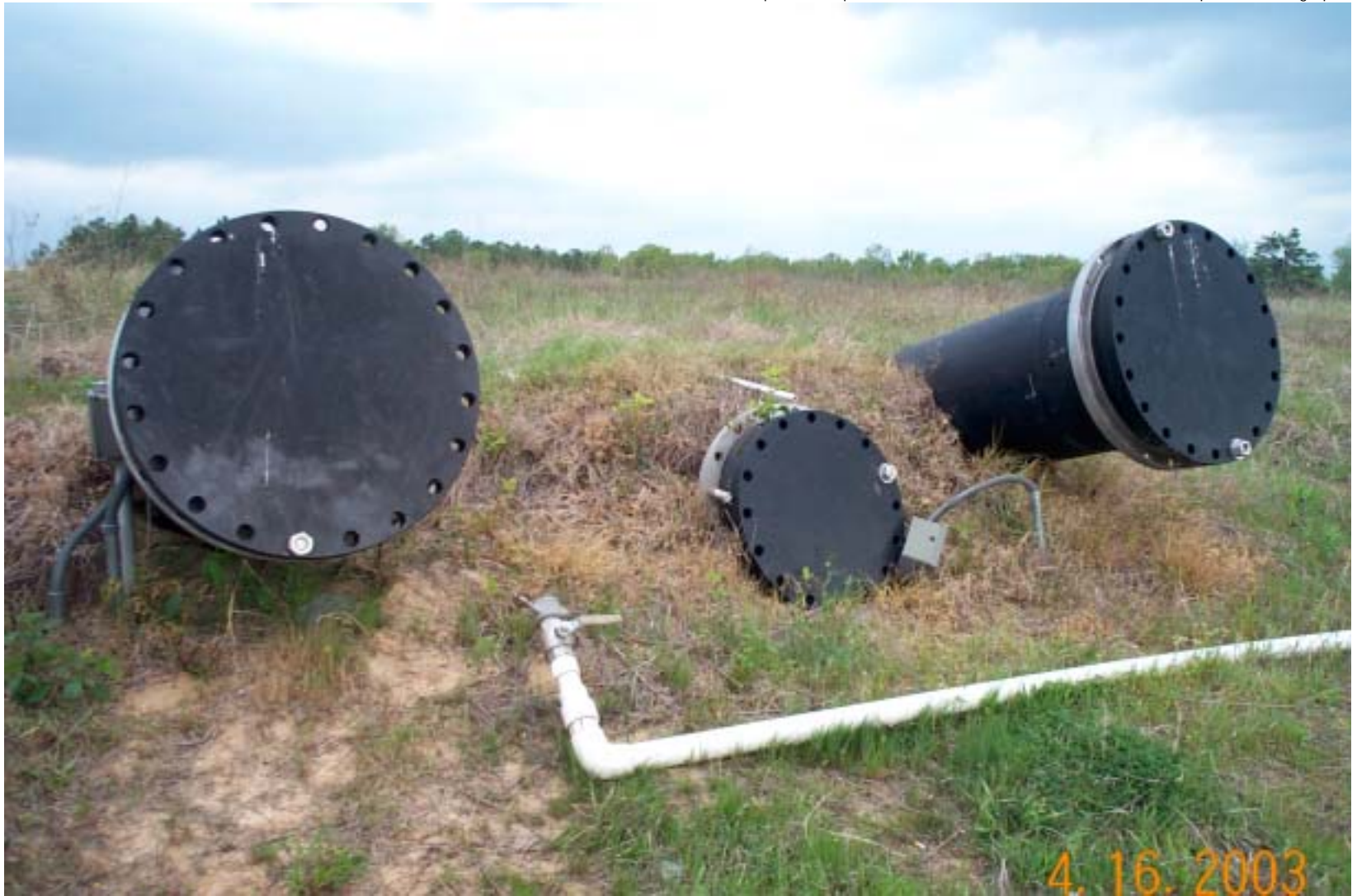
Photo 23: Access outlets for leachate collection and leachate detection sumps at the OU1 landfill.
