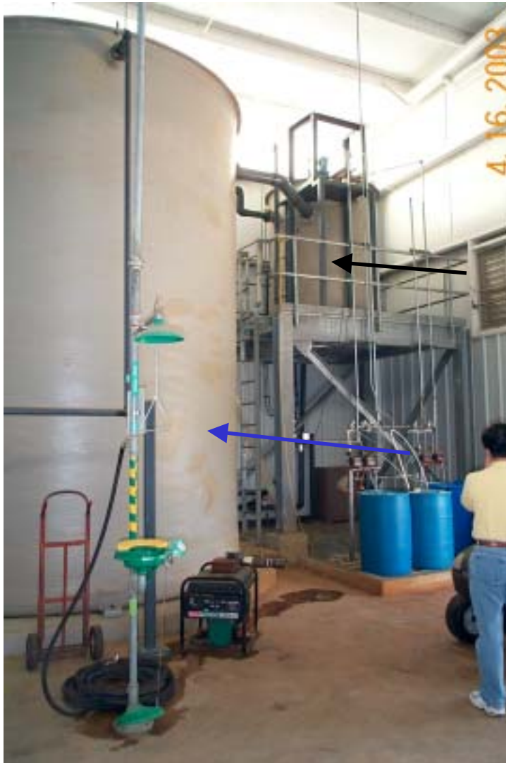
Photo 50: View inside Wastewater Treatment Plant. The large tank on top of the platform in the rear is the pH neutralization tank (black arrow). The tank to the left is the treated water tank (blue arrow).
