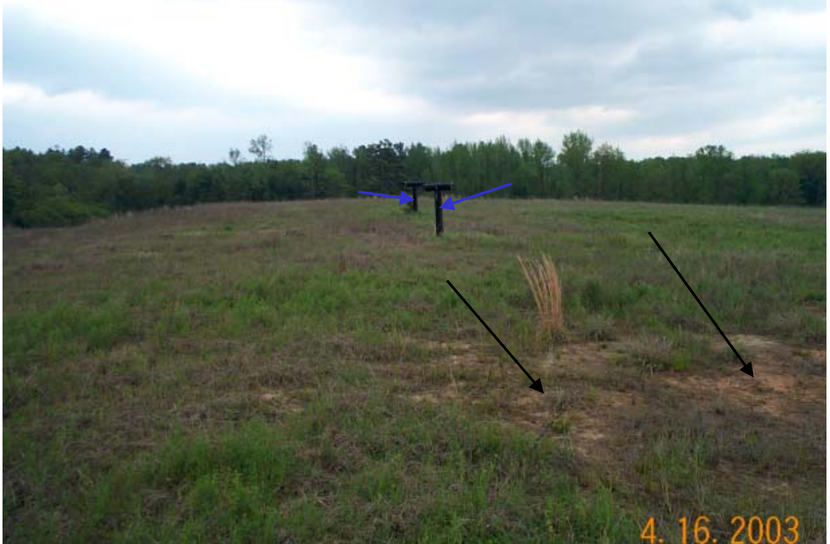
Photo 29: View of the top of the cap at the OU1 landfill. Note area of sparse vegetation (black arrow). Blue arrows are pointing to passive gas vents.
