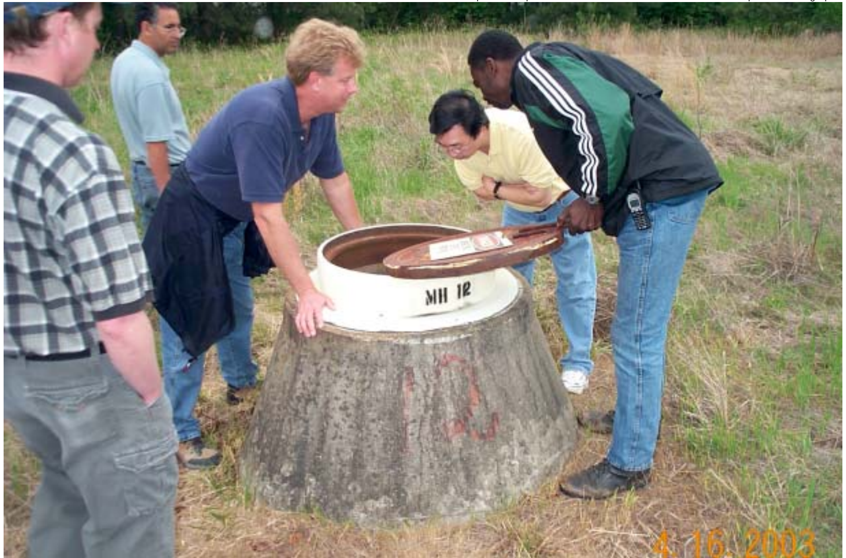
Photo 37: View of Manhole 12 of the french drain system. Manhole cover has been removed for inspection.
