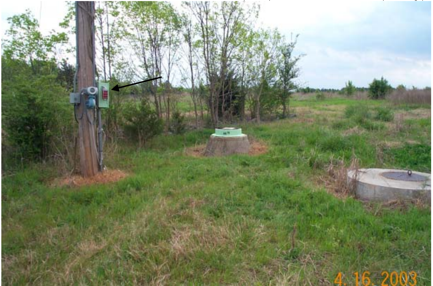
Photo 15: View of a french drain manhole. Controllers for pump and leachate level detectors are mounted on the pole to the left (arrow).
