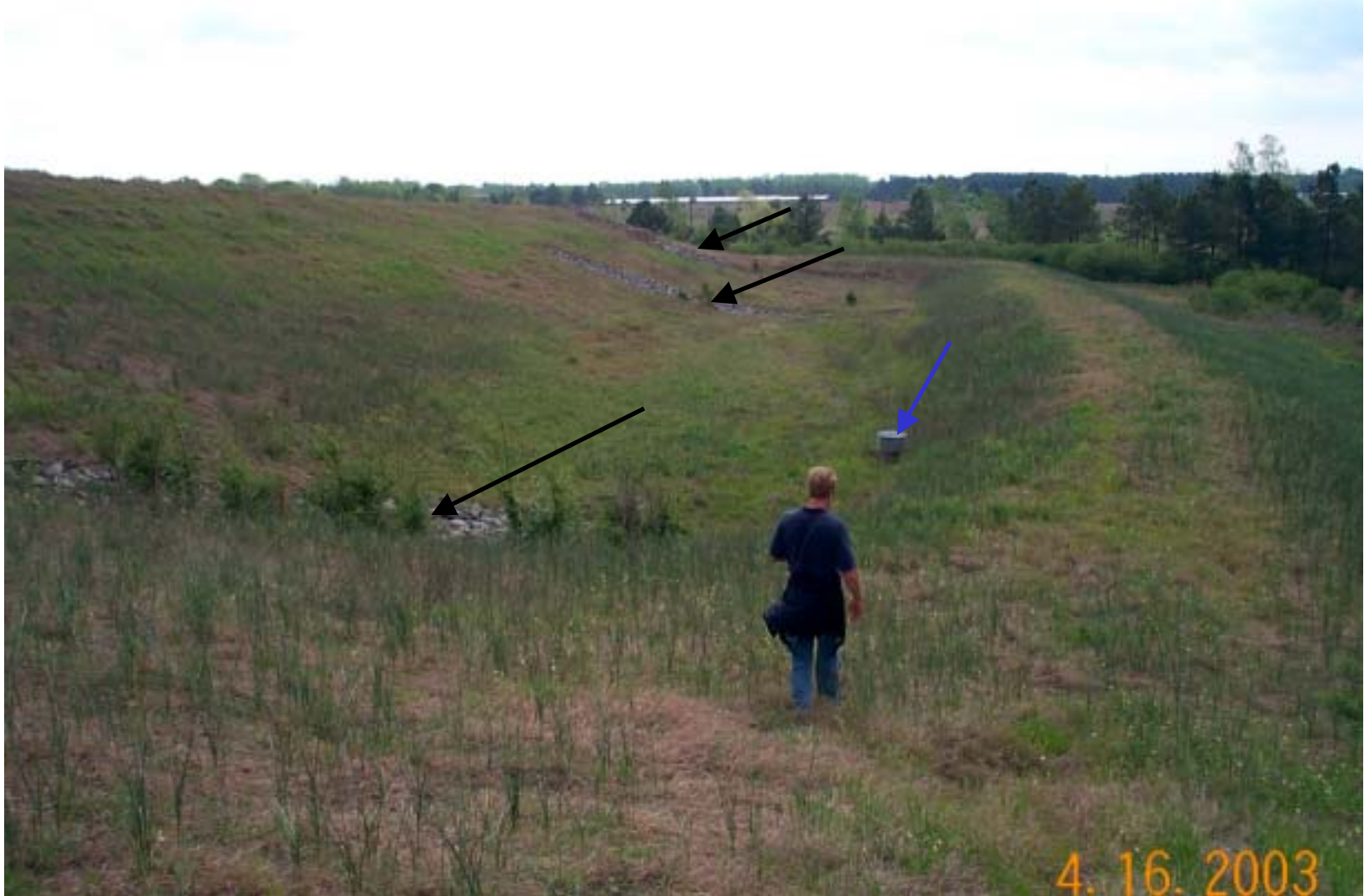
Photo 20: View of sedimentation basin at the south end of the OU1 landfill. View is to the east. Rock lined structures (black arrows) are letdown channels. Metal structure (blue arrow) is drainage pipe for the sedimentation basin.
