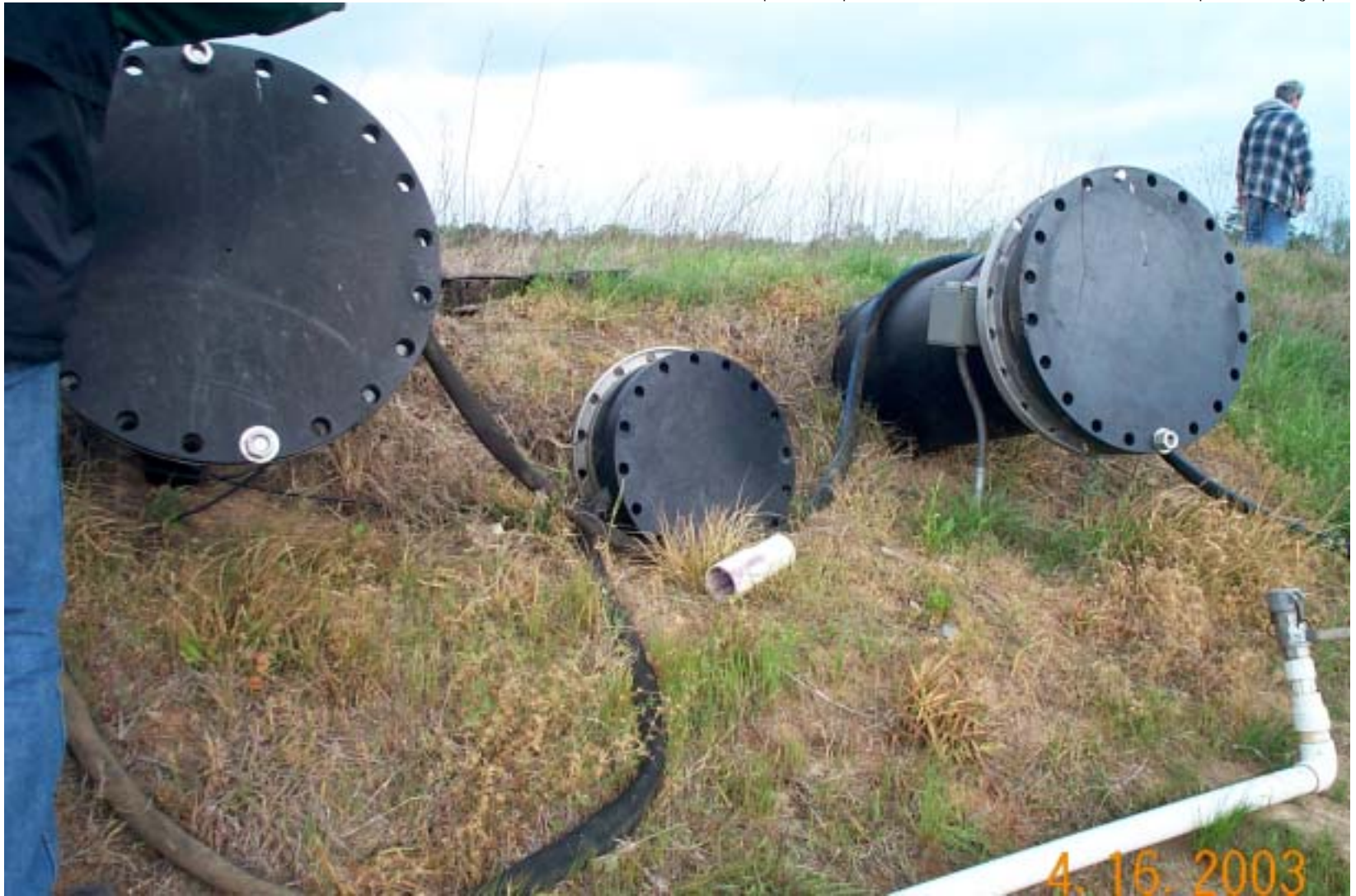
Photo 24: Access outlets for leachate collection and leachate detection sumps at the OU1 landfill.
