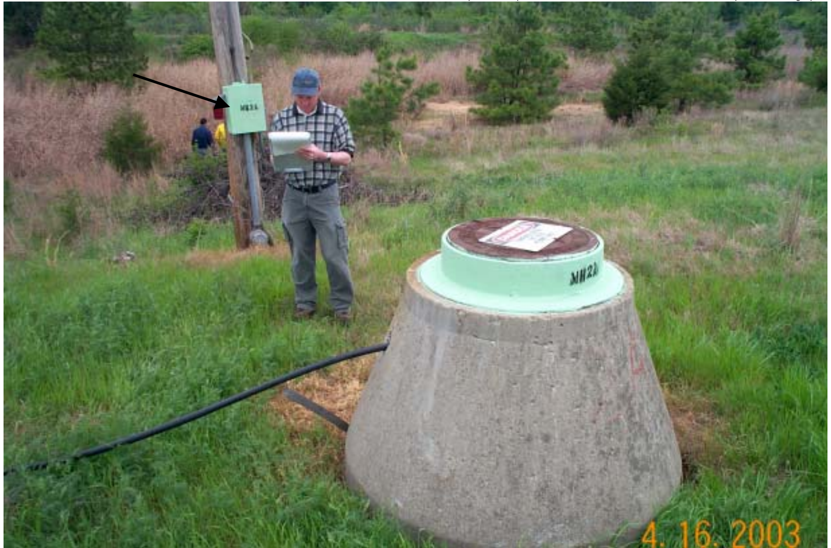
Photo 12: View of Manhole 2A of the french drain. The manhole contains a sump and pump to collect and remove leachate. The controller box for the pump and leachate level detector system is mounted on the pole in the background (at arrow).
