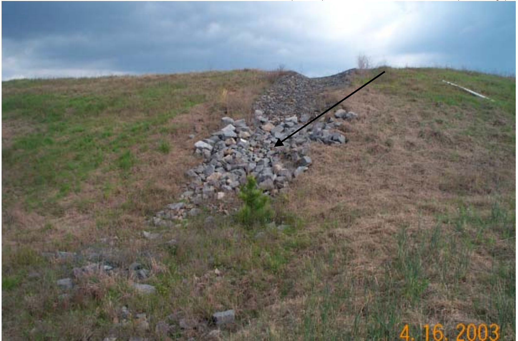
Photo 21: View of rock lined letdown channel (at arrow) at the OU1 landfill. These channels drain water from the top of the landfill cap. Note small tree growing along letdown channel in the center foreground.
