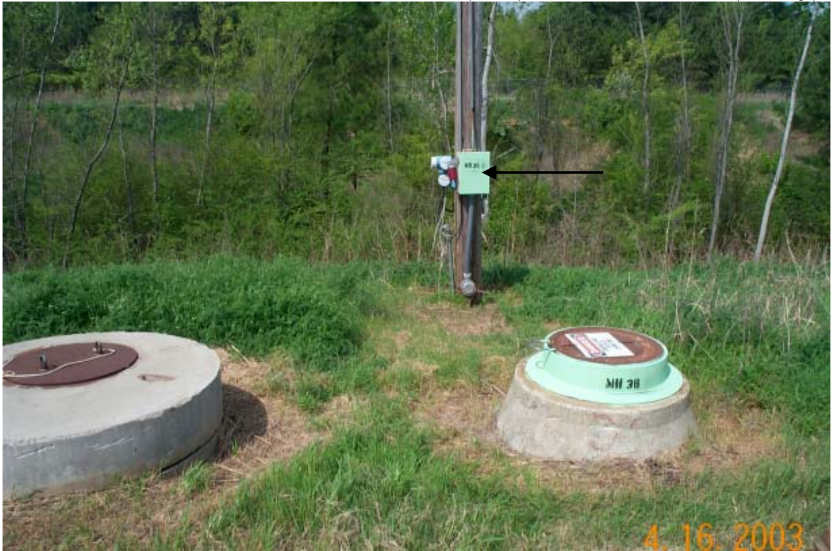
Photo 44: View of Manhole 3B of the french drain. The controller for the leachate level indicator and pump is on the pole behind the manhole (black arrow).
