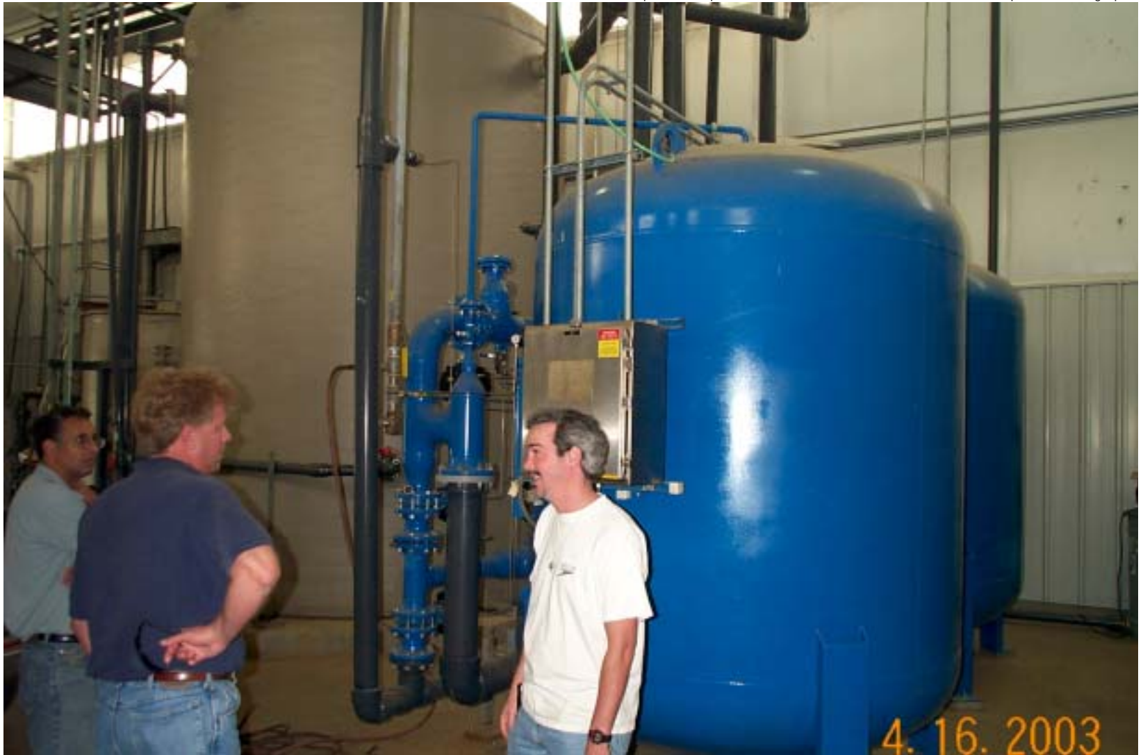
Photo 48: View inside Wastewater Treatment Plant. The two large blue tanks are the sand filters.
