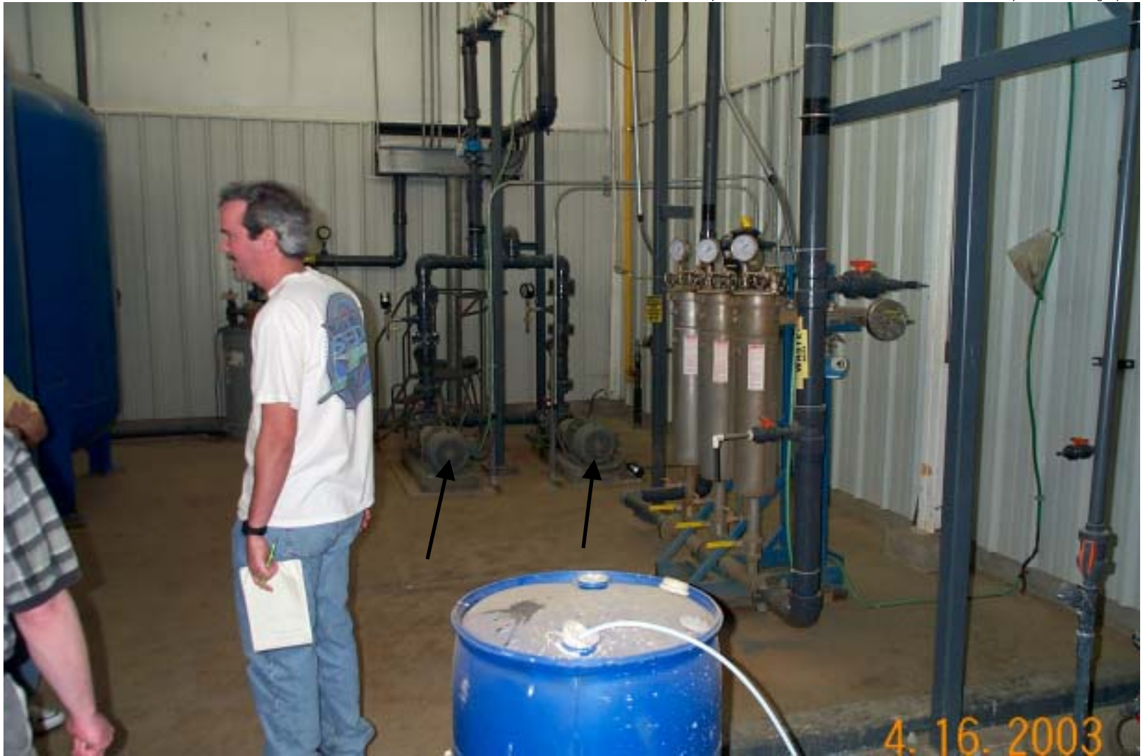
Photo 47: View inside Wastewater Treatment Plant. The pumps are on the floor next to the back wall (black arrows).
