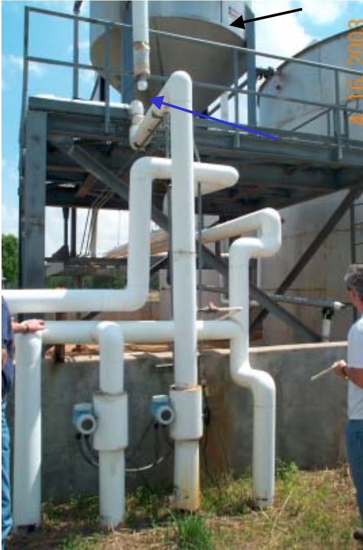
Photo 45: View of inlet pipes from french drain and ground water extraction systems at the waste Wastewater Treatment Plant. Tank at top of photo is the oil/water separator (black arrows). Note that the inlet pipes are no longer connected to the oil/water separator (blue arrow).
