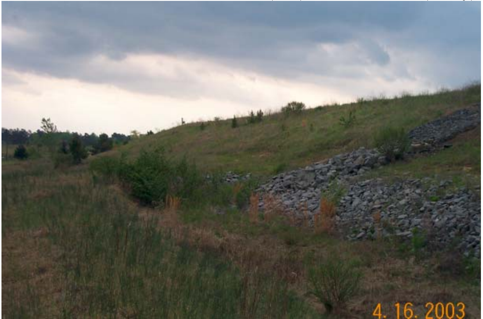
Photo 25: View of the east side of the OU1 landfill. View is facing south. Note small trees growing on the cap.
