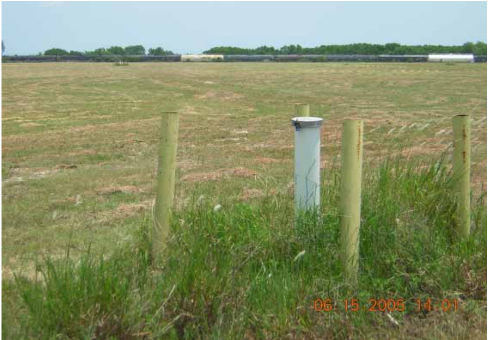
Photo 35: OU2: Site groundwater monitoring well. ID tags and locks were missing (facing east).
