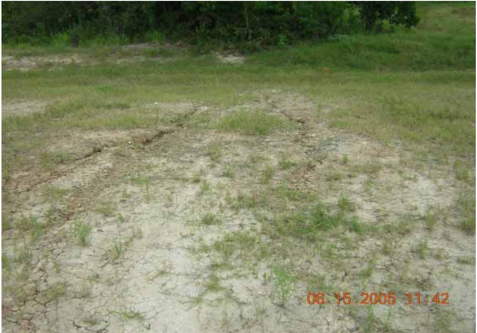
Photo 28: OU1: Erosion cuts in the north east slope of the Consolidation Cell (Pond 2).
