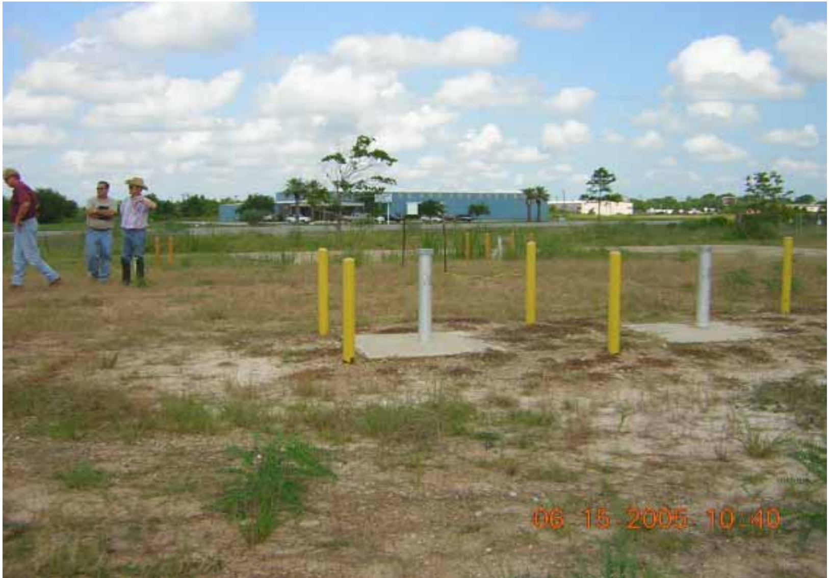
Photo 5: OU1: Groundwater monitoring wells on west side of site. All ID tags and locks are in place.
