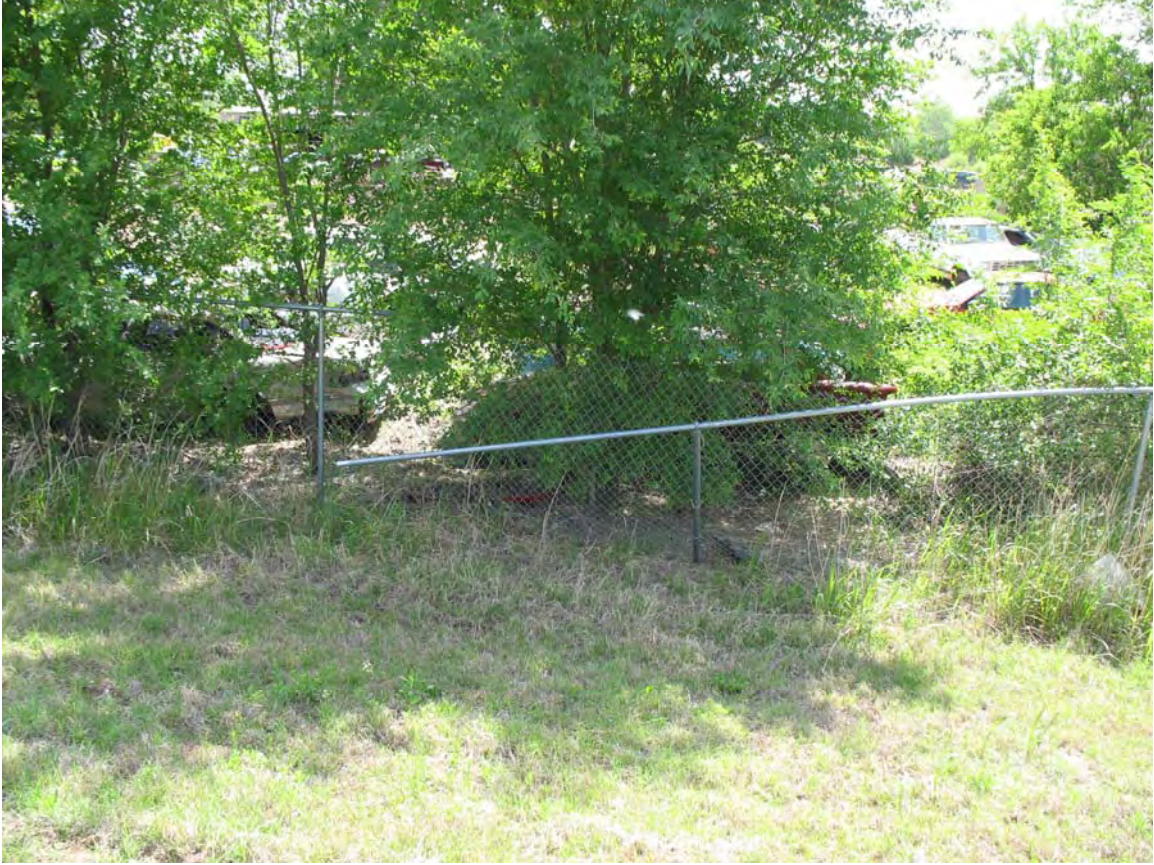
Photo 3. Bent post in the fence on the East side of the Tenth Street Superfund site.
