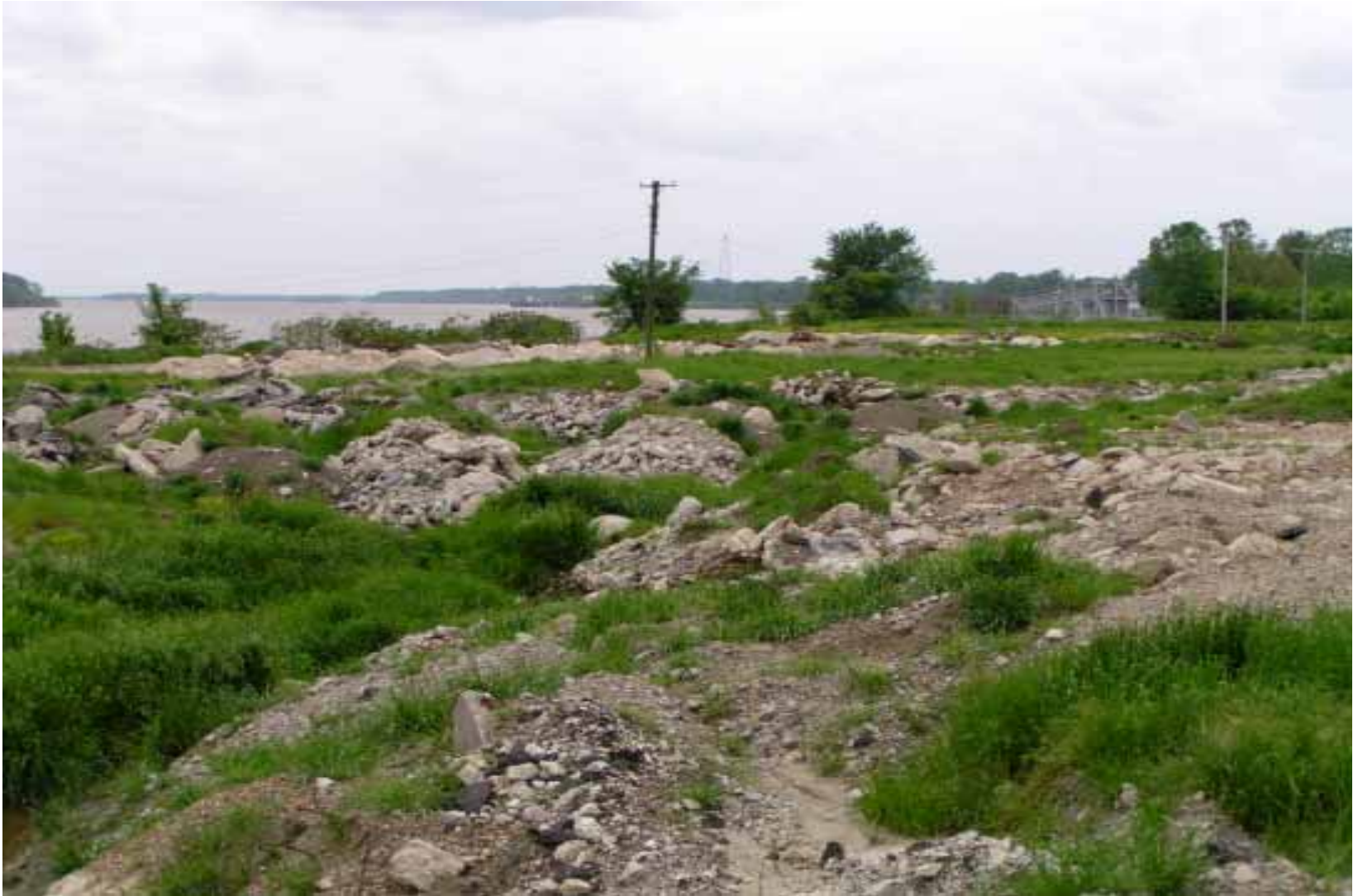
View orientated southward of the fill material being added to the raise the ground elevation between the Mississippi River and the top of the oily sludge mound. April 2004.
