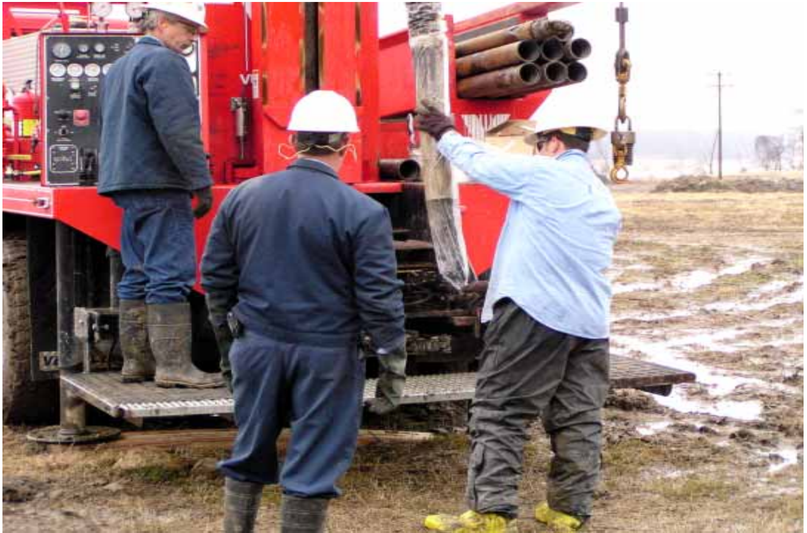
The stabilized/solidified material from the mound area is extruded from the core barrel. February 2004.
