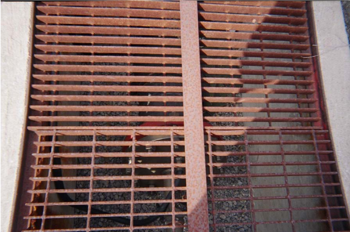
Photograph No. 3 Orientation: Down Description: Leachate collection vault with pump
