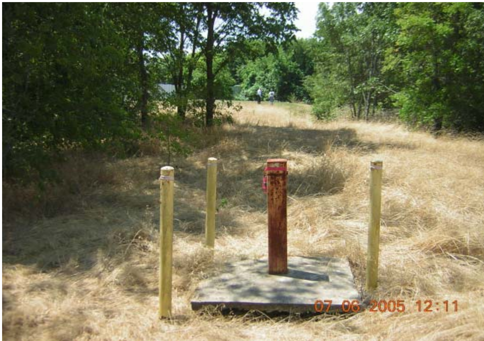
Photo 19: OU3, Site 3 – View of monitor well. Settlement can be observed at the base of the well's concrete pad.
