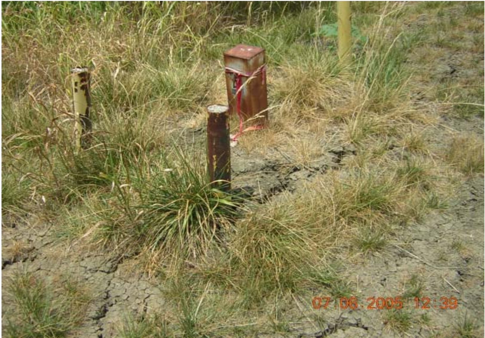
Photo 22: OU3, Site 3 – View of monitor well near soil cover in northern area of site. Monitor well lacks a well pad.
