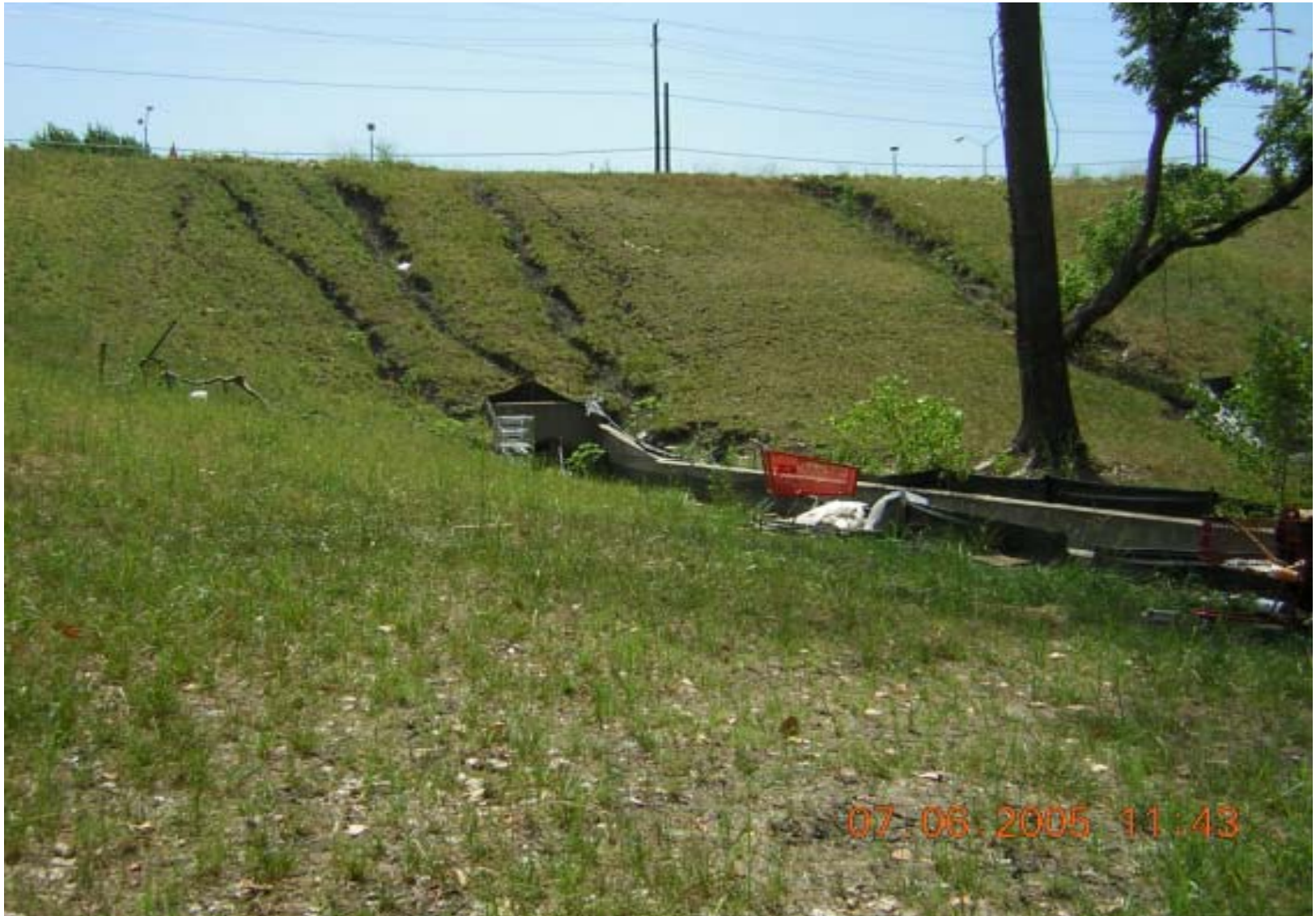
Photo 16: OU3, Site 1 – View up the slope of the erosion channels in the slope. View is facing to the east.
