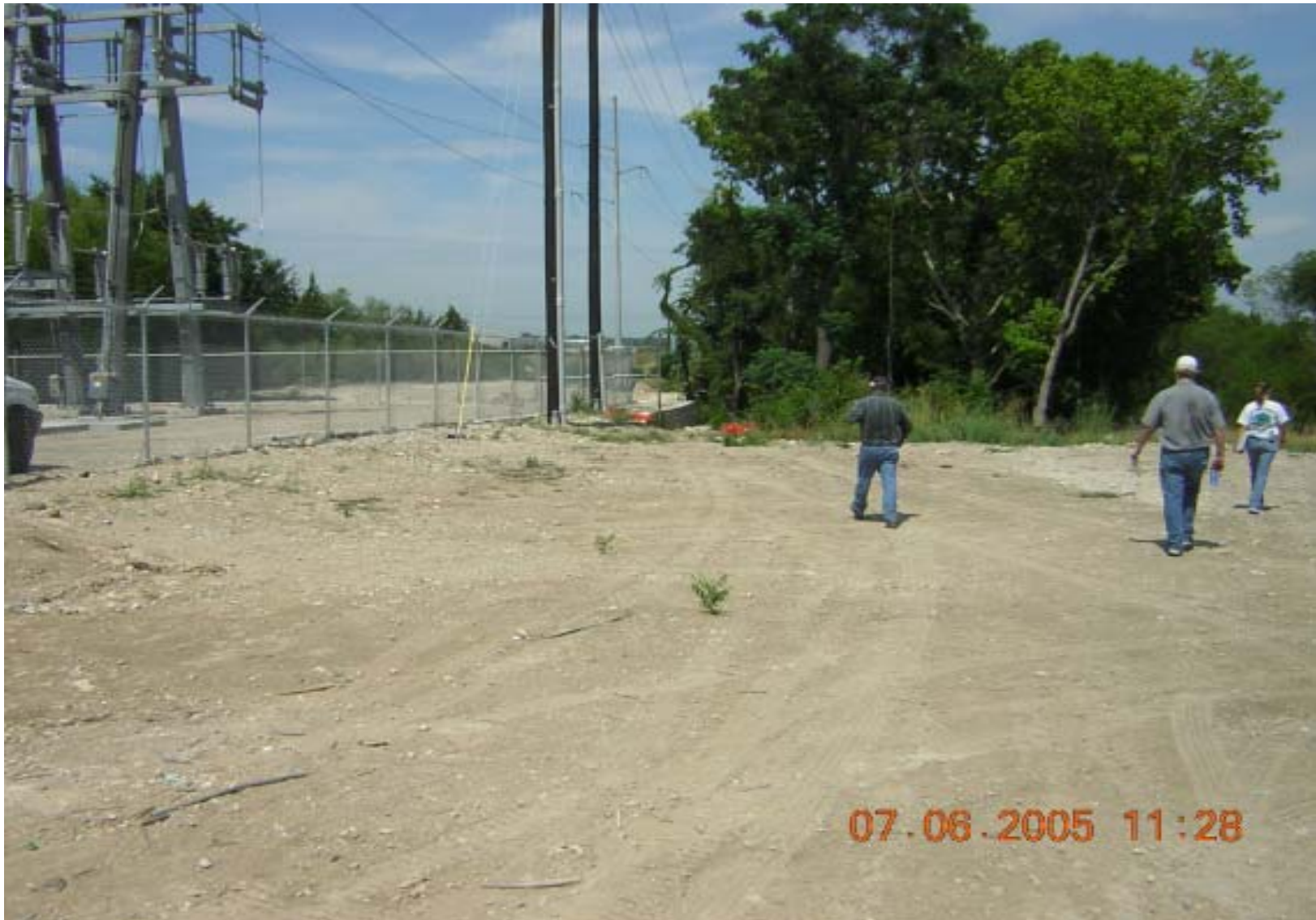
Photo 12: OU3, Site 1 – View of electrical substation built on property to the south of site, facing west.
