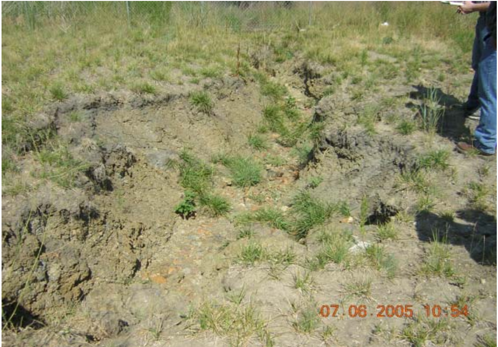
Photo 10: OU5, Subarea 2 – view of large erosion channel near fence just west of cover over former landfill.
