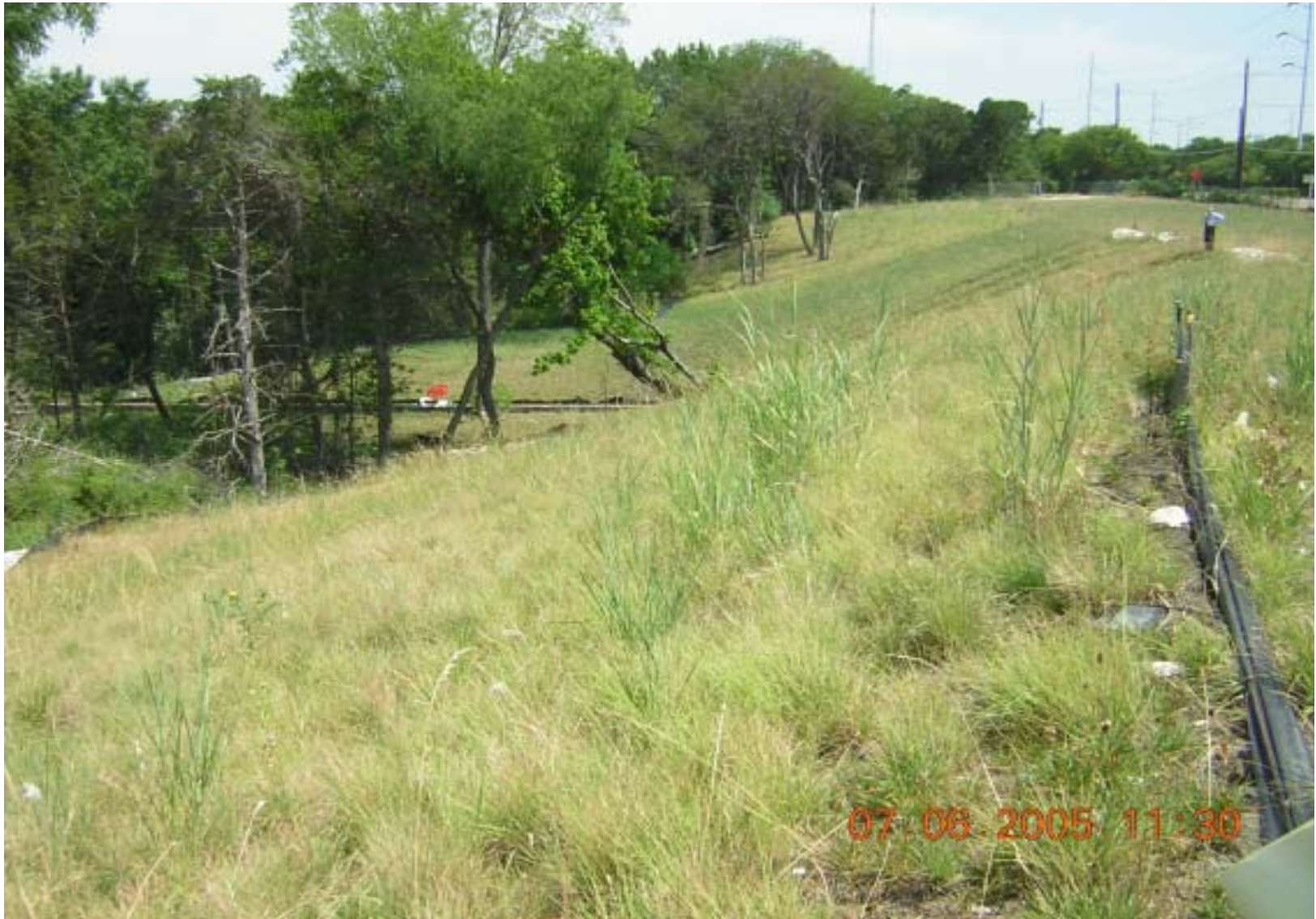
Photo 13: OU3, Site 1 – View of slope in middle of site. Erosion channels are visible in middle of slope. Rock material was placed on top of slope. View is facing north.
