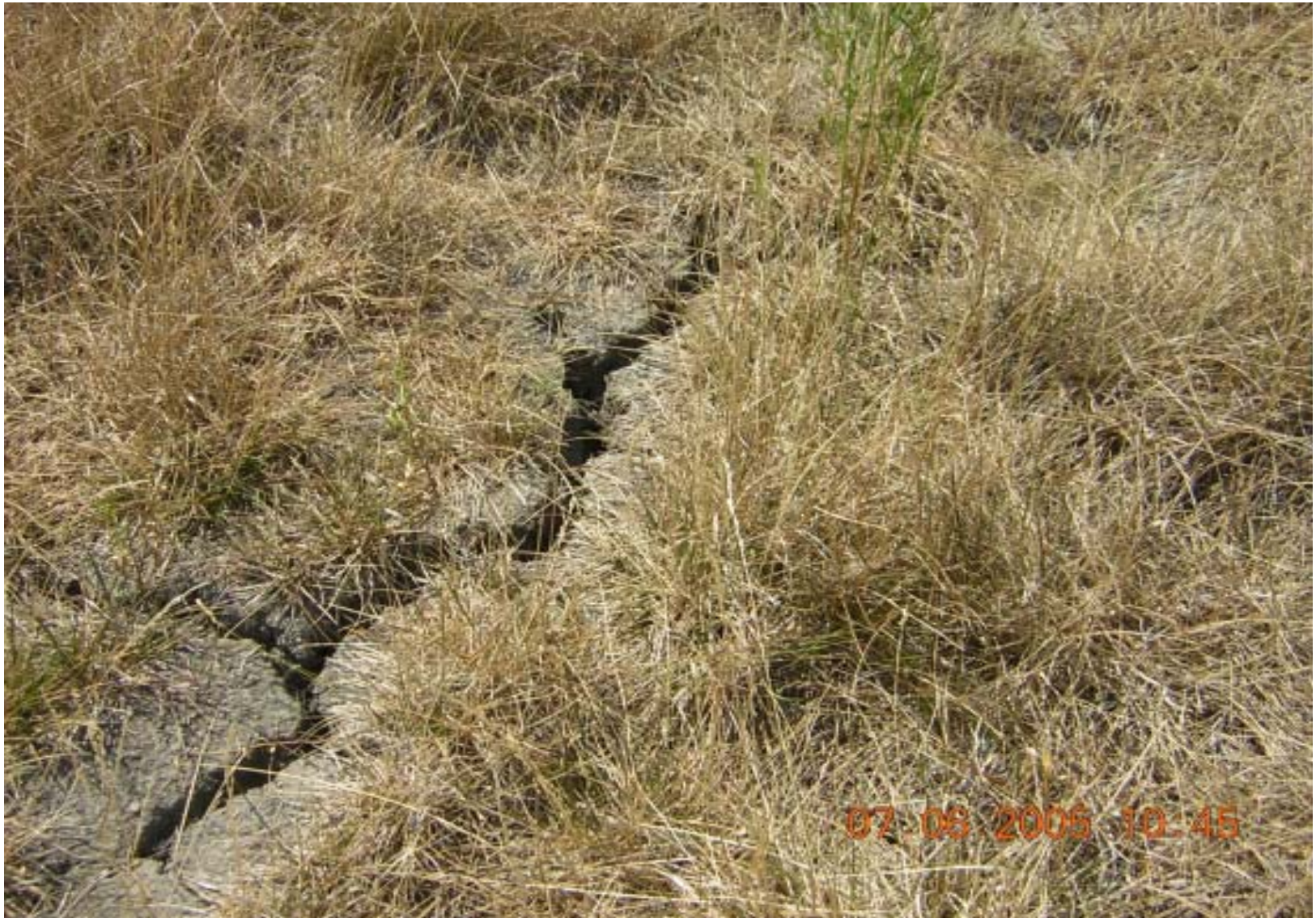
Photo 4: OU5 – Subarea 2 – view of desiccation crack in cover.
