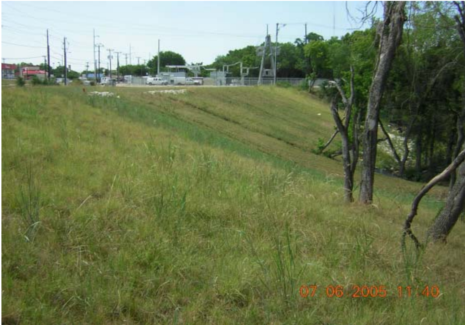
Photo 14: OU3, Site 1 – View of slope in middle of site. Erosion channels are visible in middle of slope. Rock material was placed on top of slope. View is facing south.
