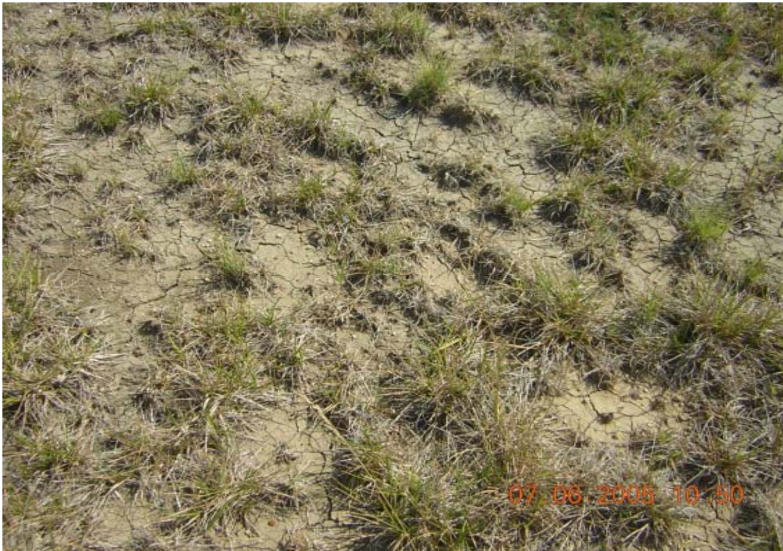
Photo 7: OU5, Subarea 2 – view of sparse vegetation and minor desiccation cracking in cover over former landfill.
