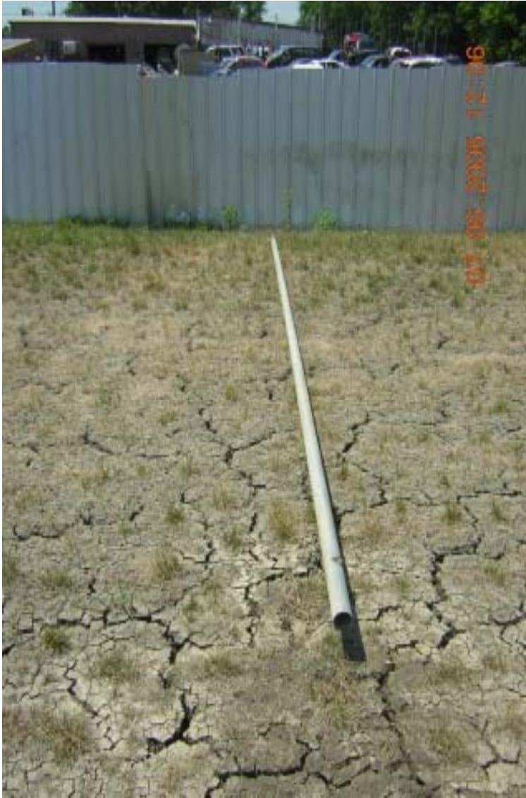
Photo 17: OU3, Site 3 – View of one of the discharge pipes placed by adjacent property owner on the cover at the southern portion of the Site. Also, desiccation cracks are present on the cap.
