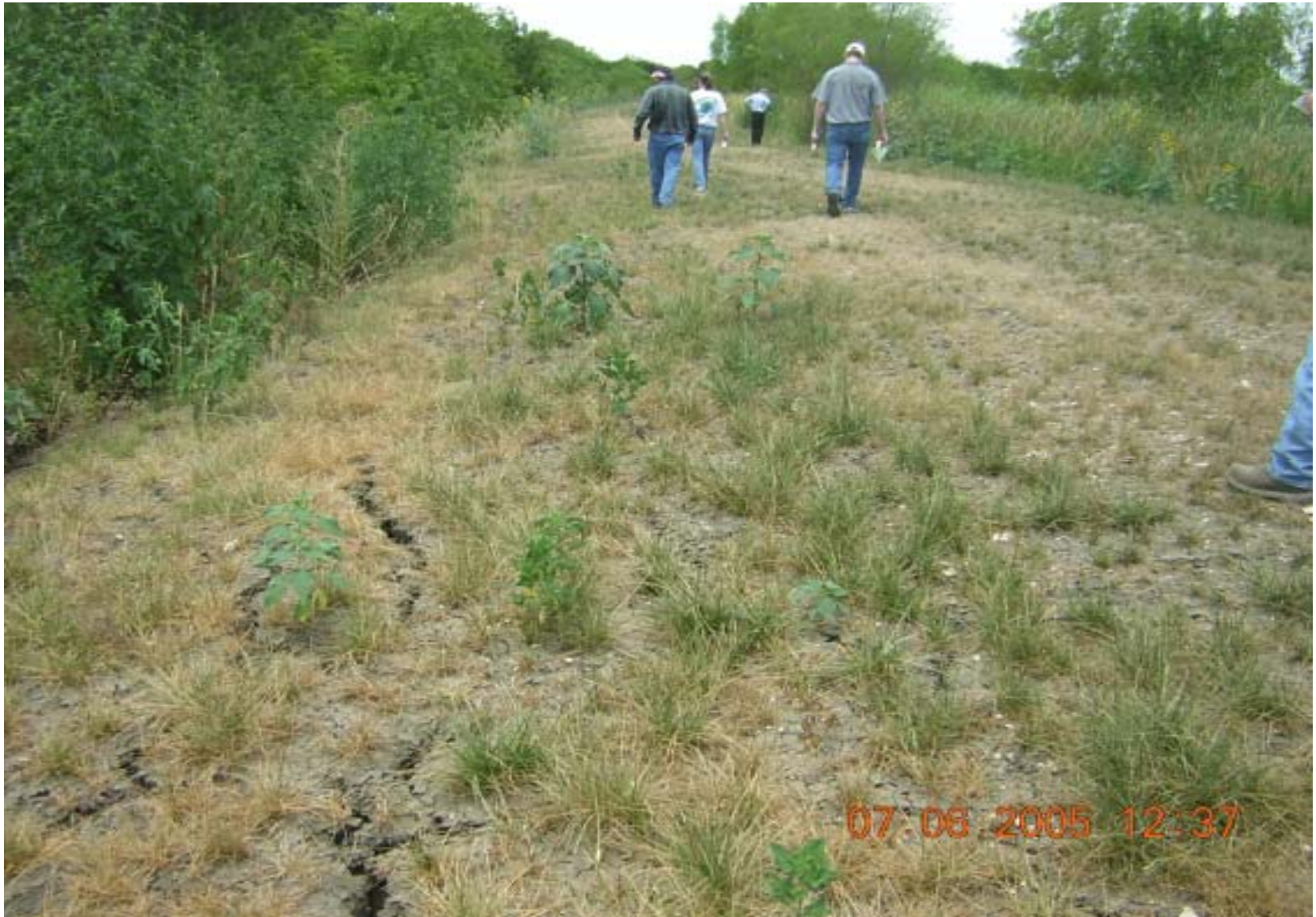
Photo 21: OU3, Site 3 – View of the soil cover in the northern portion of the site. The vegetation is sparse and large desiccation cracks are observed in this photo. View is facing west.
