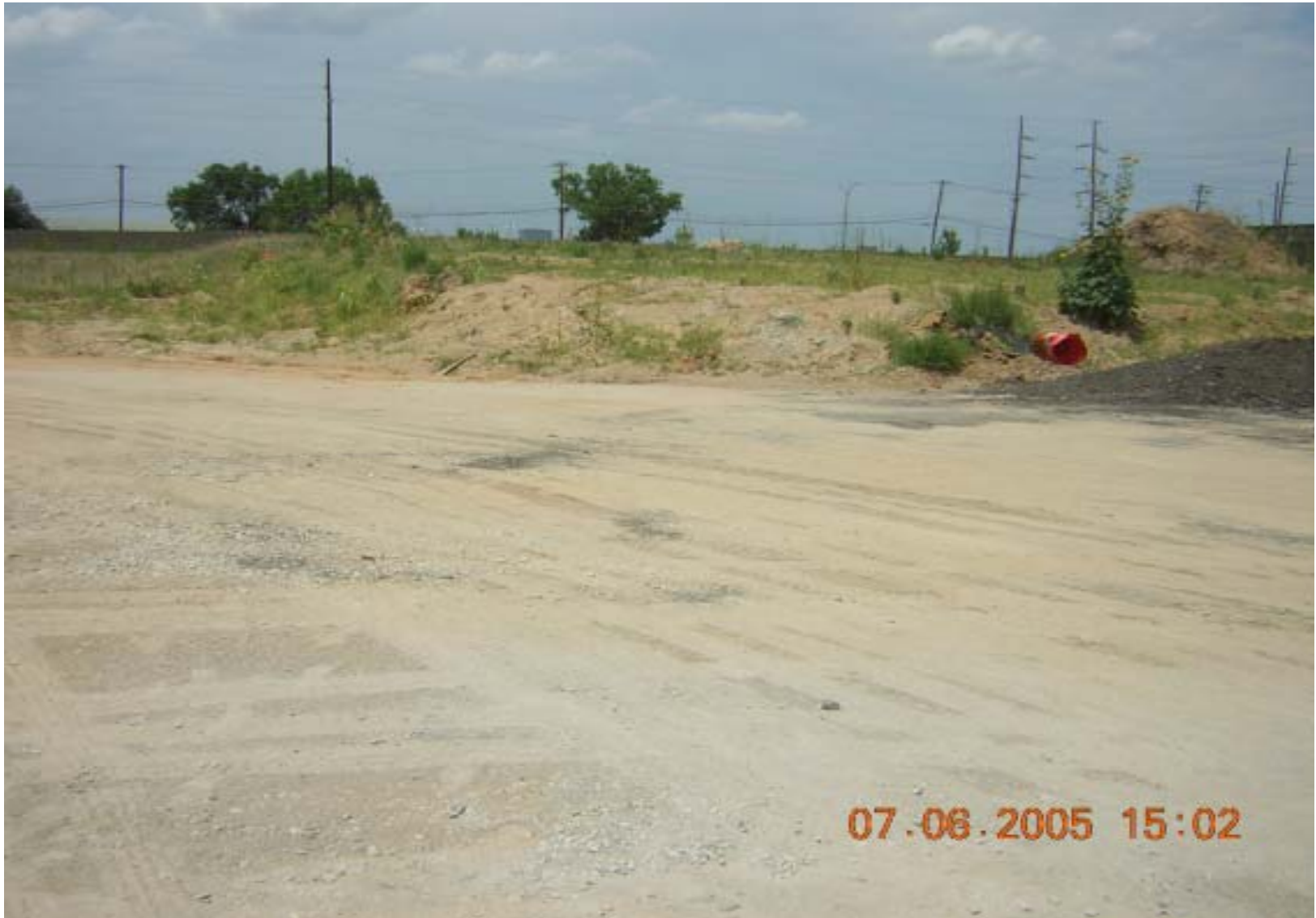
Photo 36: OU4 – View of road surface and stockpiled dirt placed on site by construction company that is leasing the property.
