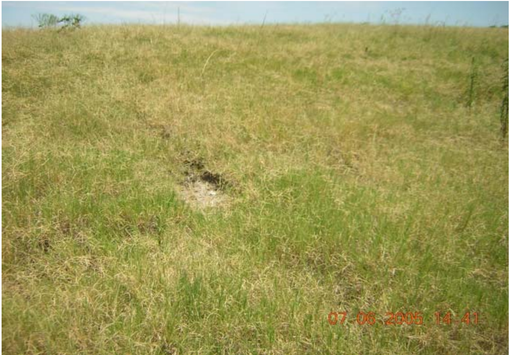
Photo 32: OU5, Subarea 1 – View of bare spot on cover at the former surface impoundment.
