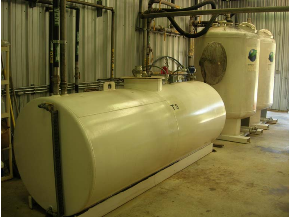
Photograph No. 9 Site: Madisonville Creosote Works Orientation: Southwest (Wastewater treatment plant interior) Date: 30 September 2008 Description: Creosote holding tank; TIGG carbon filtration tanks in background to the right
