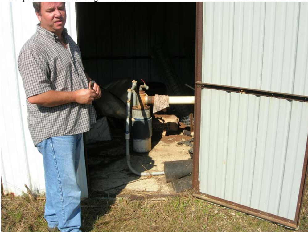
Photograph No. 24 Orientation: West Description: Water well #1
