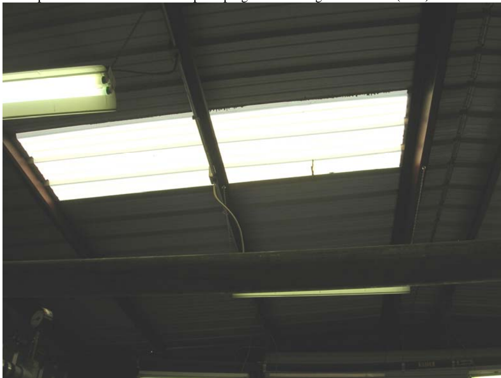
Photograph No. 12 Site: Madisonville Creosote Works Orientation: West (Wastewater treatment plant interior) Date: 30 September 2008 Description: Skylight that required sealing following Hurricane Gustav (1 Sept 2008)
