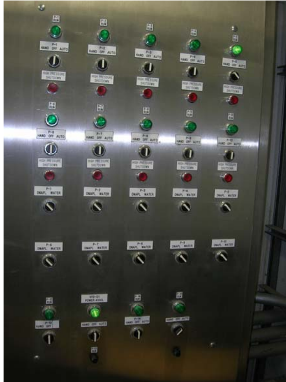
Photograph No. 11 Site: Madisonville Creosote Works Orientation: North (Wastewater treatment plant interior) Date: 30 September 2008 Description: Wastewater treatment plant programmable logic controllers (PLC) screen
