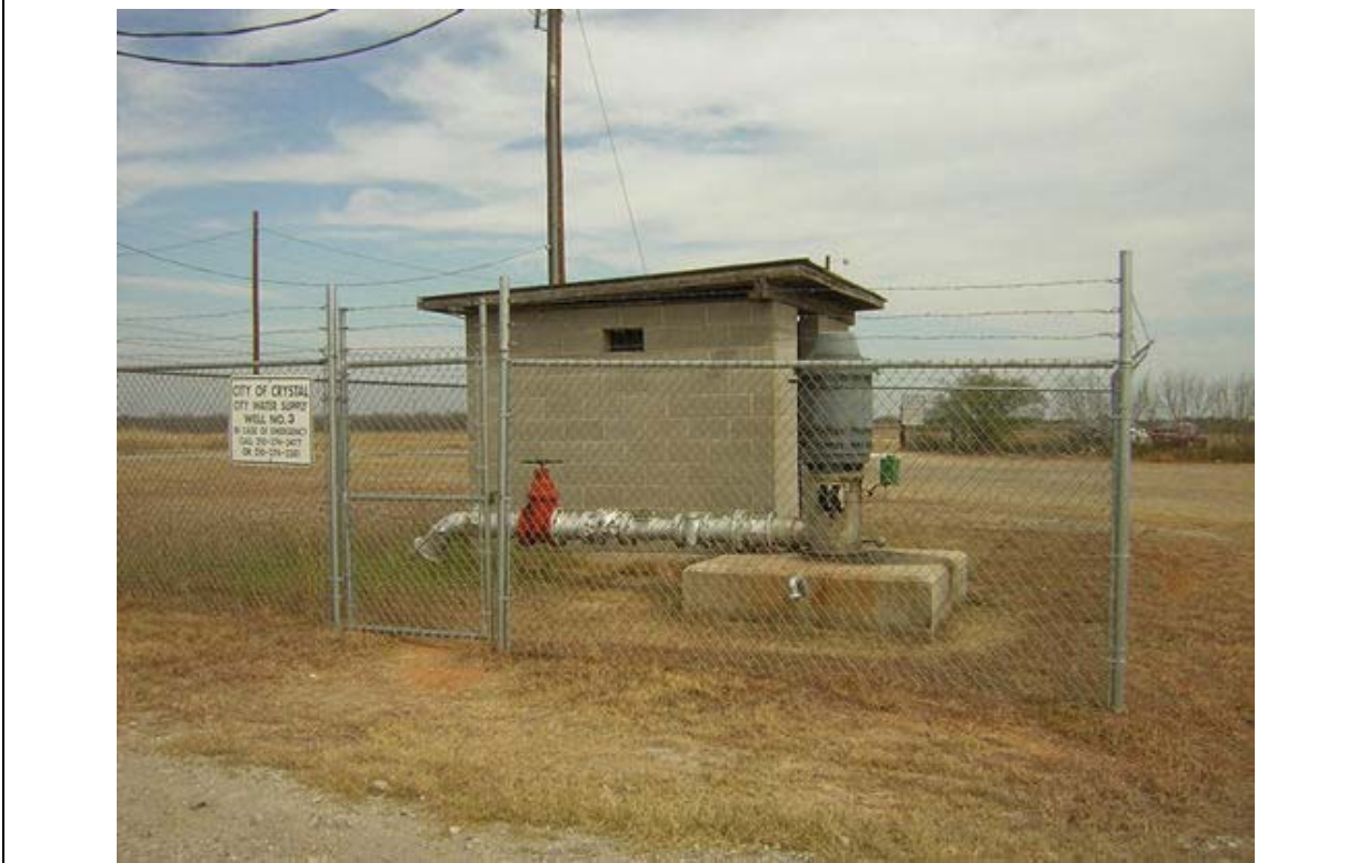
Photo 8: City of Crystal City Supply Well No. 3 (southeast of airport).
