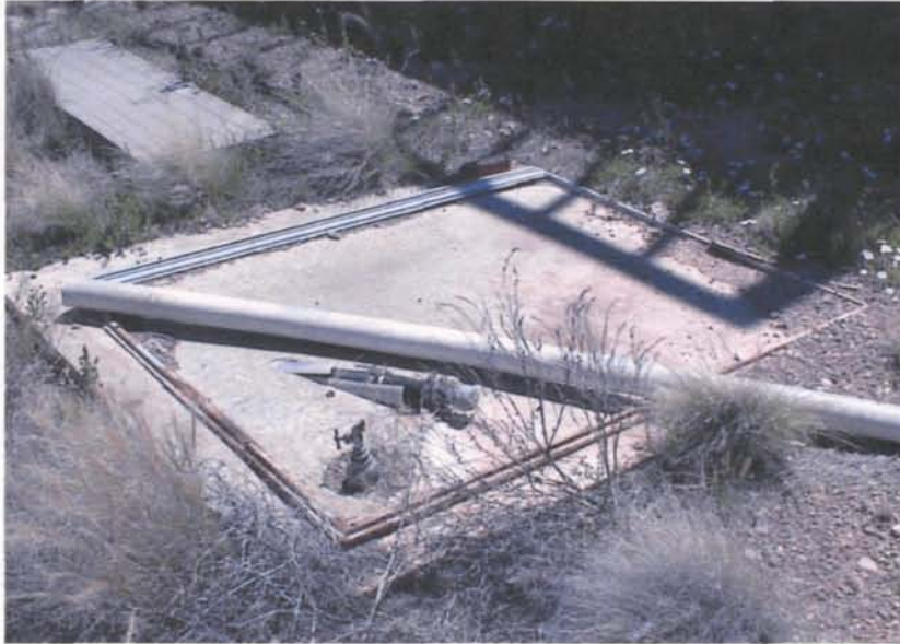
Photo 5 - Supply Well CWSW-1 with exposed two inch black PVC pipe and spigot.
