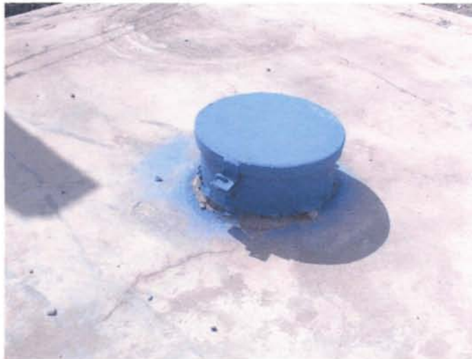
Photo 6 - Supply well CWSW-2 with steel cover and lock installed
