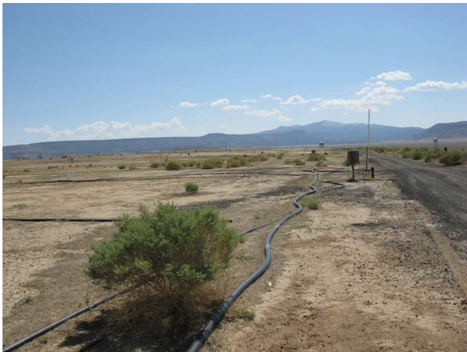
Aboveground piping (looking east)
