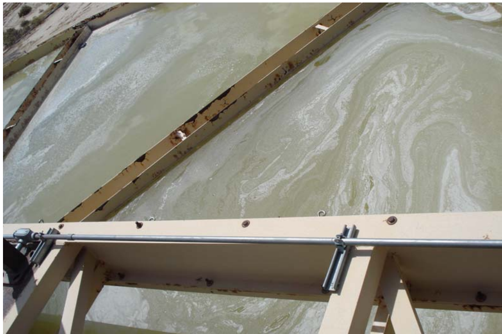
Reactor Clarifier (from top)
