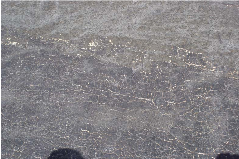
Evaporation Pond #2 liner showing effects of exposure to air and sun
