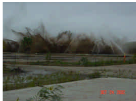
Figure 3: The impact from the stack was absorbed by a bed of sand placed over the target area. A water deluge system kept dust levels down to a minimum.
