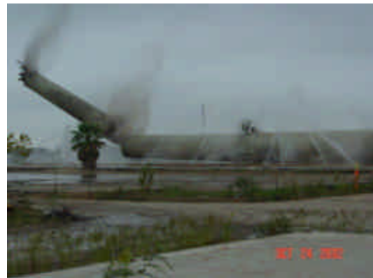
Figure 2: Smokestack falling to earth. The top third broke off the main portion of the stack, as was expected.
