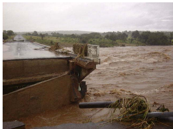
Figure 11.3 Flooding from severe storm events causes millions of dollars in damage to infrastructure every year.
