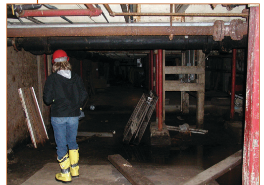
The Pearl Street Mill buildings comprise about 75,000 sq ft. (Photo courtesy of Mr. Christopher Zevitas)
