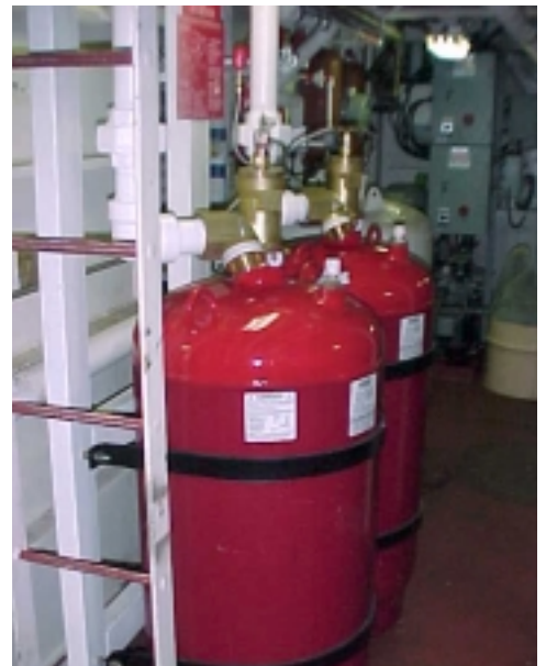
The replacement fire suppression system uses a chemical that has no adverse impacts on the ozone layer.
