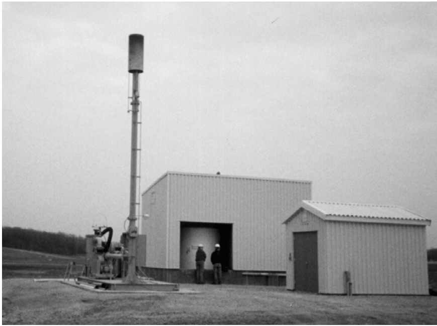
Figure 5-6. Skid-Mounted Open Flare and Blower Station.
