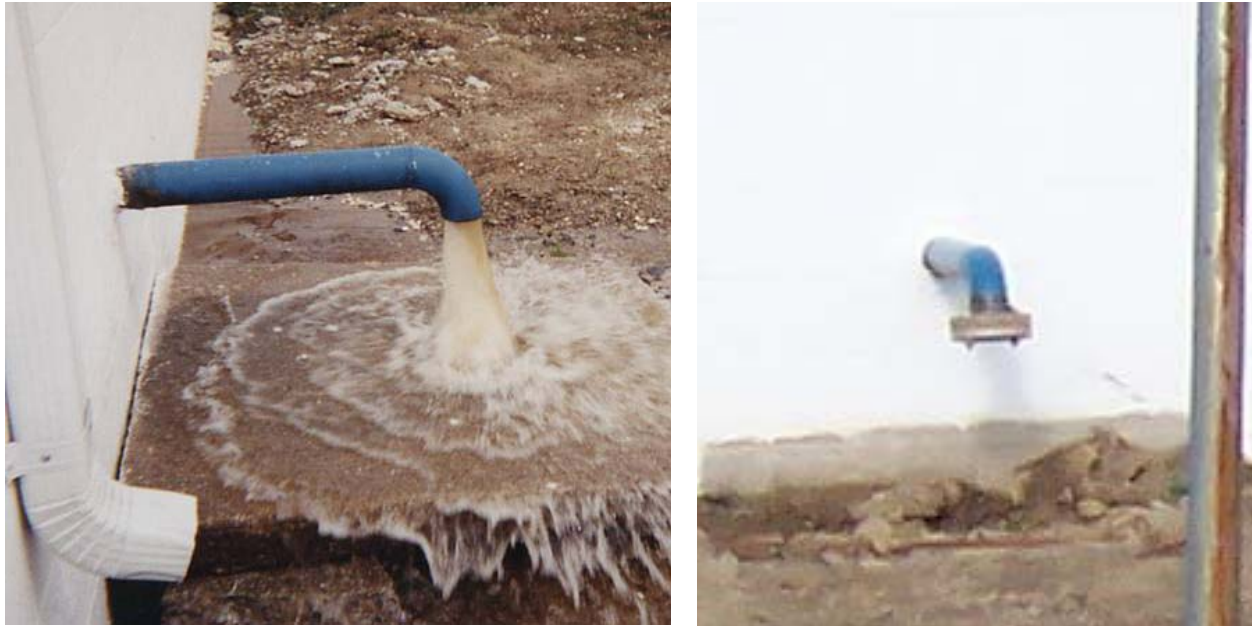
Figure 4-11. Backwash Wastewater Discharge unto the Ground (left) and into an Underground Concrete Vault (right)
