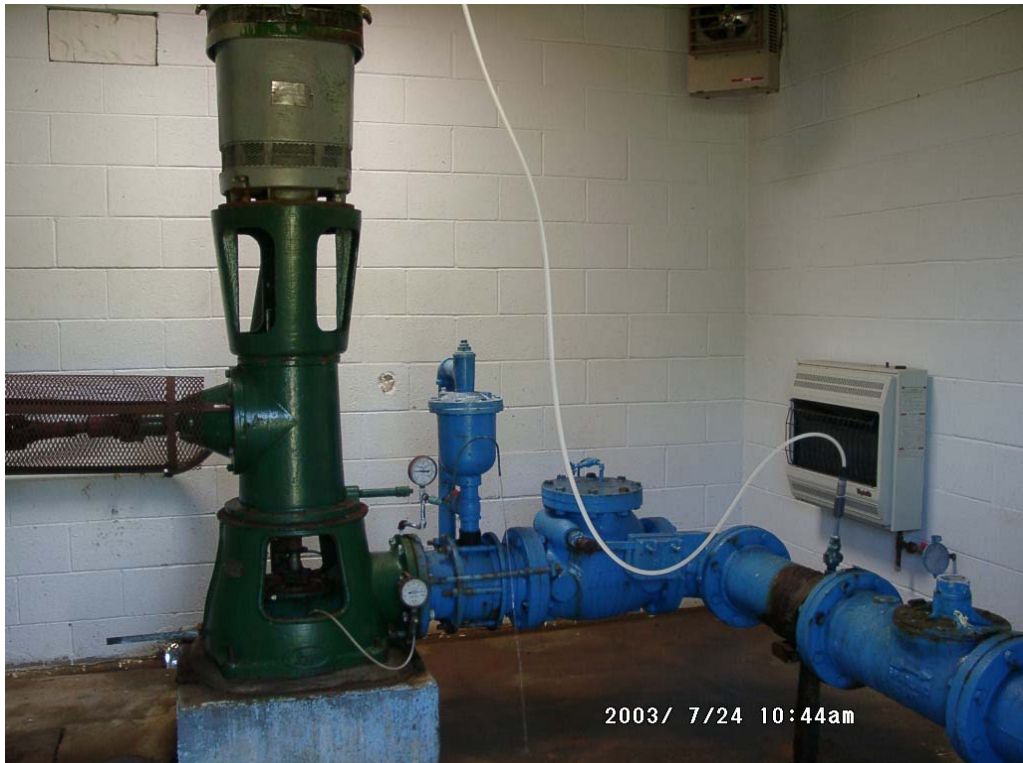
Figure 4-3. Pump Motor, System Piping, and Chlorine Addition Point at Wellhead No. 4
