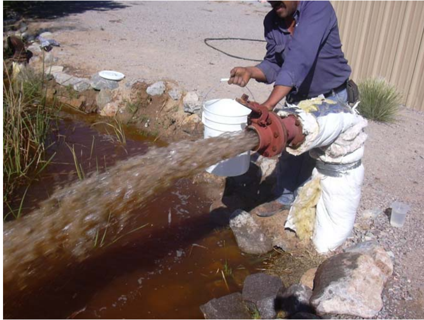
Figure 4-7. Backwash Wastewater Discharge into Pond
