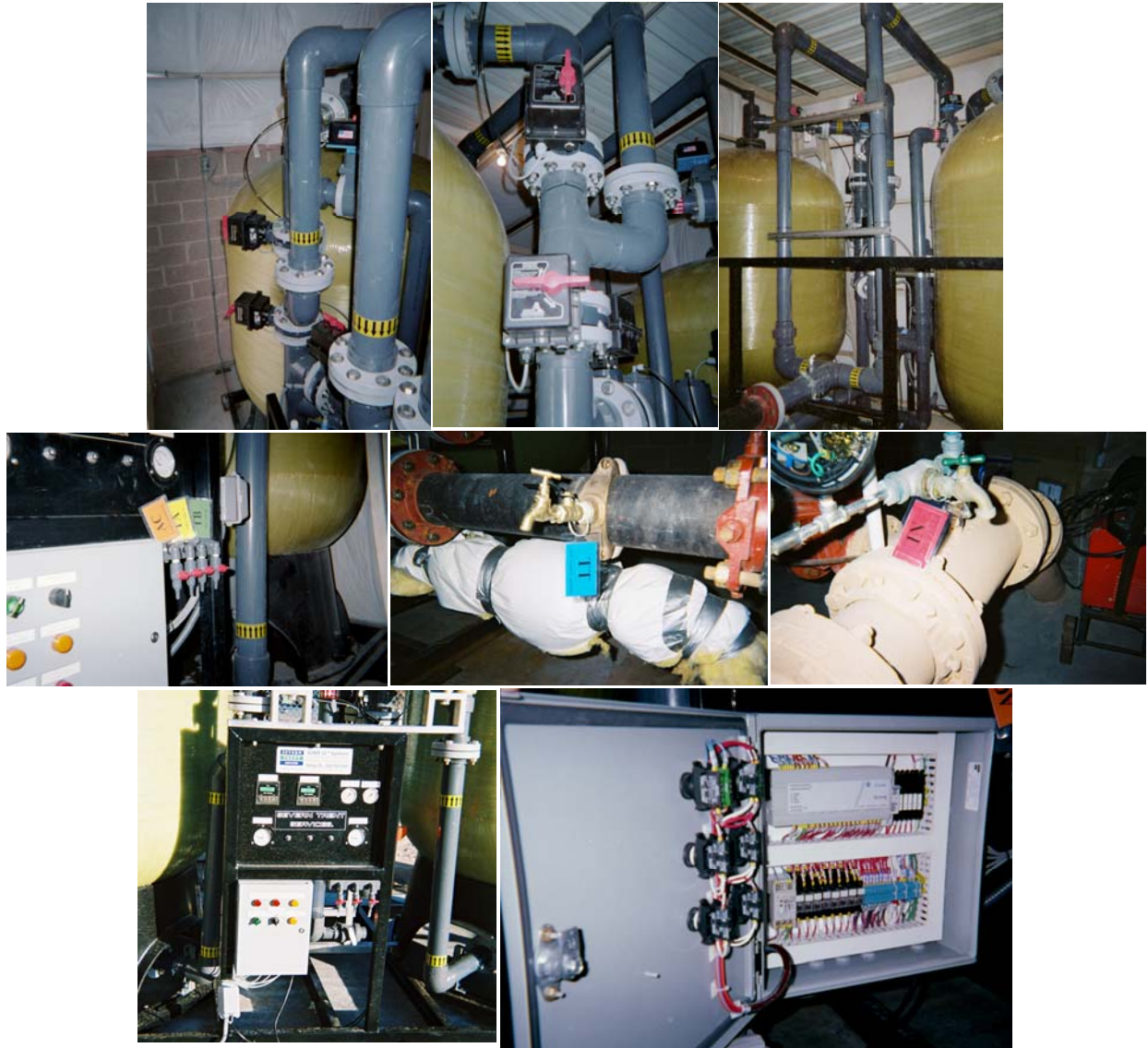
Figure 4-6. Treatment Process Components ( APU-300 System Valve Tree [top left and middle]; Backside of System Piping including Vessel Flow Meter Sensors [top right]; Sampling ports [middle]; and Control Panel [bottom] )
