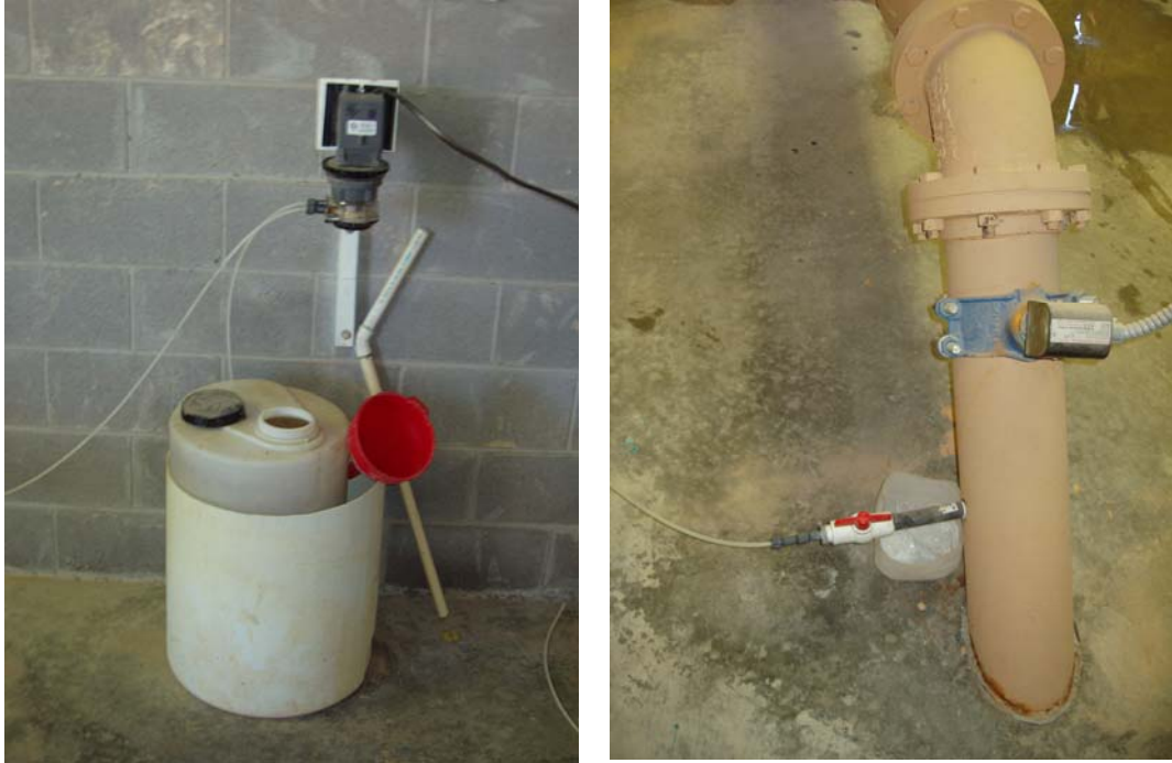
Figure 4-4. Sodium hypochlorite (NaOCl) Injection System at Desert Sands MDWCA Site
