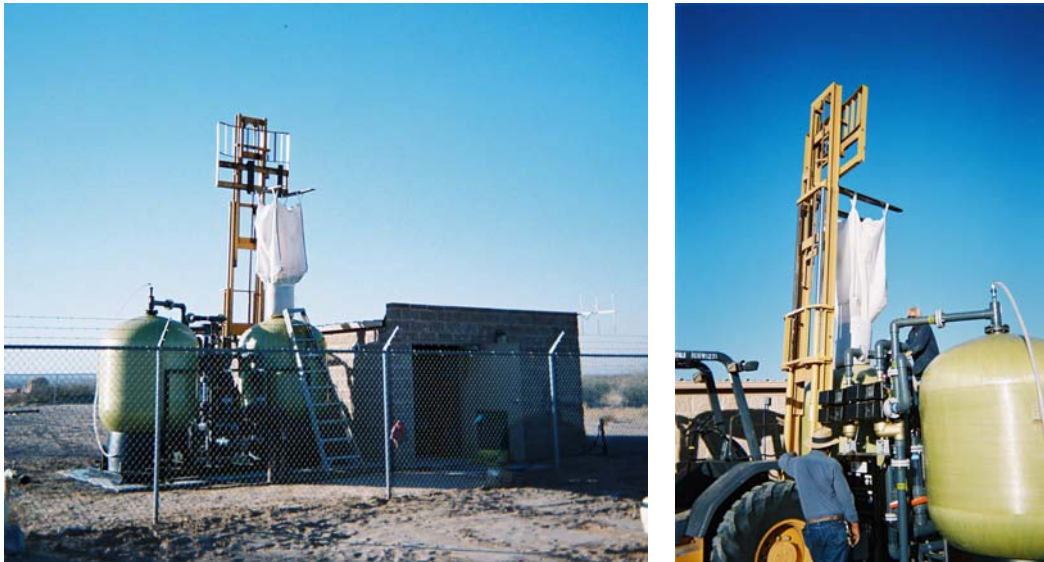
Figure 4-11. Media Loading to Adsorption Vessels
