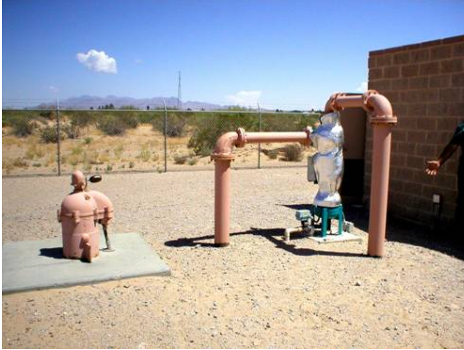
Figure 4-2. Well No. 3 (Left) and In-Line Sand Separator (Center) Adjacent to Pump House (Right) at Desert Sands MDWCA Site
