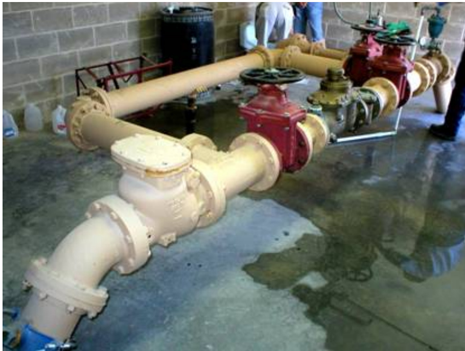
Figure 4-3. Piping Inside Pump House at Desert Sands MDWCA Site
