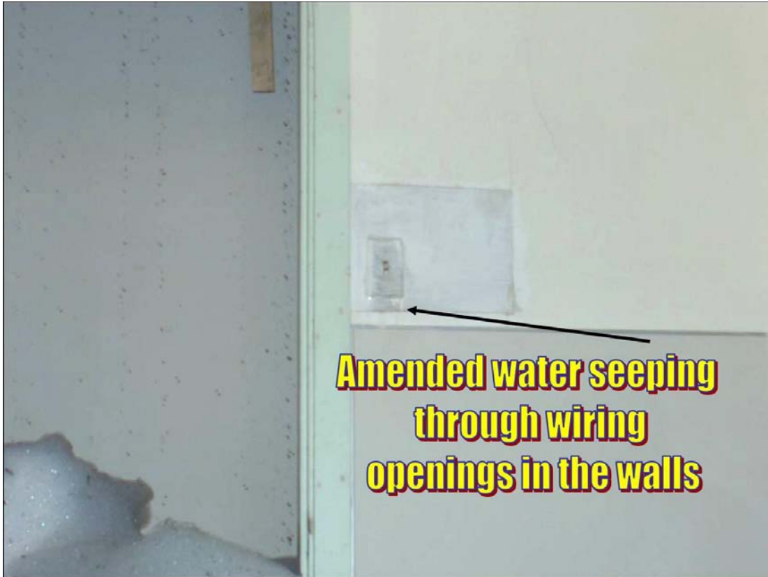
Figure 4-27. Amended Water seeping through wall openings.
