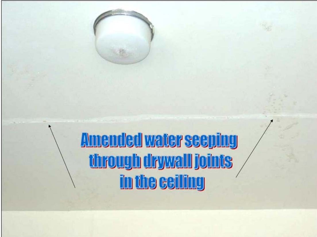
Figure 4-26. Amended Water seeping through ceiling drywall joints.
