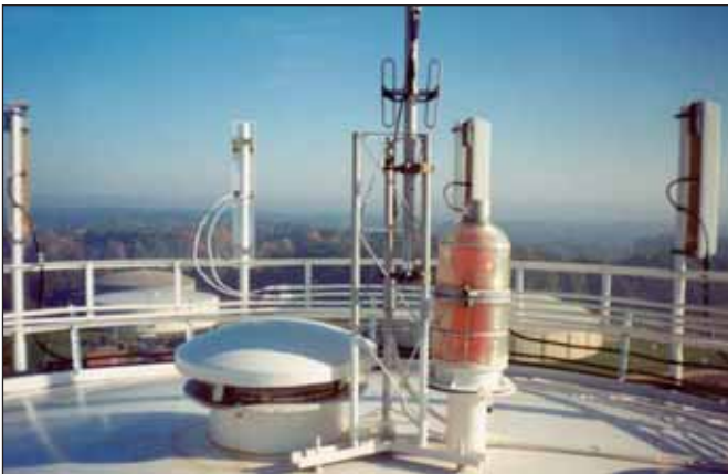
Figure 7.2 A Well-Designed and Constructed Cell Tower Installation
