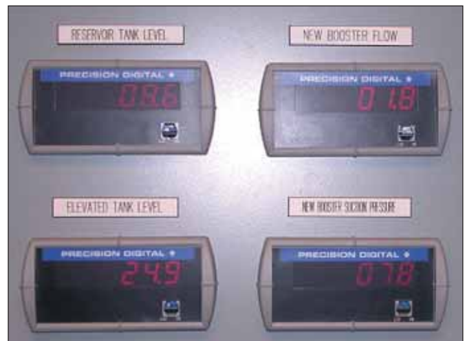
Figure 6.5 Readout meters for flow, water level and pressure from a SCADA system
