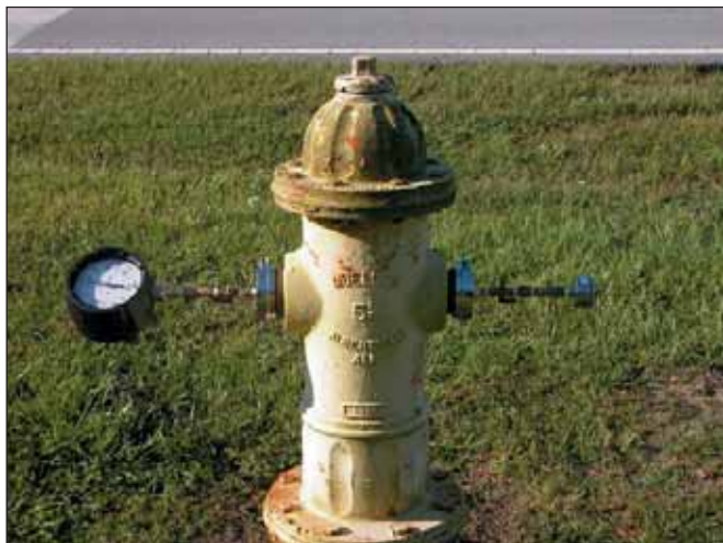
Figure 6.4 Digital and analog pressure meter attached to fire hydrant
