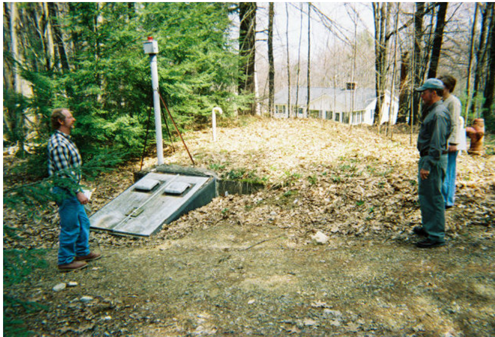
Figure 4-1. Preexisting Underground Treatment and Control Structure
