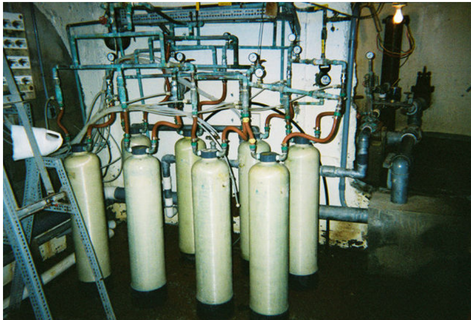
Figure 4-3. Preexisting Activated Alumina System in Underground Treatment and Control Structure
