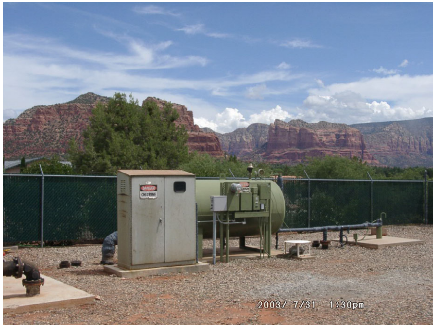
Figure 4-1. Predemonstration Site Conditions (Right to Left: Wellhead, Piping, Hydropneumatic Tank, Electrical Panel, and Chlorine Shed)
