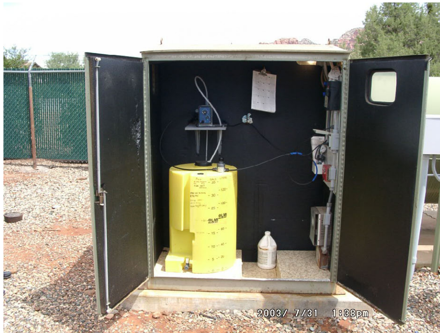
Figure 4-2. Existing Chlorine Injection System
