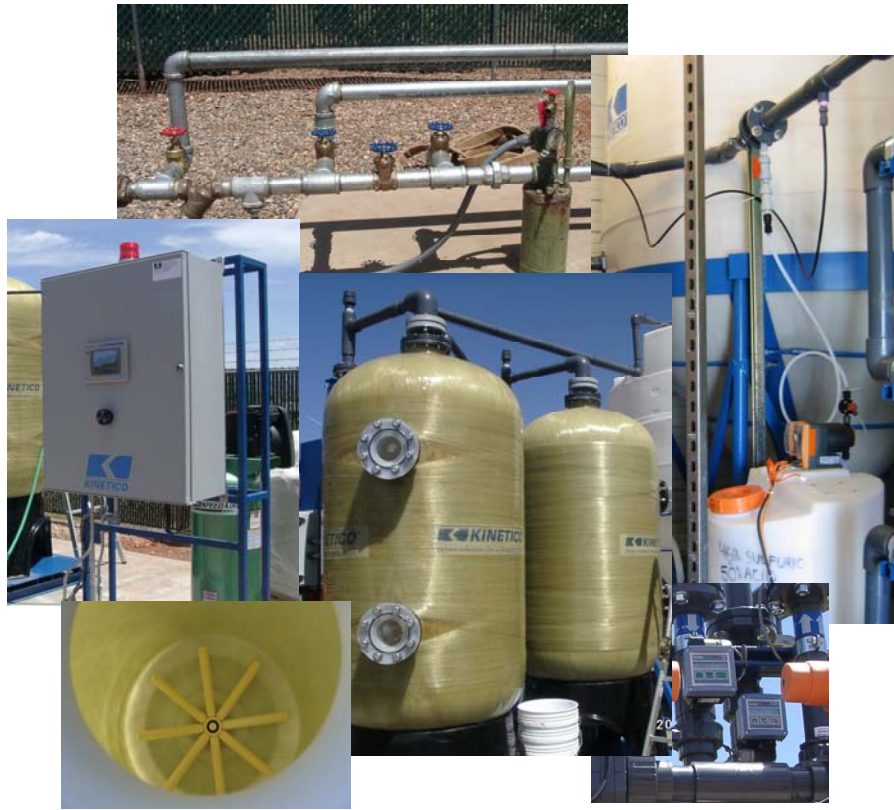
Figure 4-5. Treatment Process Components (Clockwise from Top: POE Well No. 2 and Bypass Piping; Acid Addition Setup; In-Line pH Transmitter; Adsorption Tanks and Lower Distributor; and Main Control Panel)
