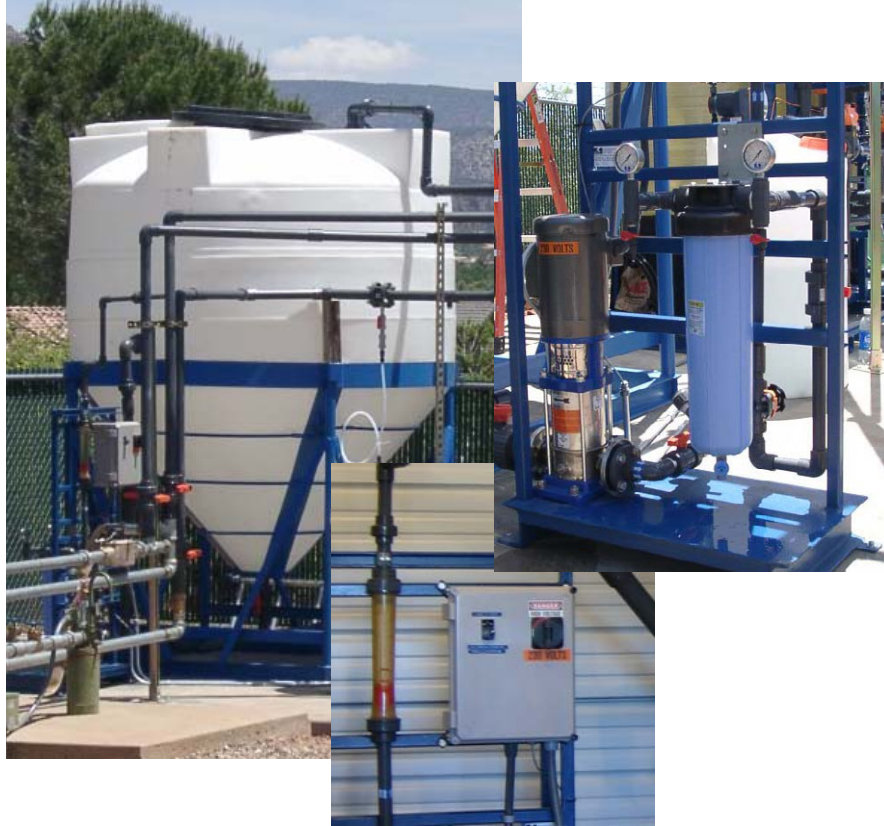
Figure 4-6. Backwash Recycling Process Components (Clockwise from Left: 1,800-gal Holding Tank; Recycle Pump and Bag Filter; and Backwash Flowrate Indicator and Pump Box)
