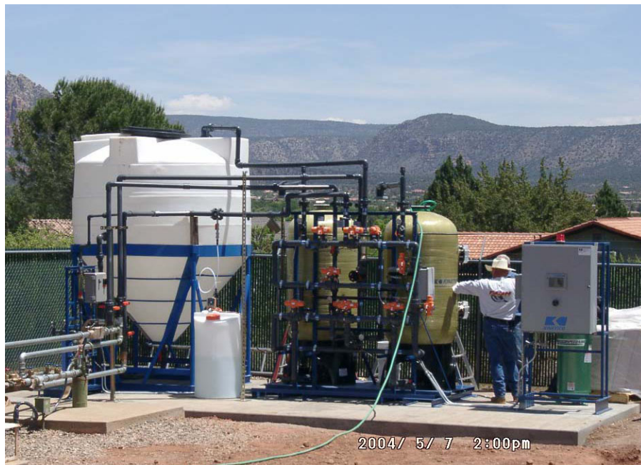
Figure 4-4. Kinetico's FA-236-AS Treatment System on Concrete Pad
