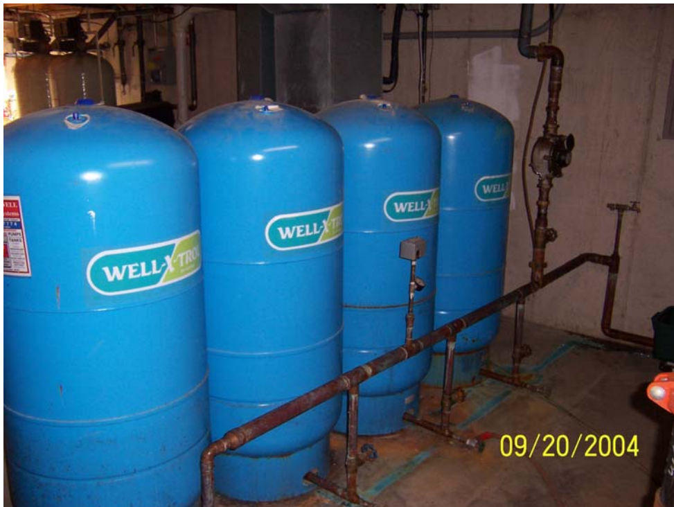
Figure 4-2. Preexisting Well Piping and Pressure Tanks
