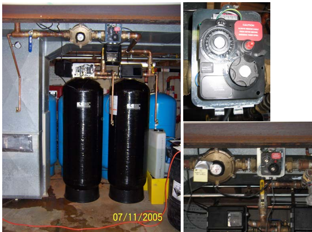
Figure 4-7. Macrolite® Pressure Filtration System (Clockwise from Left: Pressure Filters; Backwash Timer Assembly; Totalizer on Treated Waterline)
