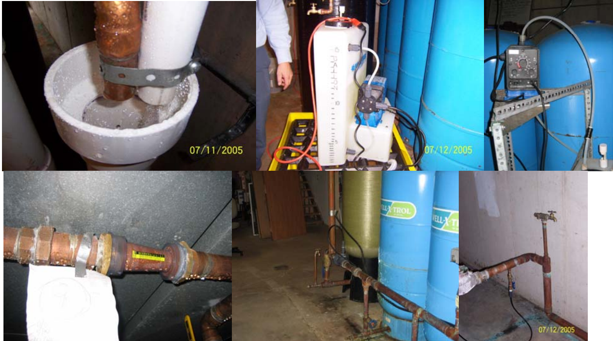
Figure 4-9. Photographs of System Components
