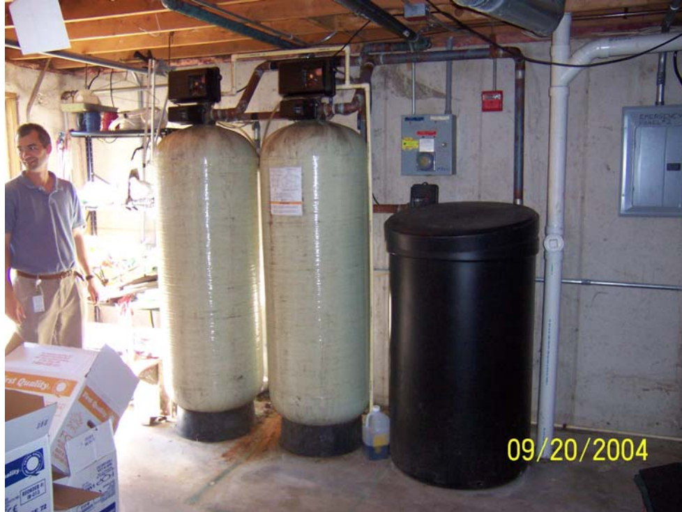
Figure 4-3. Preexisting Softener System
