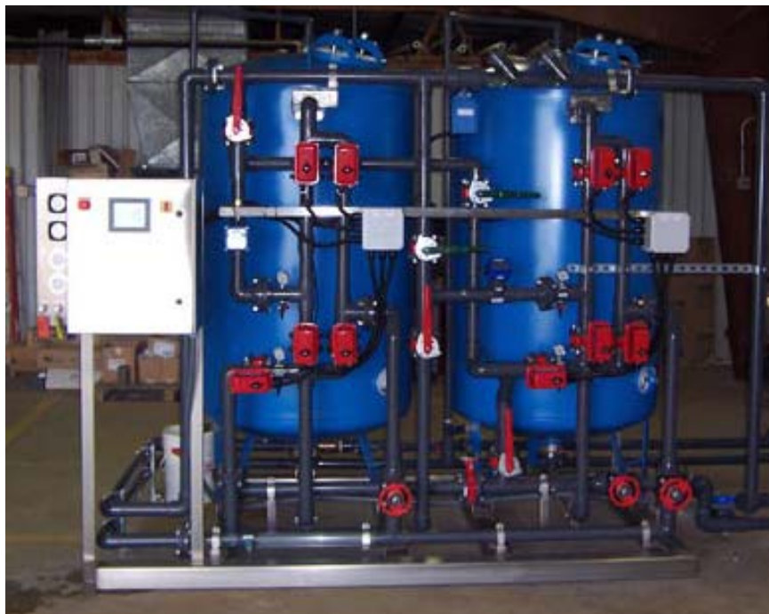
Figure 4-9. Adsorption System Valve Tree and Piping Configuration
