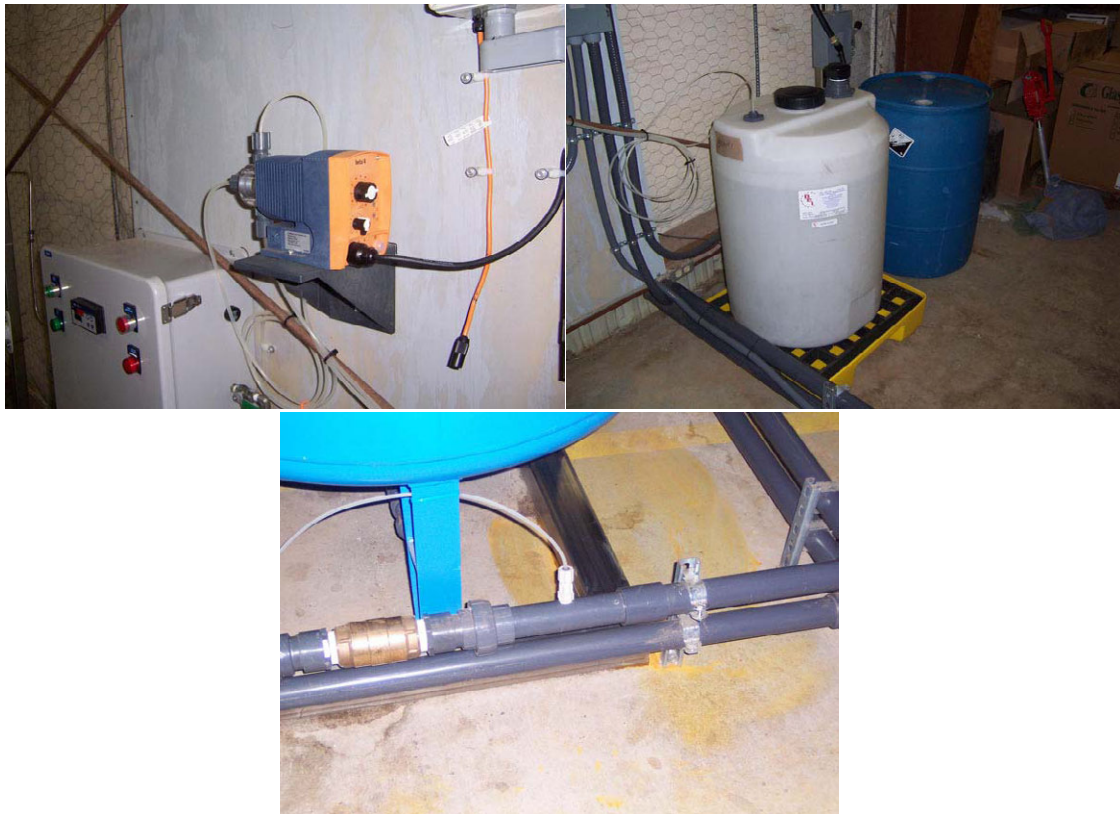
Figure 4-8. Chlorination Feed System (Clockwise from Top Left: Chlorine Metering Pump; HDPE Chemical Feed Tank with Secondary Containment; Chlorine Injection Port)
