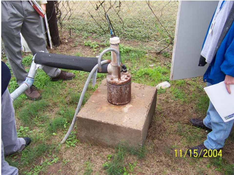
Figure 4-2. Wellhead at Webb CISD
