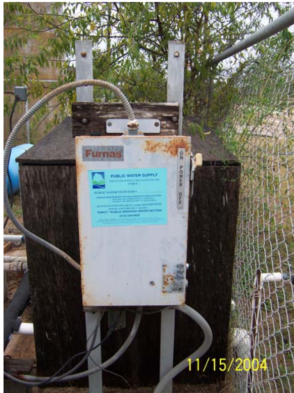
Figure 4-3. Existing Chlorine Addition System
