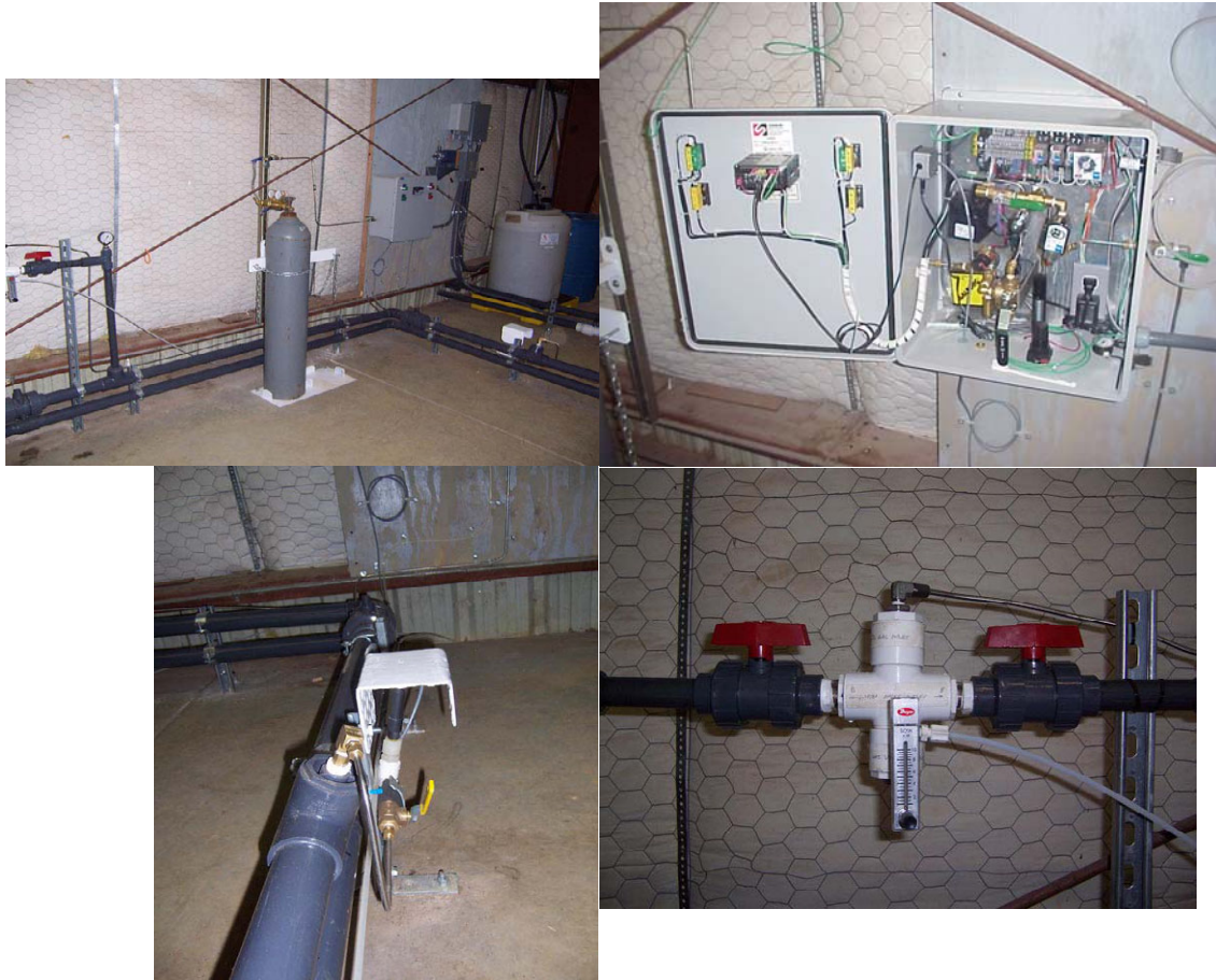
Figure 4-7. Carbon Dioxide Gas Flow Control System for pH Adjustment (Clockwise from Top Left: Liquid CO 2 Supply Assembly; Automatic pH Control Panel; CO 2 Membrane Module; Port for pH Probe)
