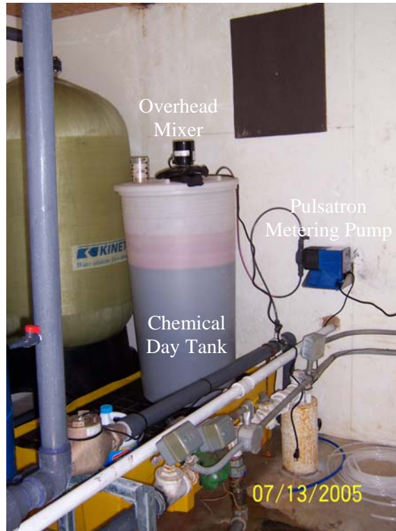
Figure 4-5. KMnO 4 Feed System
