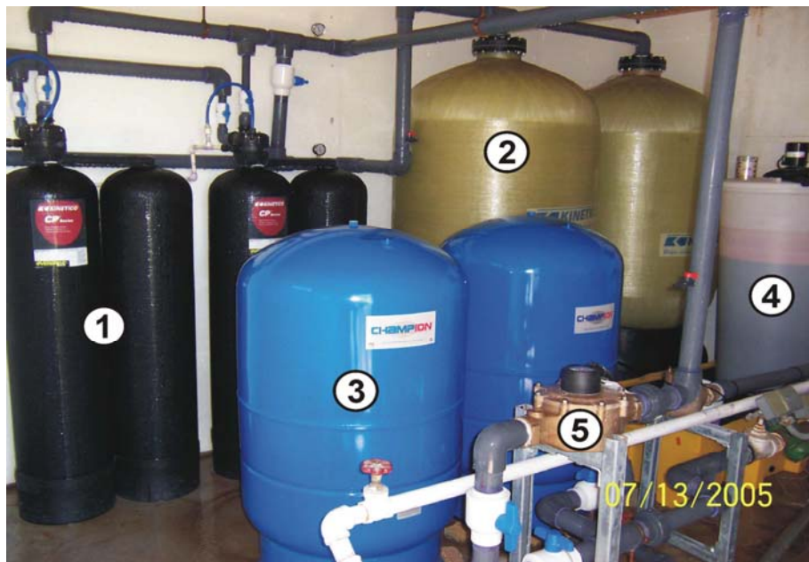
Figure 4-4. Photograph of Macrolite® Pressure Filtration System (1. Duplex Units, 2. Contact Tanks, 3. Pressure Tanks, 4. Chemical Day Tank, and 5. Totalizer on Raw Water Line)
