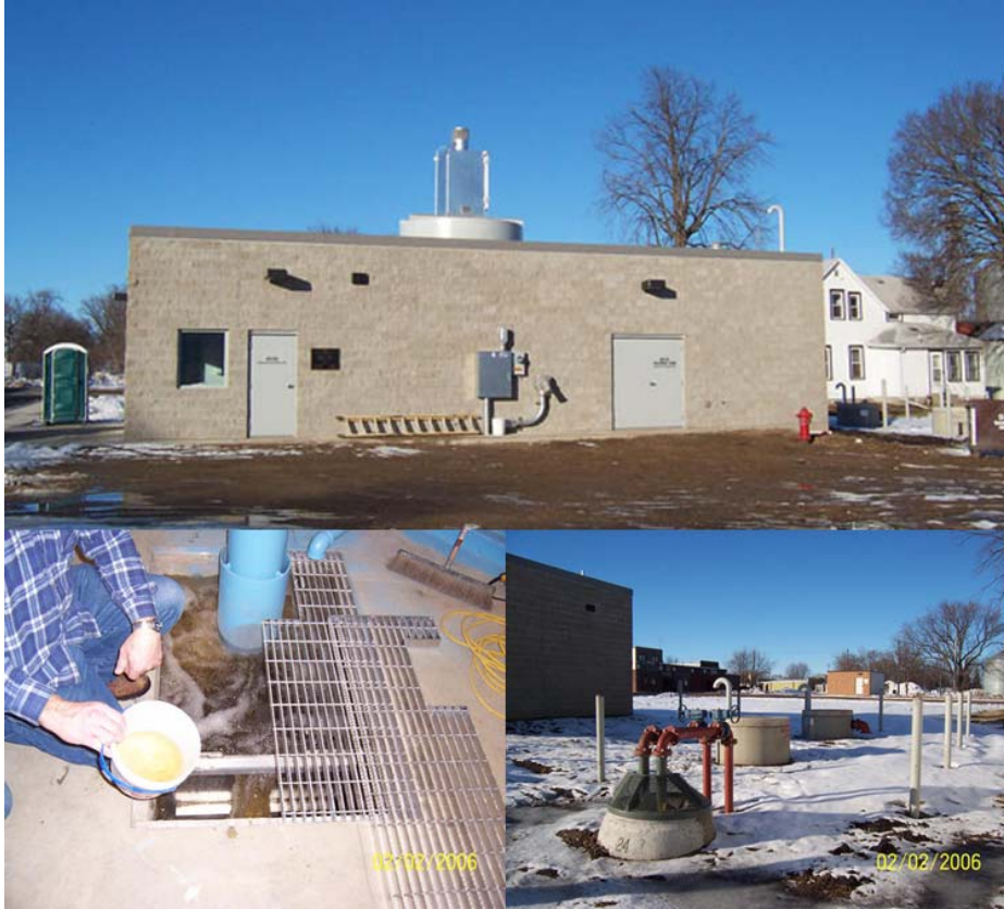
Figure 4-10. Building with AERALATER® Tower (top), Backwash Sump (bottom left), and Backwash Water Holding Tanks (bottom right) at Stewart, MN
