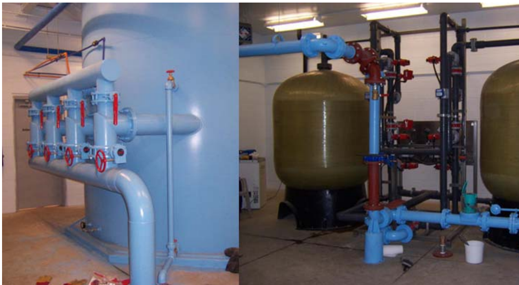
Figure 4-7. AERALATER ® (left) and APU-300 Systems (right) at Stewart, MN
