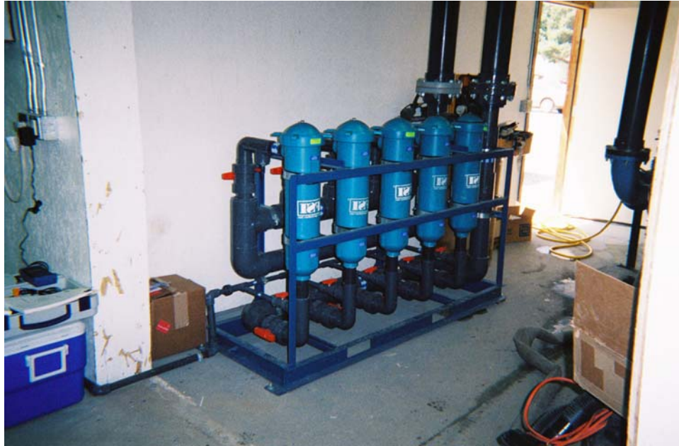
Figure 4-4. Photograph of Bank of Five Bag Filters
