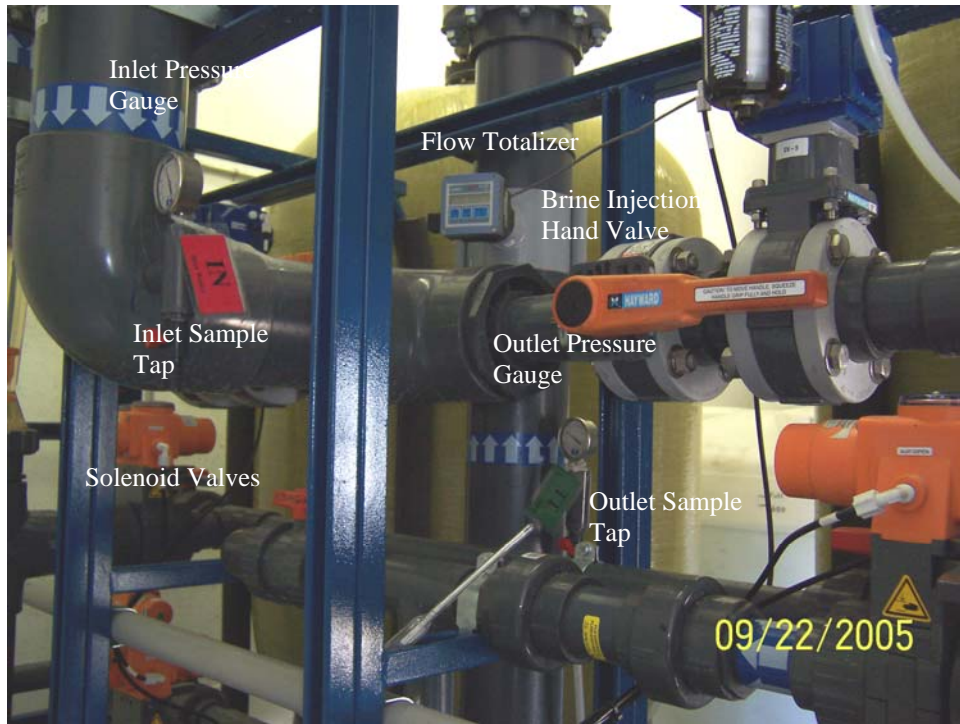
Figure 4-6. Sampling Taps, Pressure Gauges, and Valves
