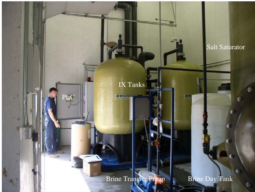
Figure 4-5. Photograph of IX-248-As/N System at Fruitland, ID
