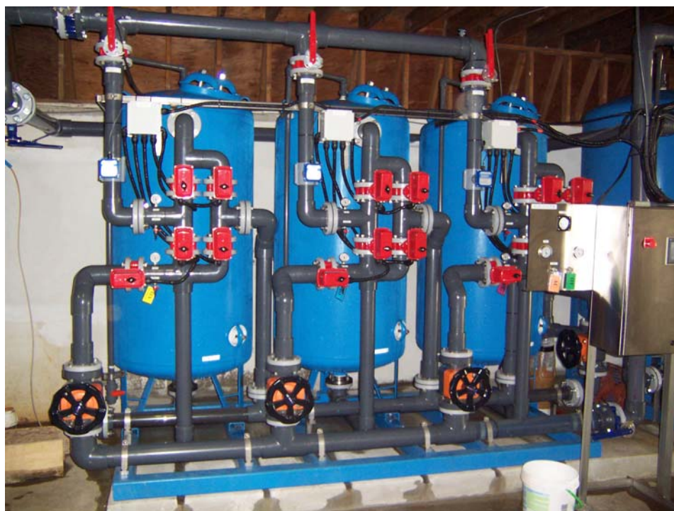
Figure 4-7. AD-26 Treatment System
