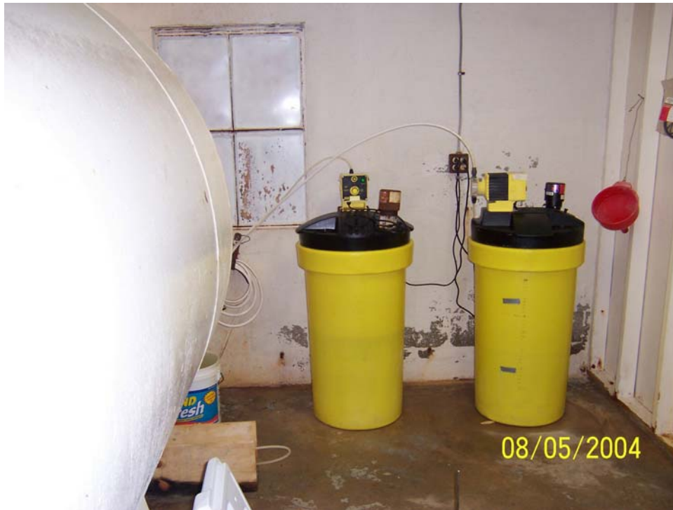
Figure 4-2. Pre-Existing Chlorine and Polyphosphate Addition Systems
