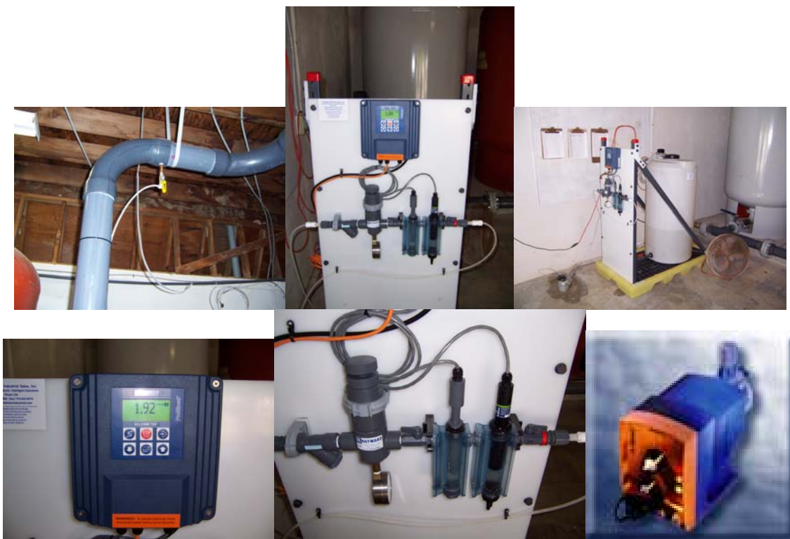
Figure 4-6. Chlorine Injection System
