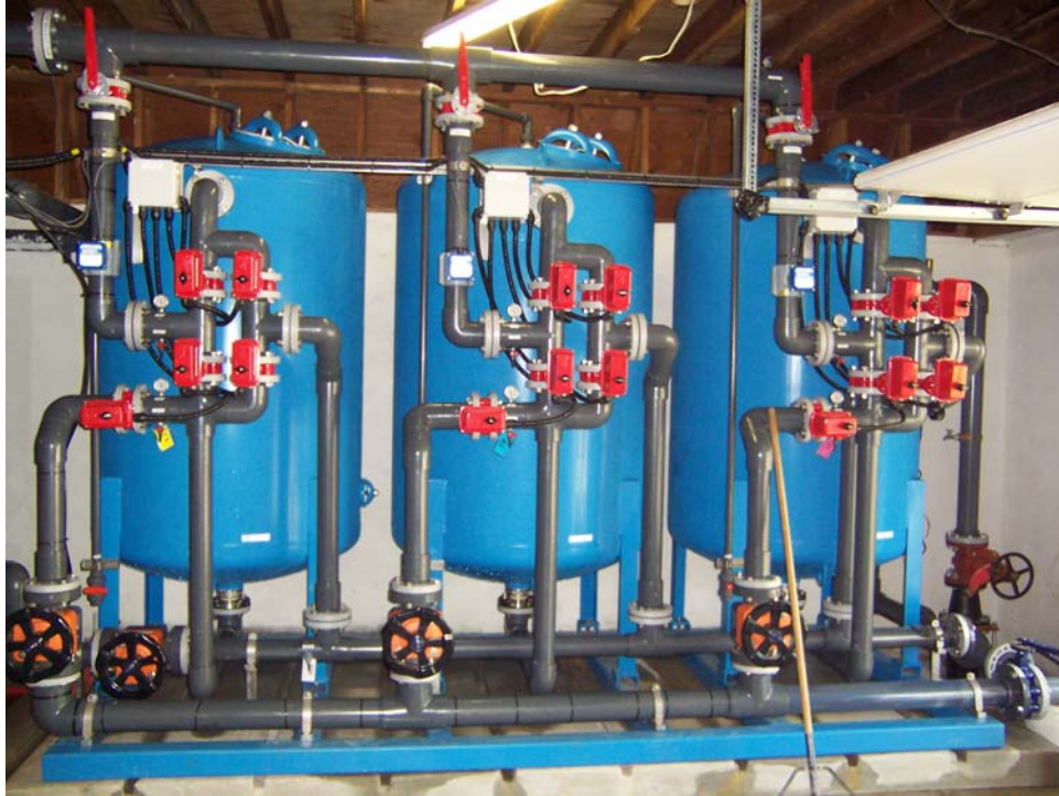
Figure 4-9. AD-33 Treatment System
