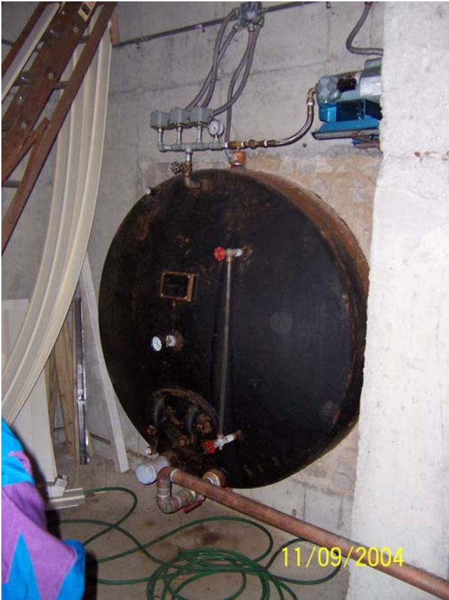
Figure 4-5. 2,000-gal Hydro-pneumatic Pressure Tank
