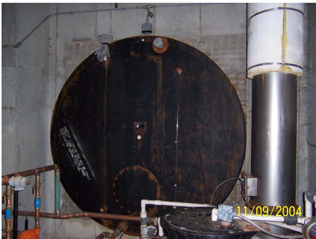
Figure 4-3. 10,000-gal Storage Tank
