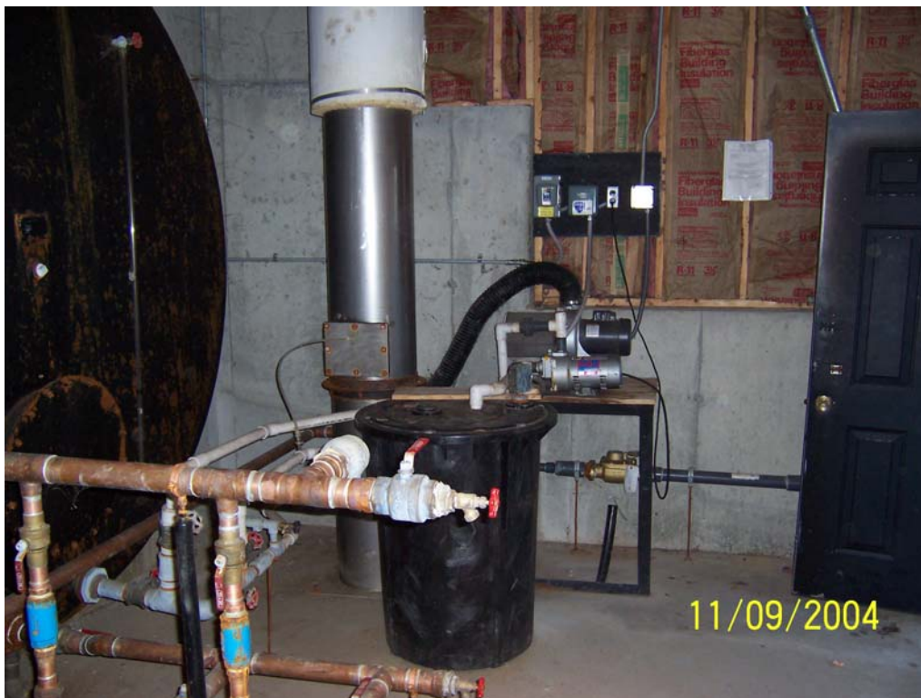
Figure 4-2. Aeration System for Radon Treatment
