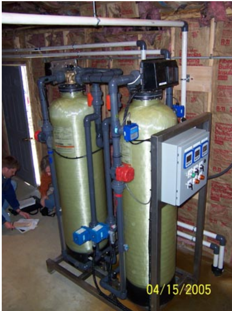
Figure 4-8. APU-GOFF-LL Treatment System
