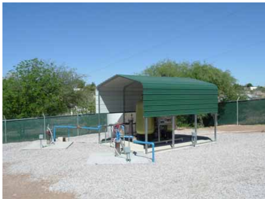
Figure 4-6. Sun Shed Structure over the Treatment System
