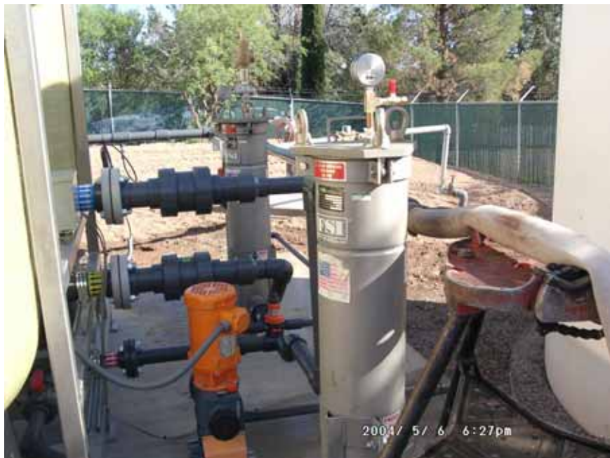
Figure 4-5. Photograph of the Backwash Recycle System
