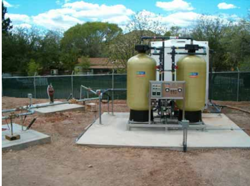
Figure 4-4. Photograph of the APU-100 System
