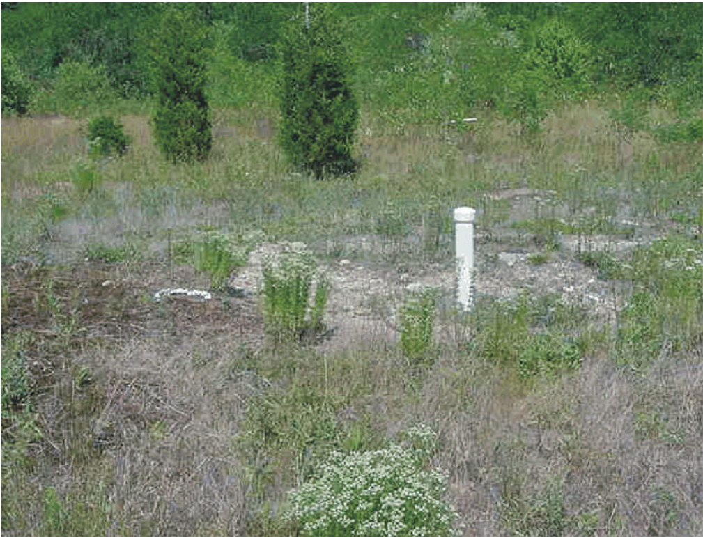
Passive Vent at Grid 80
