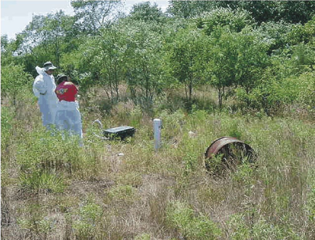
Passive Vent at Grid 131
