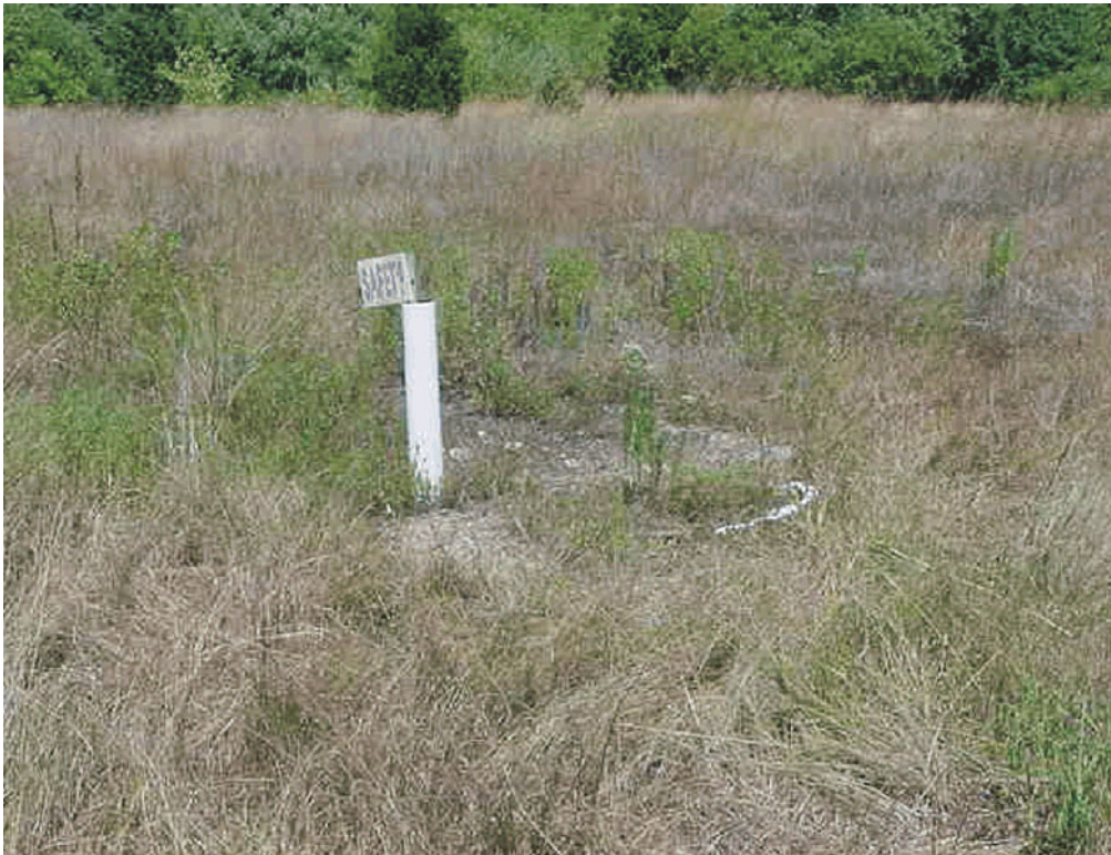
Passive Vent at Grid 140
