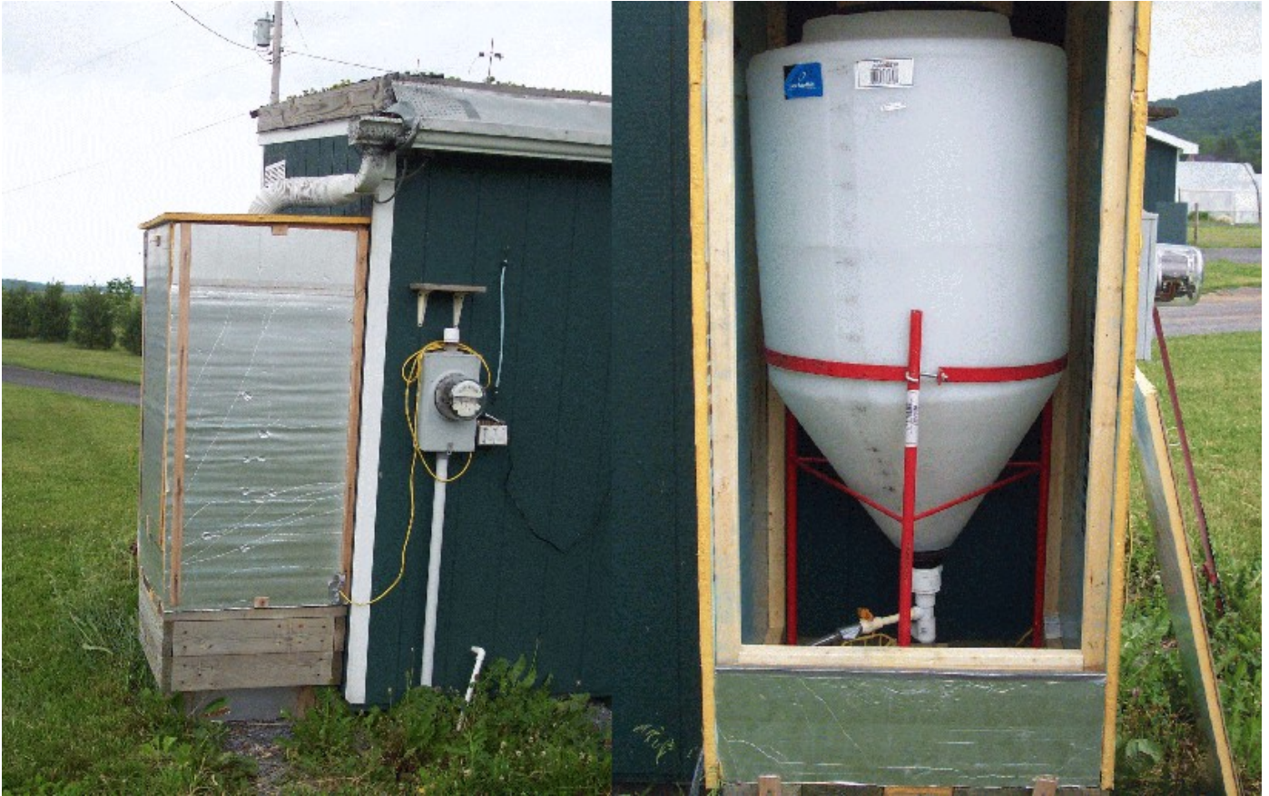
Figure A-6. Barrel enclosure with 1 in. (2.5 cm) insulation with a small heater inside to prevent the barrels from freezing (closed view on left and open view on right)
