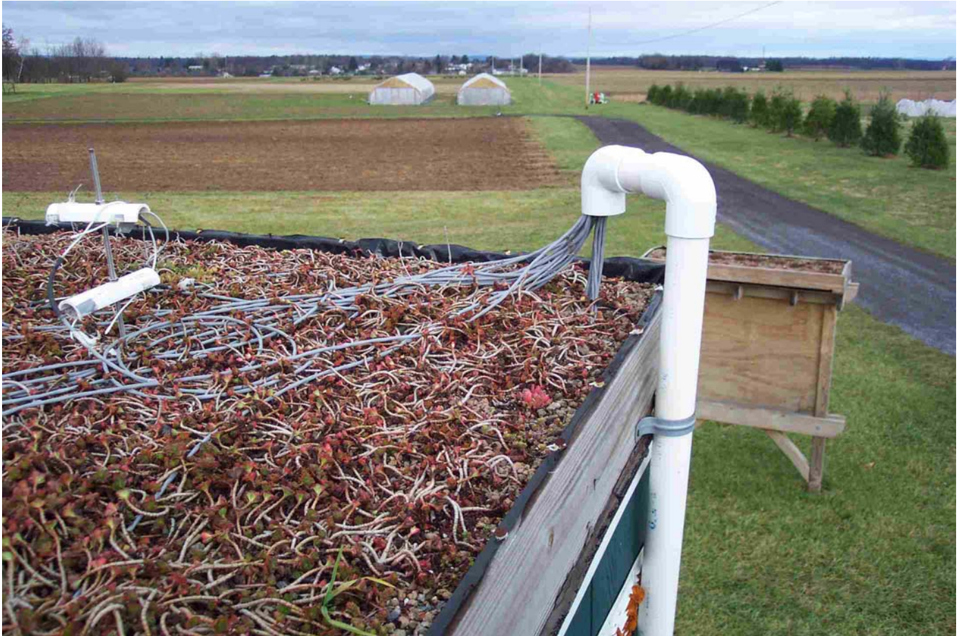
Figure A-3. Green roof with monitoring equipment, November 2003
