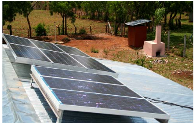
Solar energy powers the El Sol Health Center in Carazo, Nicaragua
