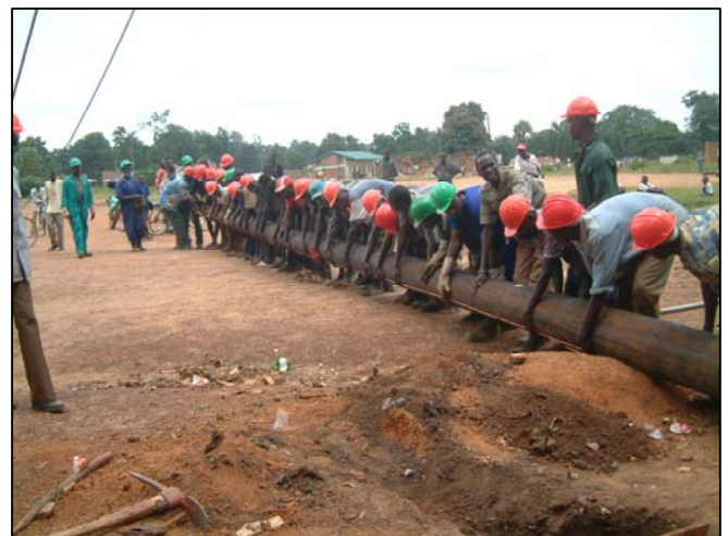
Yei residents raise a pole in the construction of their electricity system
