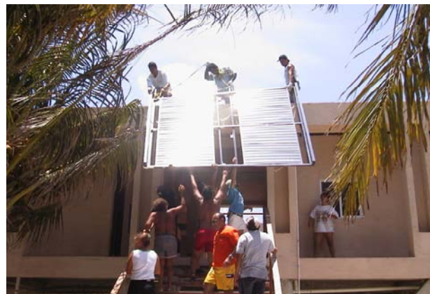
Teamwork by Field Station stakeholders is demonstrated as solar collectors are lifted to the roof for installation.
