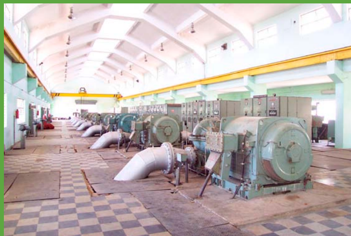
Water pumping station at the Bangalore Water Supply and Sewerage Board in Karnataka, India.
