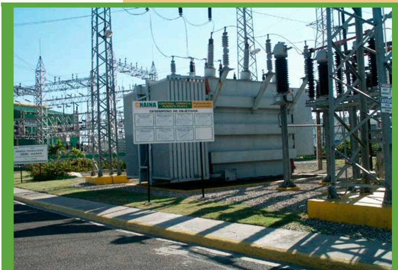
Power plant in Haina, the Dominican Republic.
