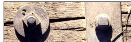
Figure 3. Original Conrail System using a Hook Bolt and a Washer Nut.
