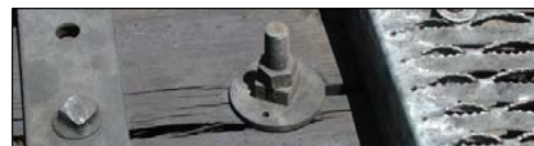
Figure 4. Double Nut and Washer Nut with Nail Hole Fasteners under a Moveable Bridge Joint.
