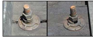
Figure 6a (left). Locking Nut, Spring Lock, and Washer. Figure 6b (right). Broken Spring Lock on Hook Bolt Hook Bolts with Lock Nuts, Spring Washers, and Locking Clips.
