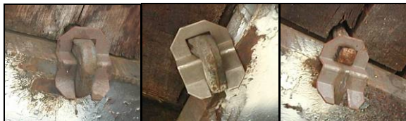
Figure 5. Hook Bolt Fasteners with Locking Clips, (5a) Typical, (5b) Turned Hook Bolt, and (5c) Broken Hook Bolt.
